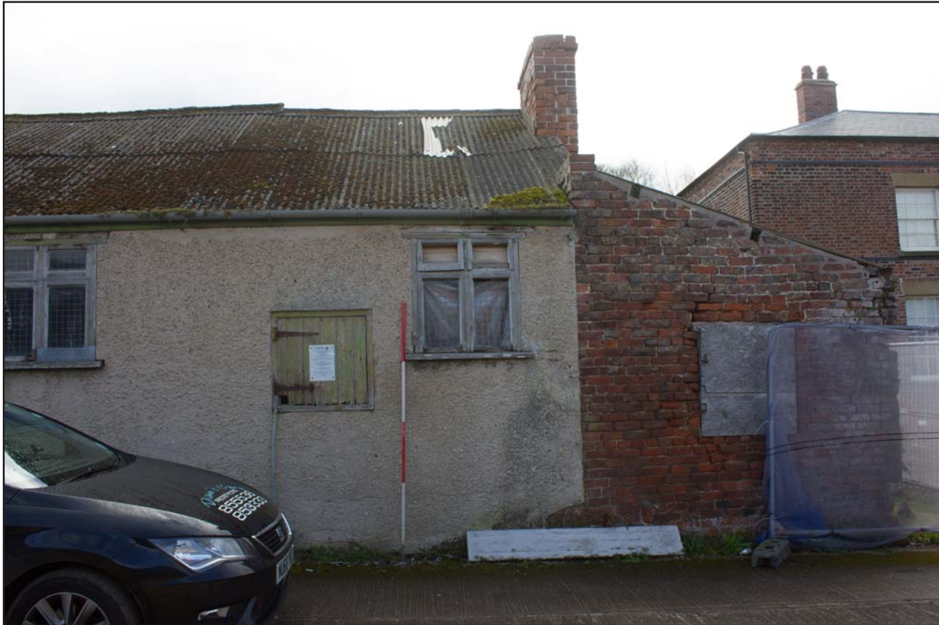
Plate 08: External northwest (right) elevation shot of Dairy Outbuilding at Bryn Cwnin Farm, Pentre Lane, Rhuddlan, Rhyl, Denbighshire - from the northwest - 2.00m scale
