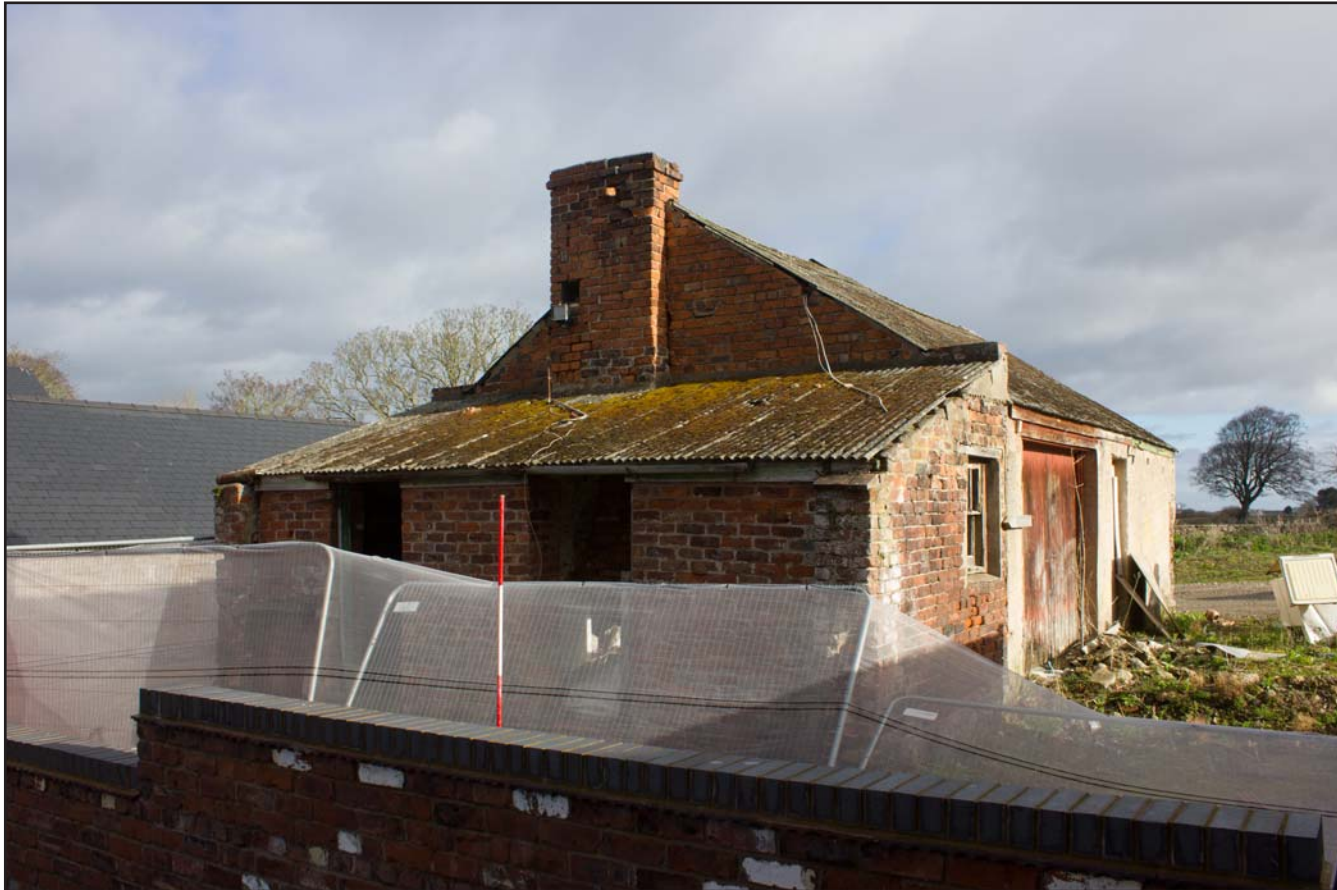
Plate 05: Oblique shot of southeast and southwest elevations of Dairy Outbuilding at Bryn Cwnin Farm, Pentre Lane, Rhuddlan, Rhyl, Denbighshire - from the south - 2.00m scale
