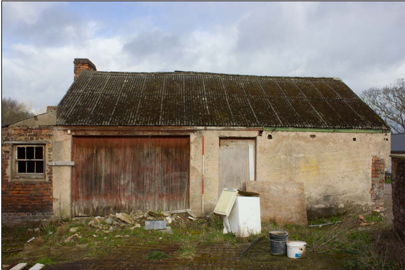
Plate 03: External southeast (right) elevation shot of Dairy Outbuilding at Bryn Cwnin Farm, Pentre Lane, Rhuddlan, Rhyl, Denbighshire - from the southeast - 2.00m scale
