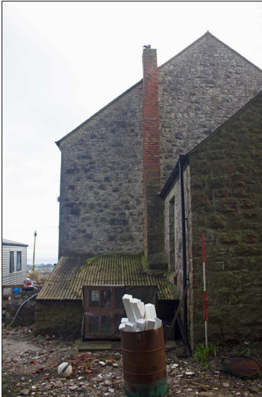
Plate 09: Shot showing southern elevation (left) of Capel Carmel, Carmel Road, Carmel, Flintshire - from the south - 2.00m scale
