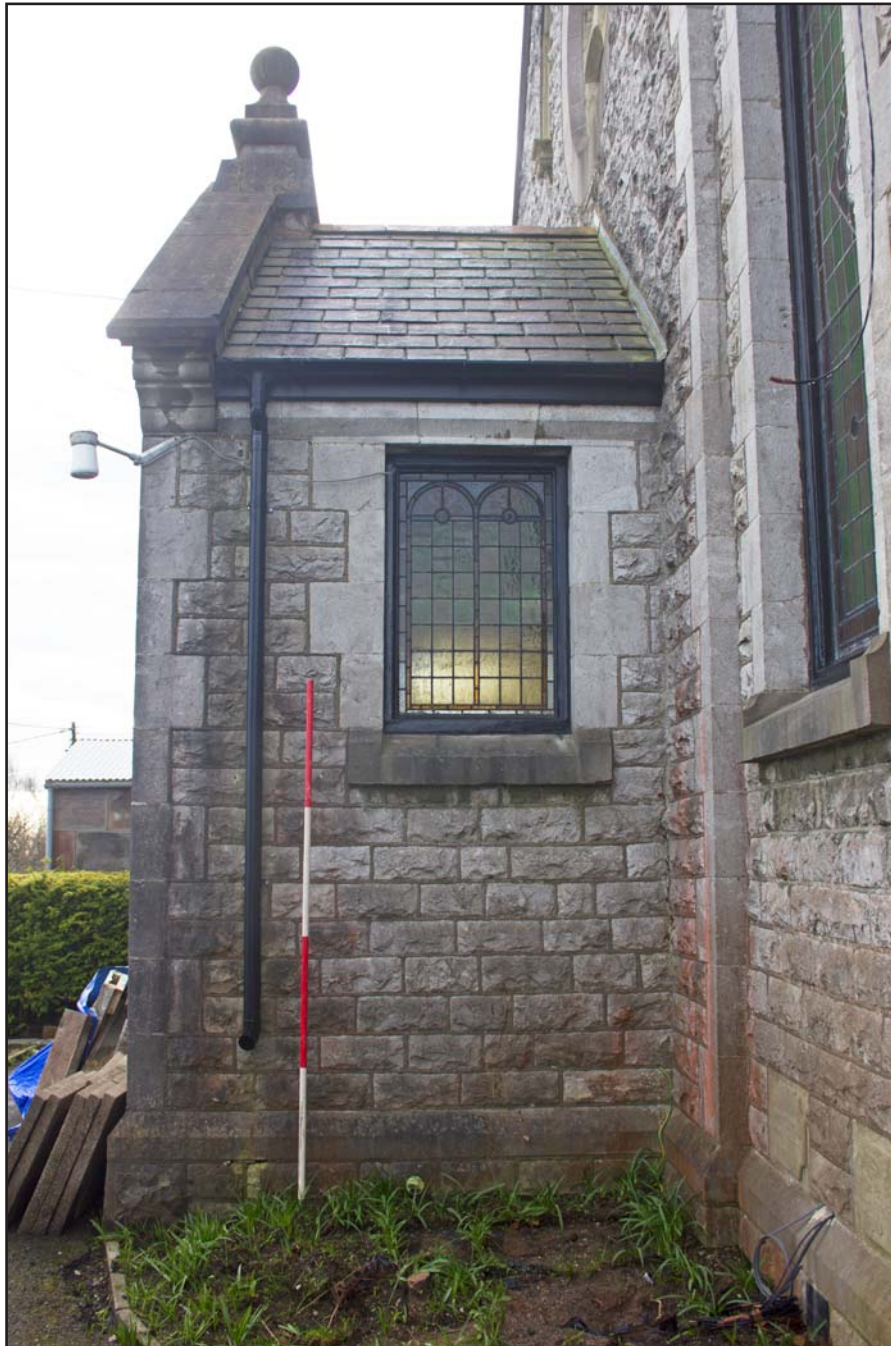
Plate 19: Shot of porch window of Capel Carmel, Carmel Road, Carmel, Flintshire - from the east- 2.00m
