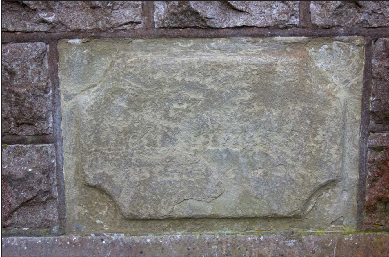
Plate 22: Commemorative stone (illegible) on lower portion (right side) of northern elevation of Capel Carmel, Carmel Road, Carmel, Flintshire - from the north - no scale
