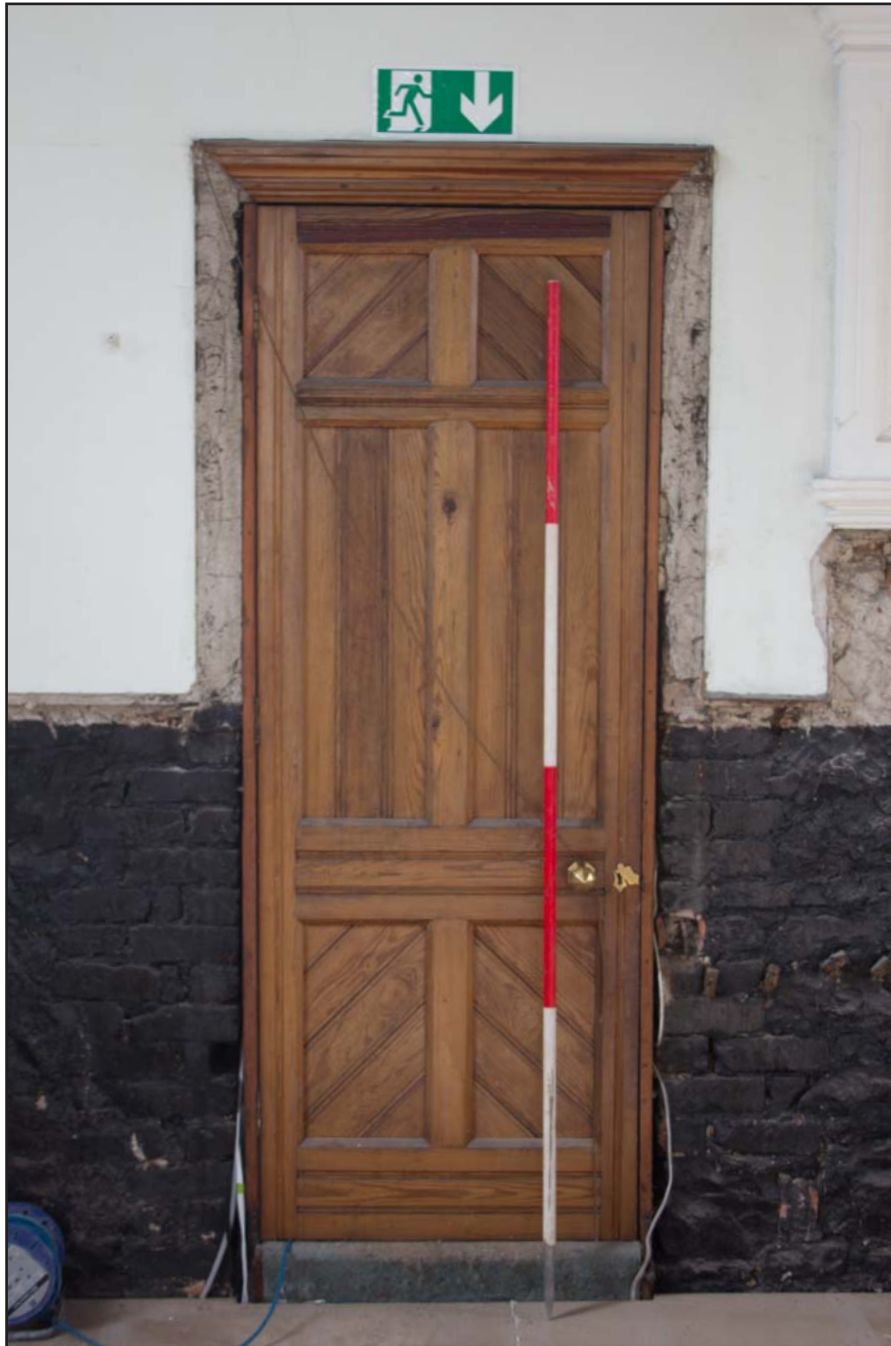
Plate 51: The Vestry door, internal shot, at Capel Carmel, Carmel Road, Carmel, Flintshire - from the north - 2.00m scale
