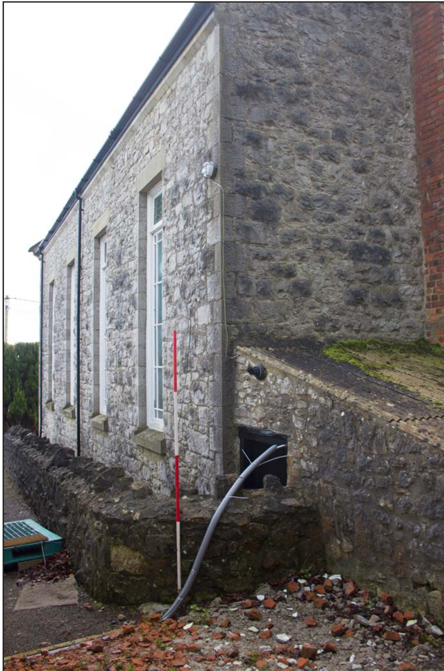
Plate 07: Shot showing western elevation (oblique) of Capel Carmel, Carmel Road, Carmel, Flintshire - from the southwest - 2.00m scale
