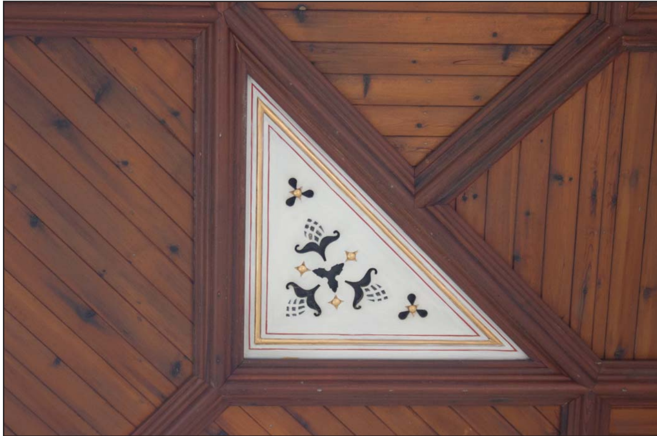
Plate 35: Triangular ventilation plate (example), internal shot, at Capel Carmel, Carmel Road, Carmel, Flintshire - no scale
