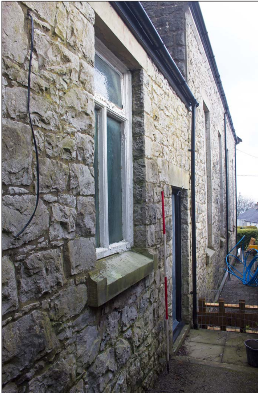
Plate 11: Shot showing eastern elevation (oblique) of Capel Carmel, Carmel Road, Carmel, Flintshire - from the southeast - 2.00m scale
