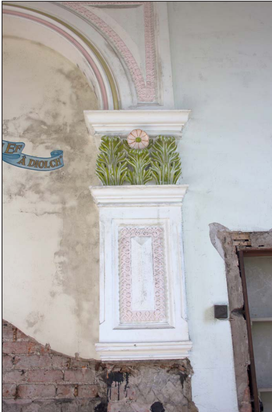
Plate 50: Decorative timber and plaster pillar (left), internal shot, at Capel Carmel, Carmel Road, Carmel, Flintshire - from the north - 2.00m
