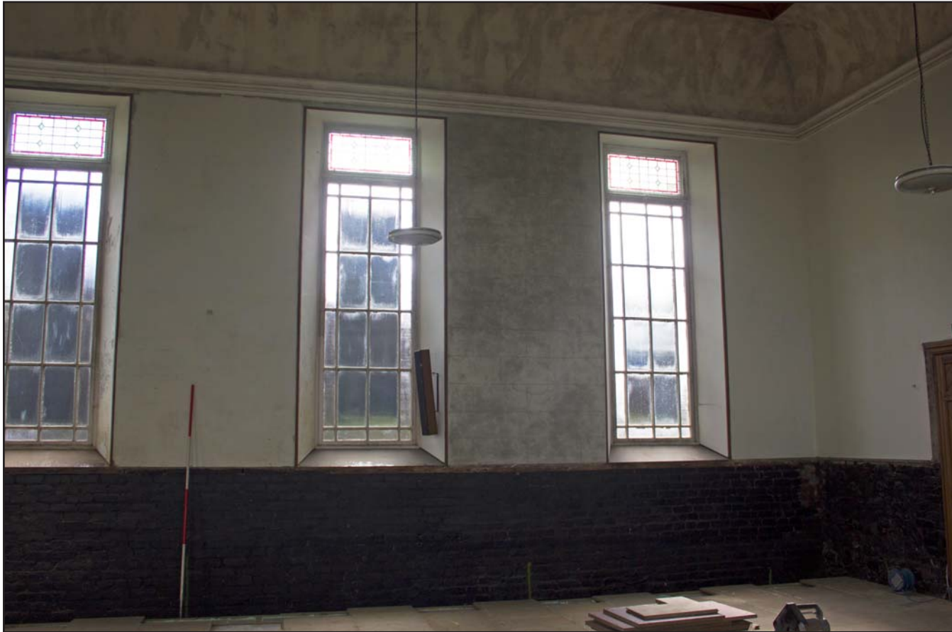
Plate 46: Eastern wall of Chapel (right), internal shot, at Capel Carmel, Carmel Road, Carmel, Flintshire - from the west - 2.00m
