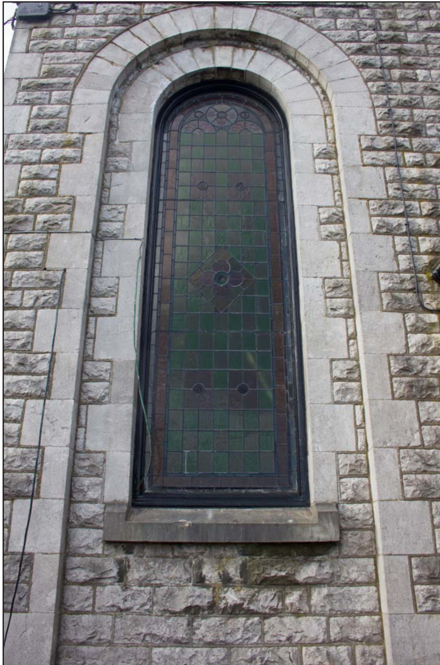
Plate 14: Shot of northern (left) gable window of Capel Carmel, Carmel Road, Carmel, Flintshire - from the north - no scale
