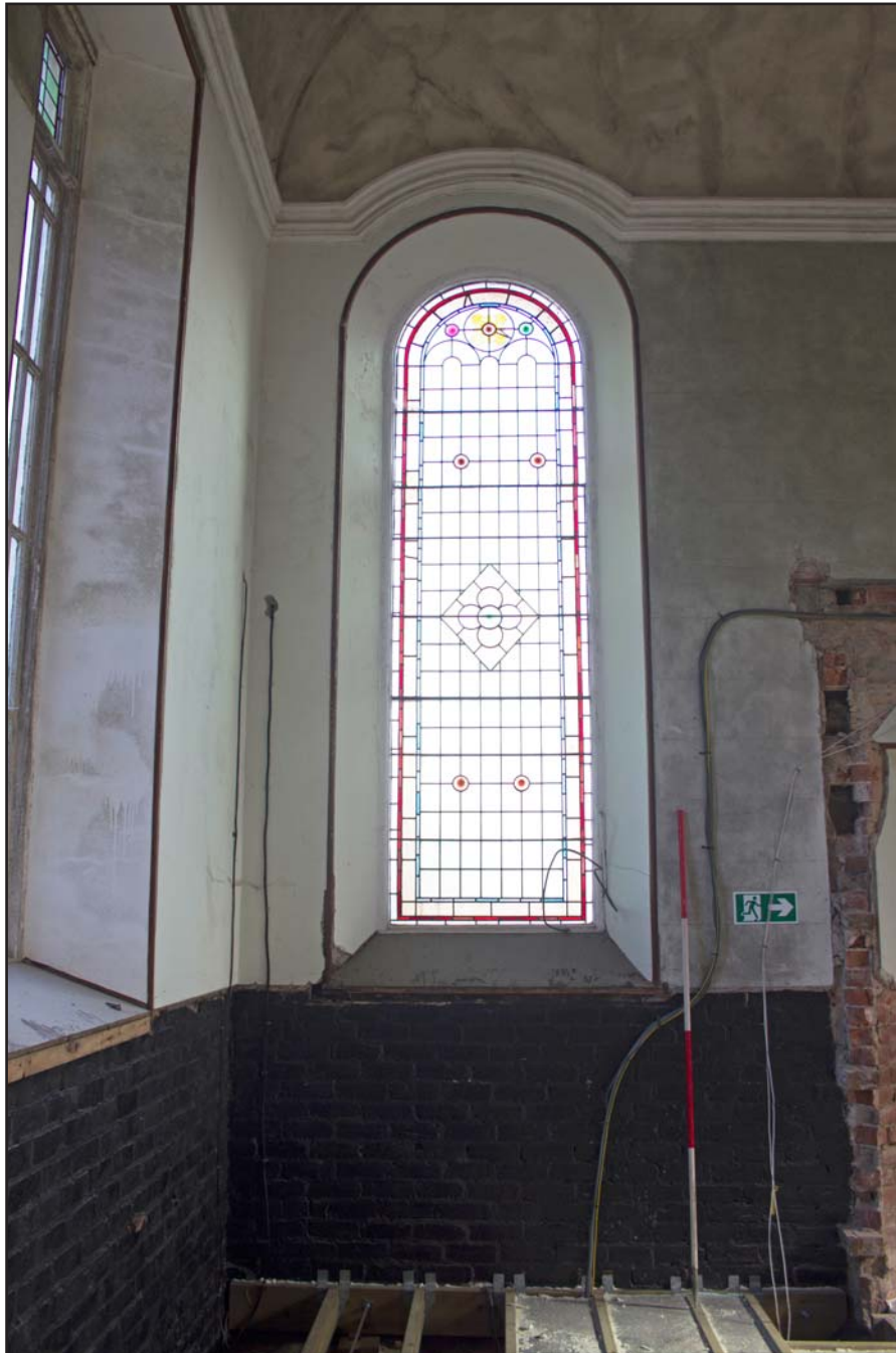
Plate 37: Gable round-headed window (left), internal shot, at Capel Carmel, Carmel Road, Carmel, Flintshire - from the south - 2.00m
