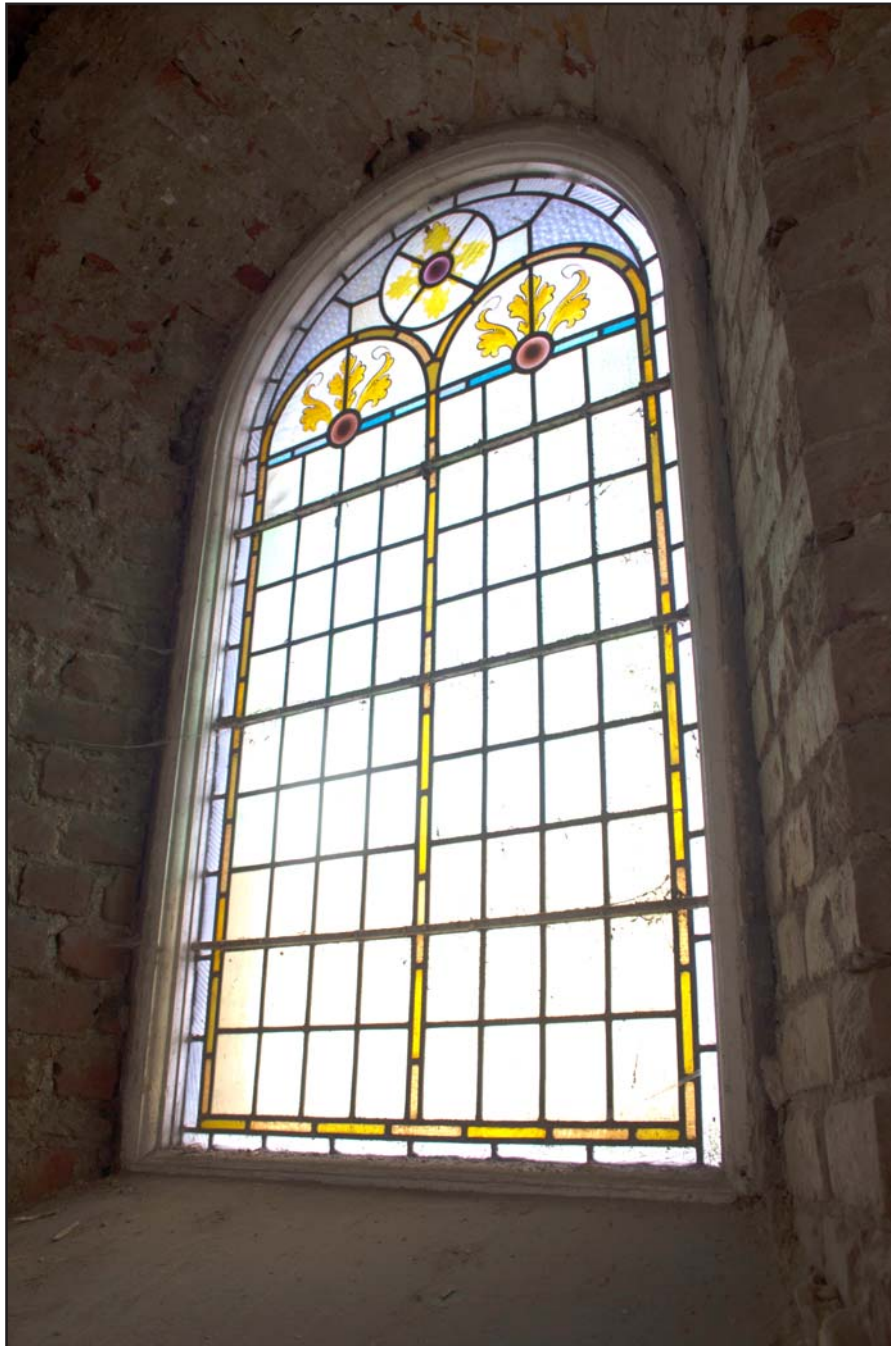
Plate 28: Northern window of porch, internal shot, at Capel Carmel, Carmel Road, Carmel, Flintshire - from the southeast - no scale
