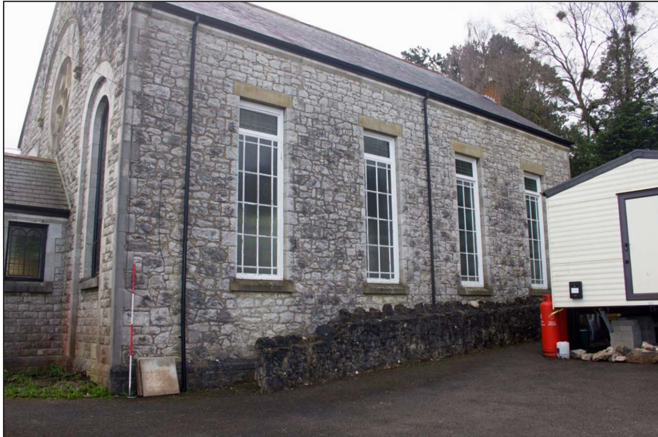
Plate 06: Shot showing western elevation of Capel Carmel, Carmel Road, Carmel, Flintshire - from the northwest - 2.00m scale
