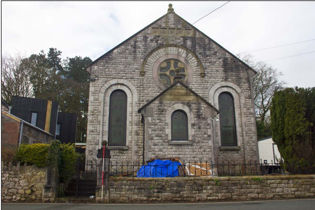
Plate 04: Shot showing Principal elevation of Capel Carmel, Carmel Road, Carmel, Flintshire - from the north - 2.00m scale
