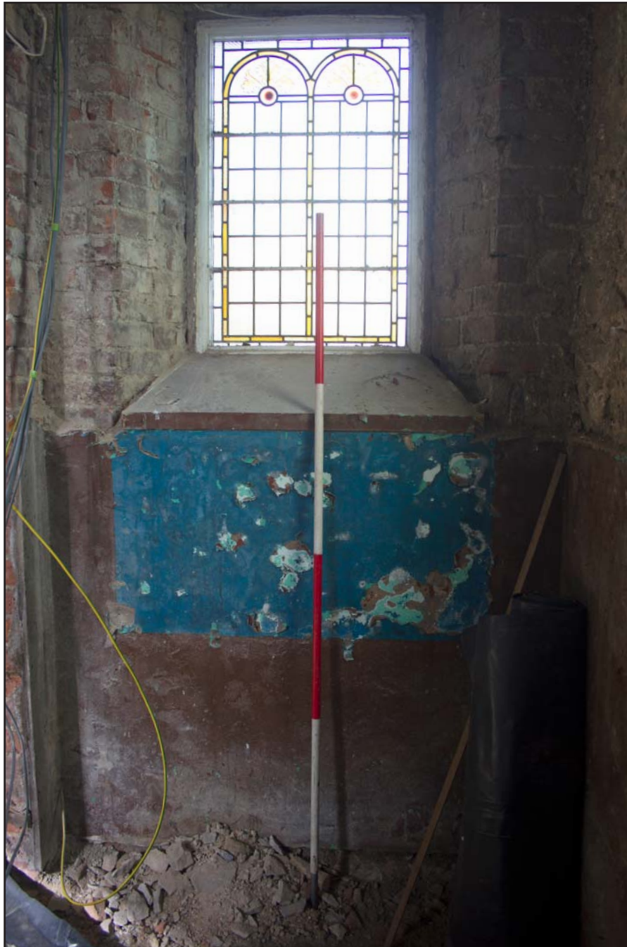
Plate 26: Western window of porch, internal shot, at Capel Carmel, Carmel Road, Carmel, Flintshire - from the east - 2.00m
