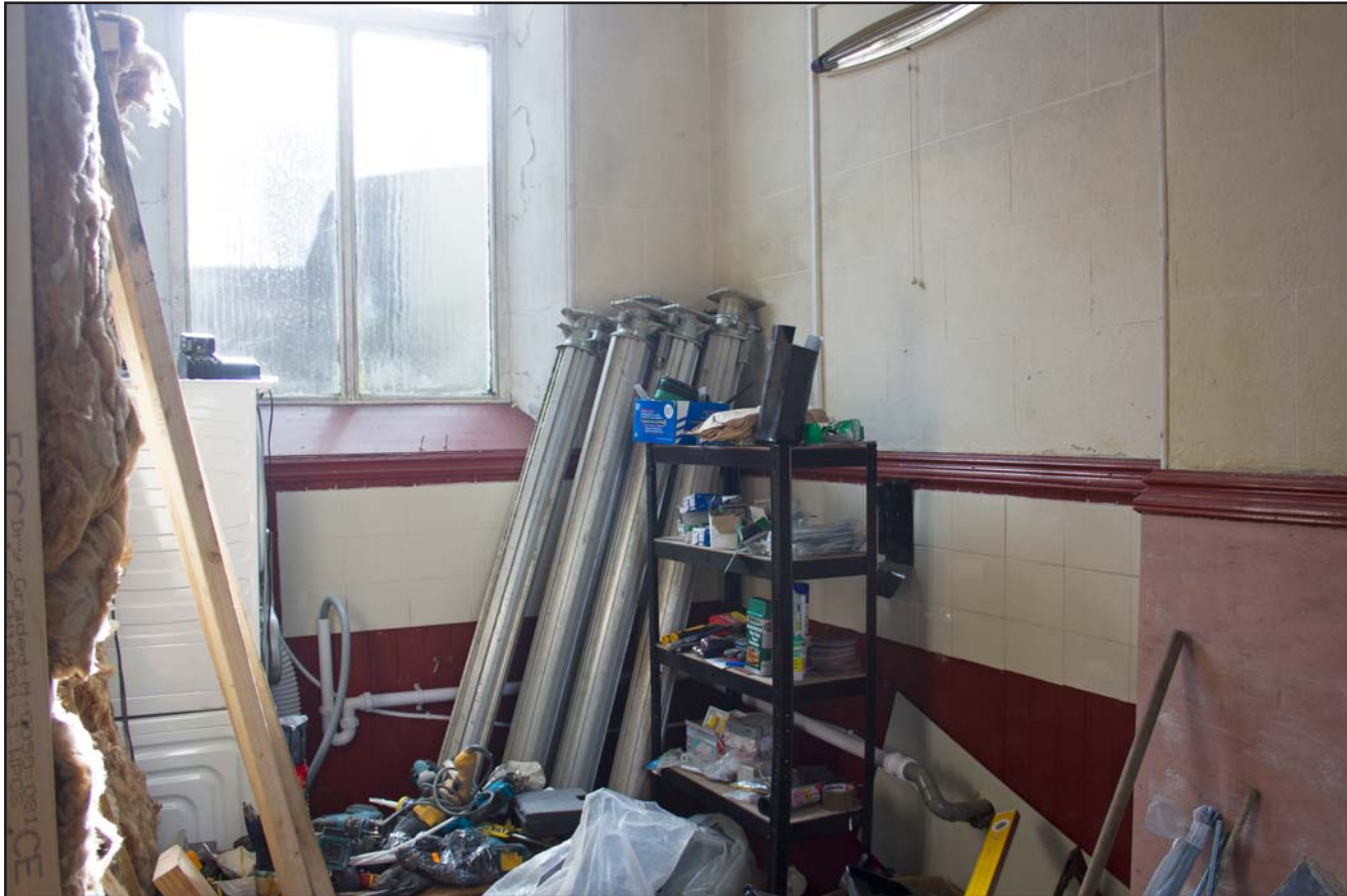
Plate 53: The Vestry, internal shot, at Capel Carmel, Carmel Road, Carmel, Flintshire - from the northwest - no scale
