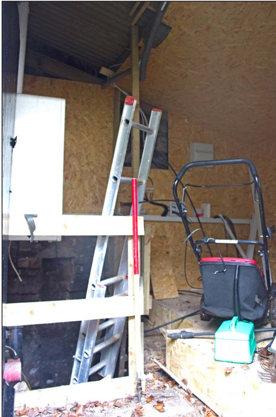
Plate 55: The Boiler Room, internal shot, at Capel Carmel, Carmel Road, Carmel, Flintshire - from the west - 2.00m scale
