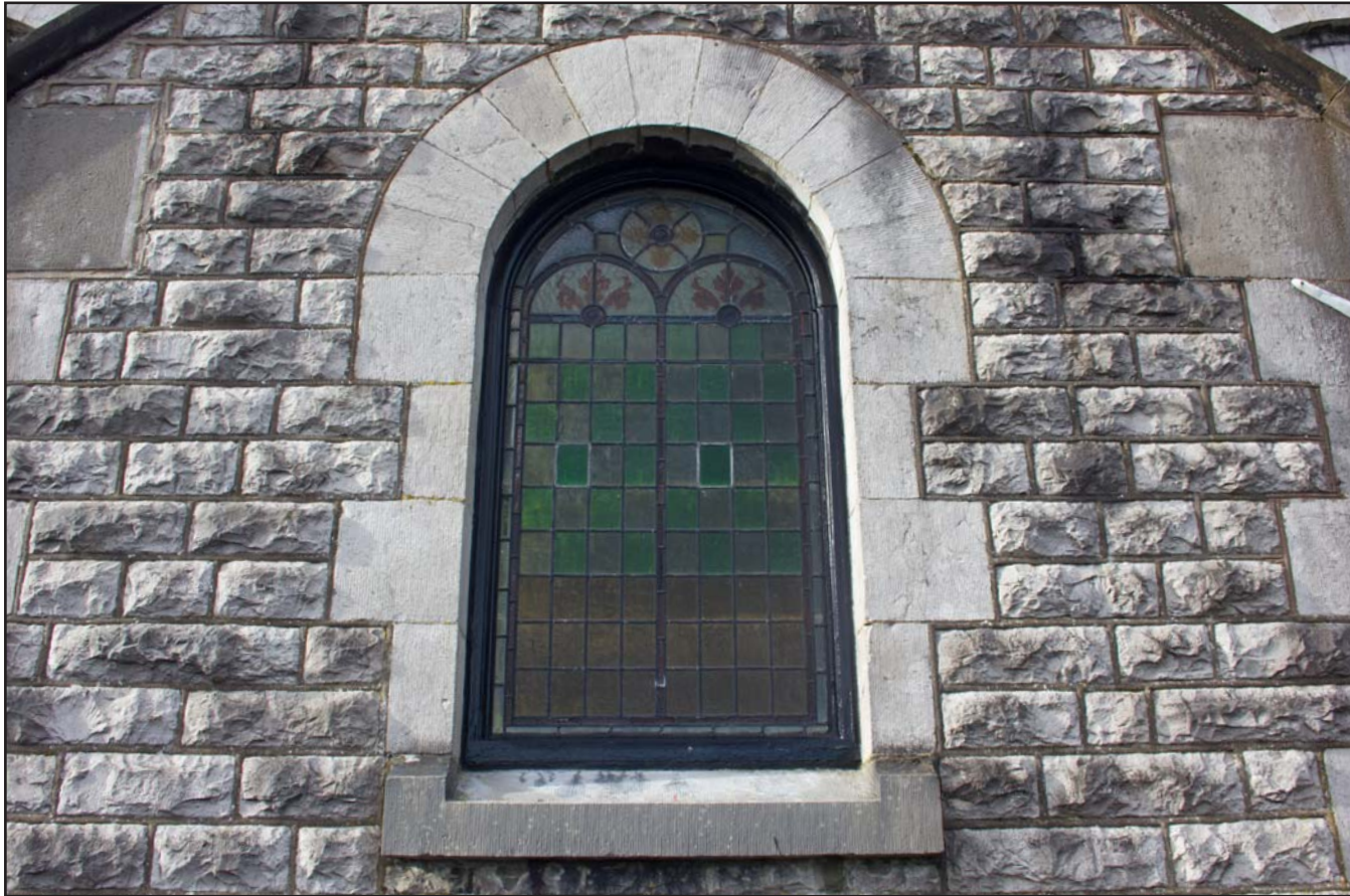
Plate 18: Shot of porch window of Capel Carmel, Carmel Road, Carmel, Flintshire - from the north - no scale
