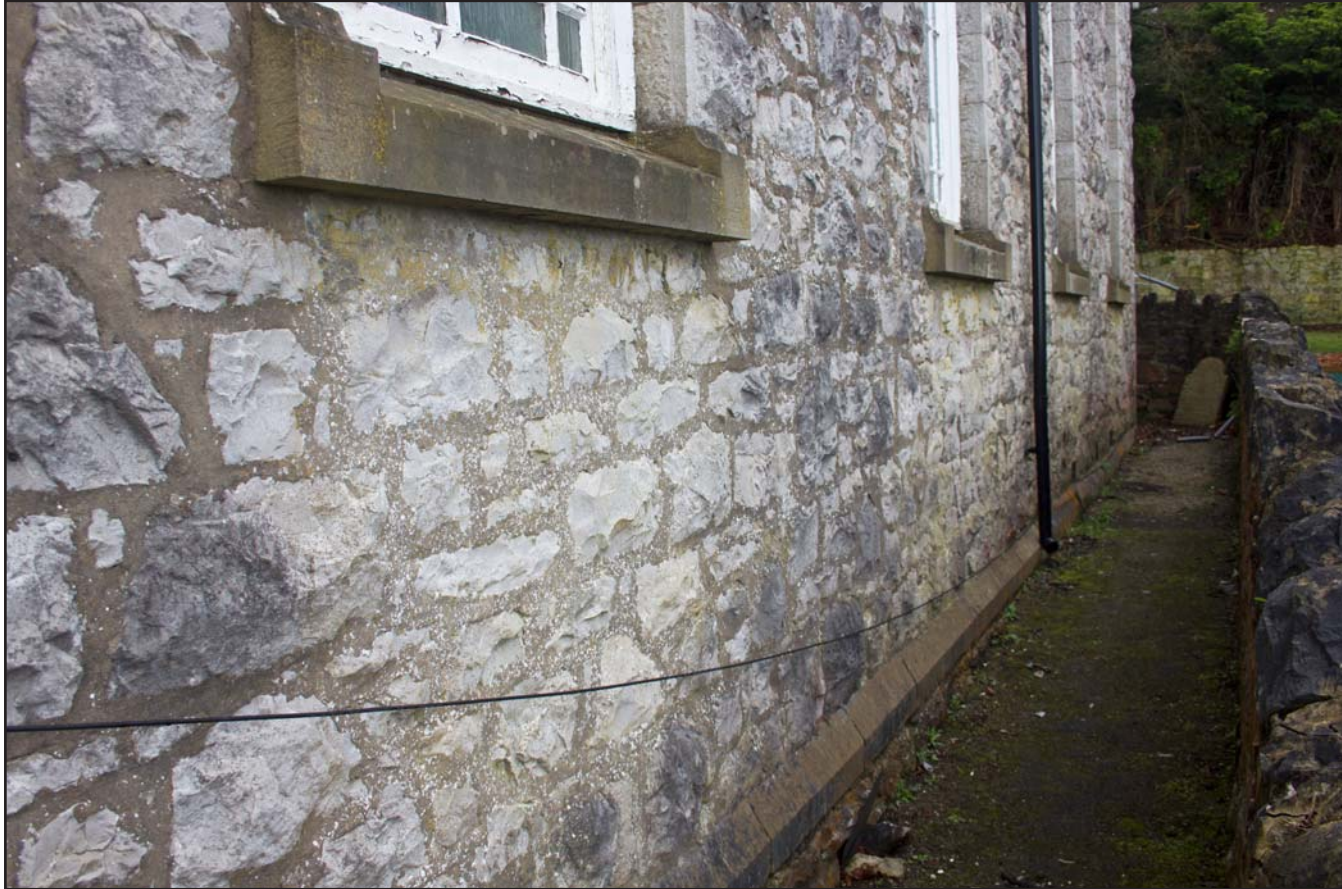
Plate 25: Wall cill of western elevation of Capel Carmel, Carmel Road, Carmel, Flintshire - from the southwest - no scale
