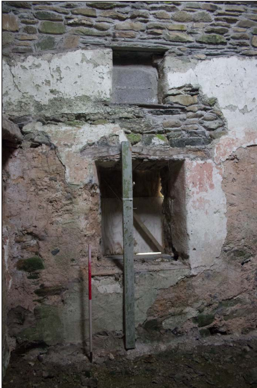
Plate 39: Internal shot, northeast elevation, (secondary, northwest extension), showing blocked windows, within the post medieval farmhouse at Penrhyn Garn, Rhydlydan, Pentrefeolas, Conwy - from the southwest - 1.00m scale
