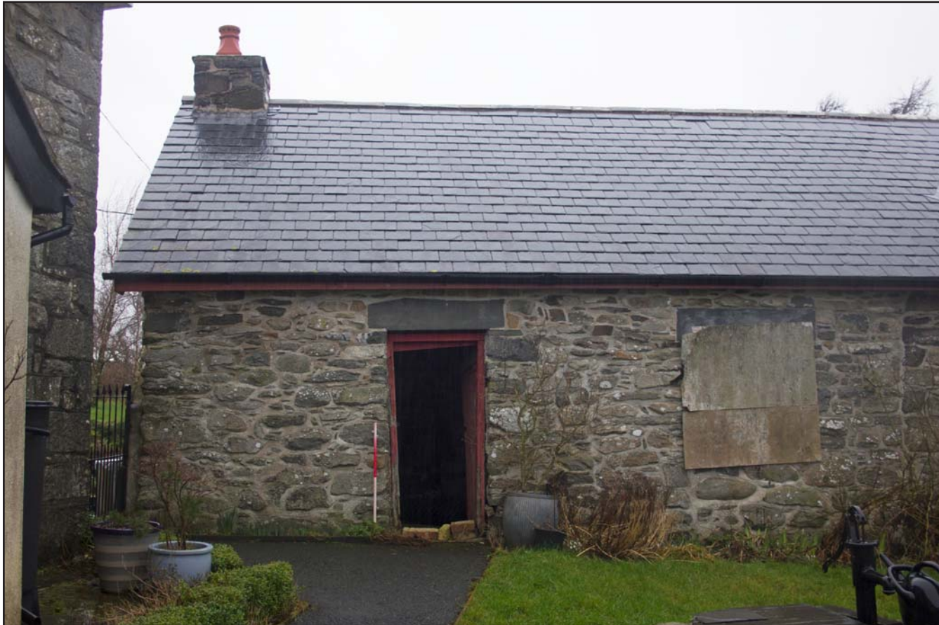
Plate 02: Southeast elevation (left) of the post medieval farmhouse at Penrhyn Garn, Rhydlydan, Pentrefeolas, Conwy - from the southeast - 1.00m scale
