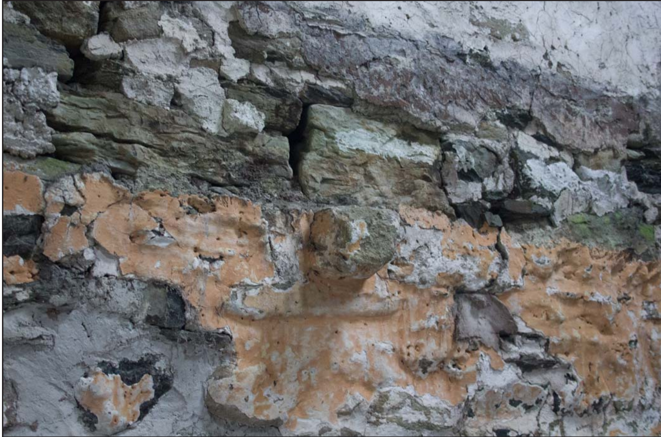
Plate 21: Corbel for presumed axial beam, southwest elevation, (Primary phase room) of the post medieval farmhouse at Penrhyn Garn, Rhydydan, Pentrefeolas, Conwy - from the east - no scale
