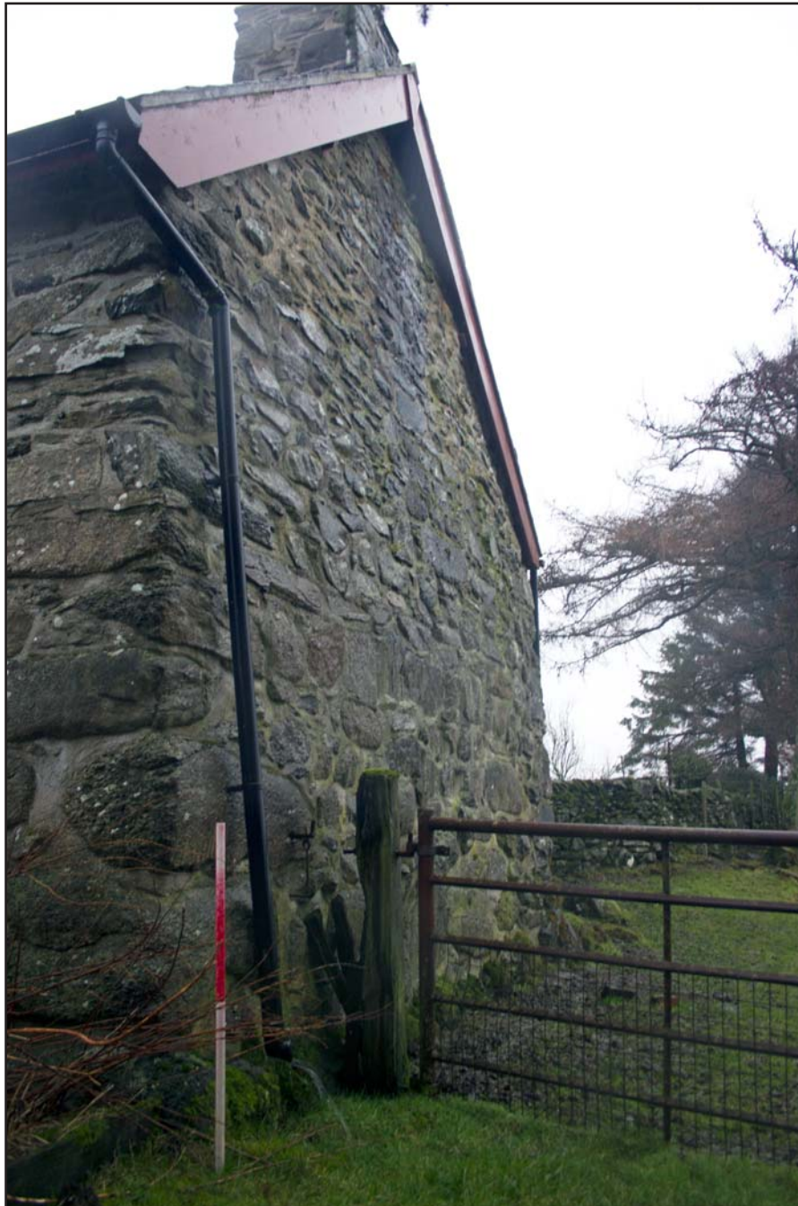
Plate 09: Northeast elevation (oblique) of the post medieval farmhouse at Penrhyn Garn, Rhydydan, Pentrefeolas, Conwy - from the east - 1.00m scale
