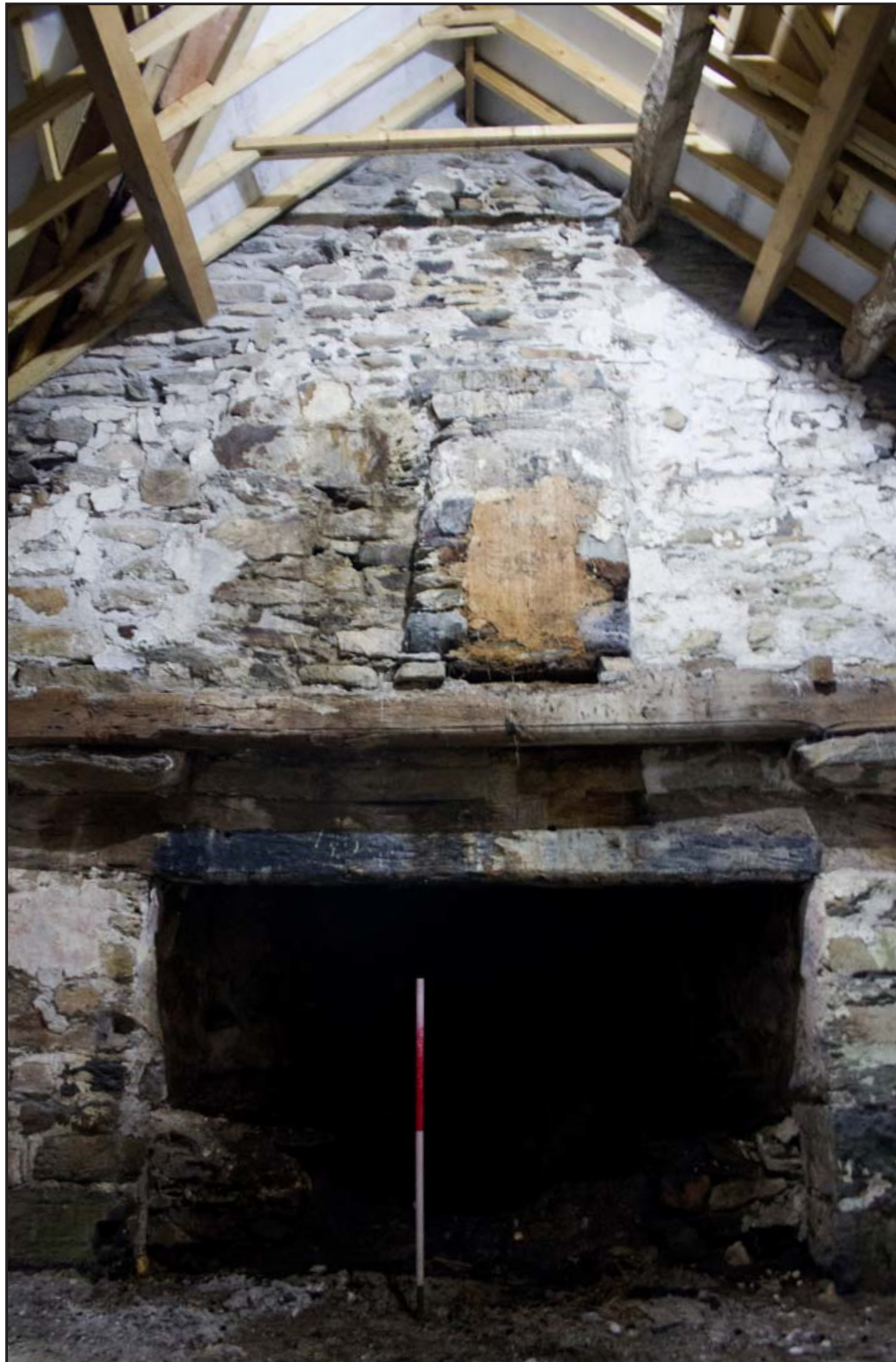
Plate 24: Internal shot, Fireplace with Bressumer Beam, transverse beam with Ovolo Moulding, First floor fireplace (Primary phase room) of the post medieval farmhouse at Penrhyn Garn, Rhydydan, Pentrefeolas, Conwy - from the southwest - 1.00m scale
