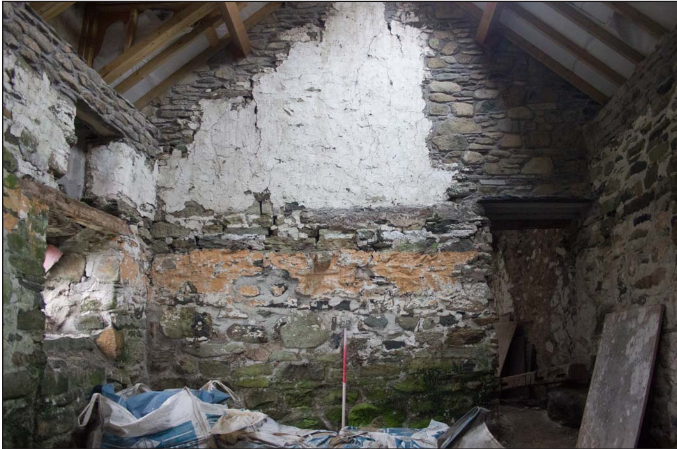
Plate 20: Internal shot, southwest elevation, (Primary phase room) of the post medieval farmhouse at Penrhyn Garn, Rhydlydan, Pentrefeolas, Conwy - from the northeast - 1.00m scale
