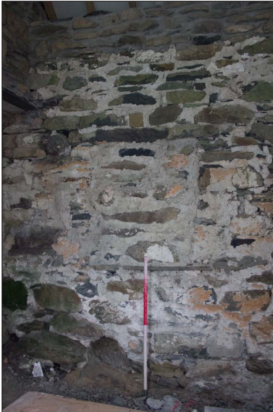
Plate 23: Internal shot, blocked window in northwest elevation, (Primary phase room) of the post medieval farmhouse at Penrhyn Garn, Rhydydan, Pentrefeolas, Conwy - from the southeast - 1.00m scale
