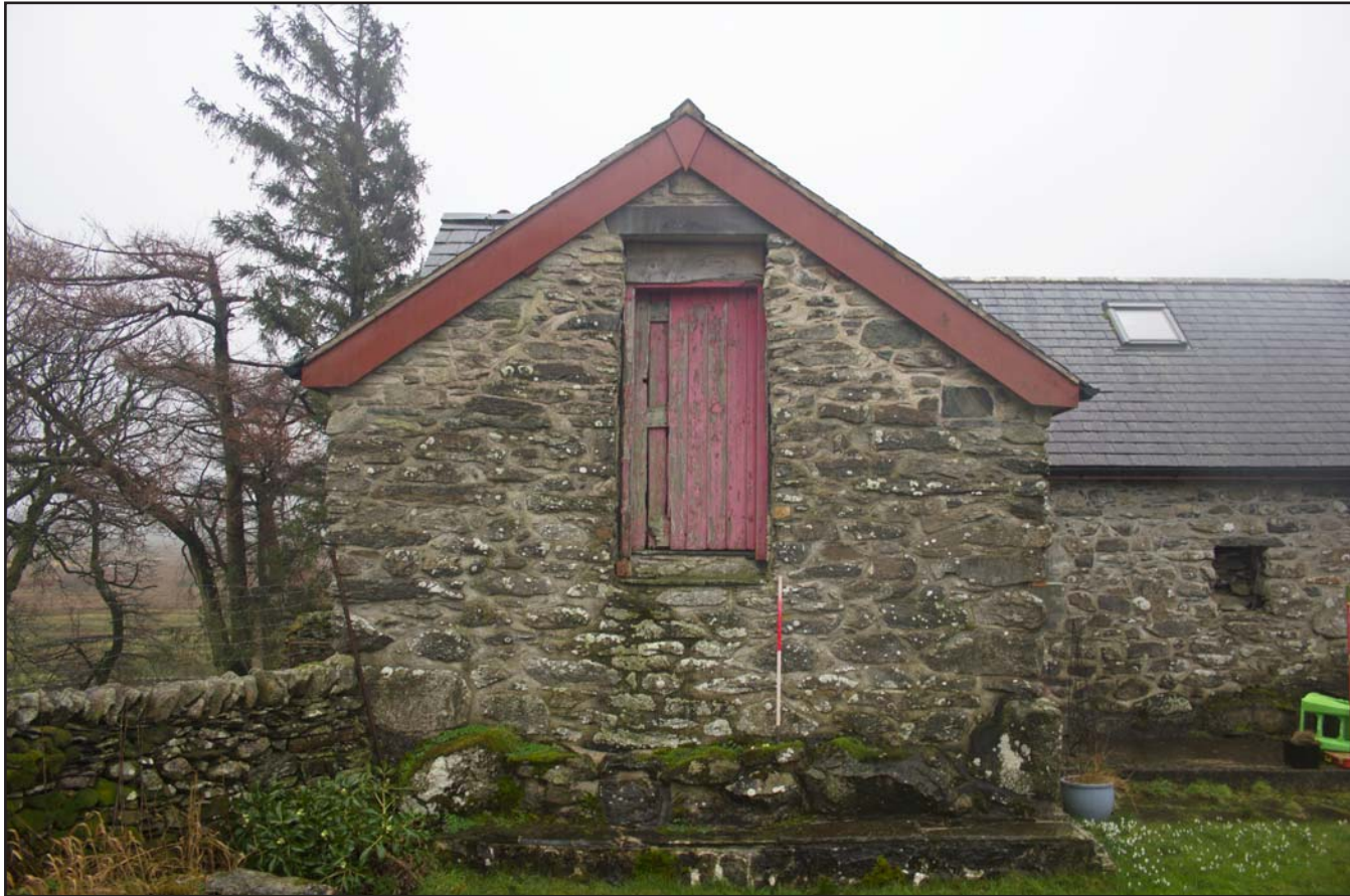
Plate 12: Northwest elevation (left) of the post medieval farmhouse at Penrhyn Garn, Rhydlydan, Pentrefeolas, Conwy - from the northwest - 1.00m scale
