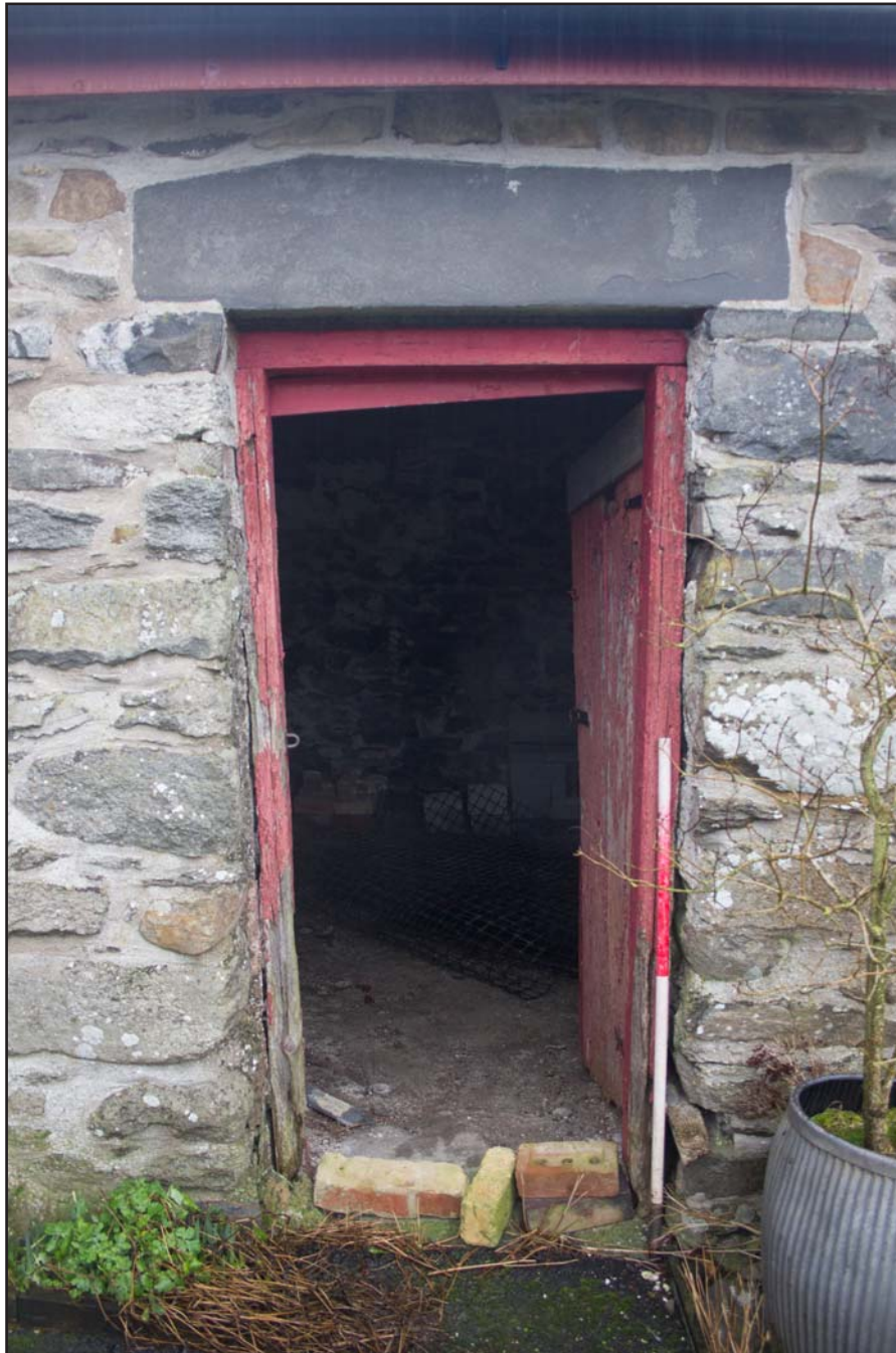
Plate 07: Doorway (Secondary phase) of the post medieval farmhouse at Penrhyn Garn, Rhydydan, Pentrefeolas, Conwy - from the southeast - 1.00m scale
