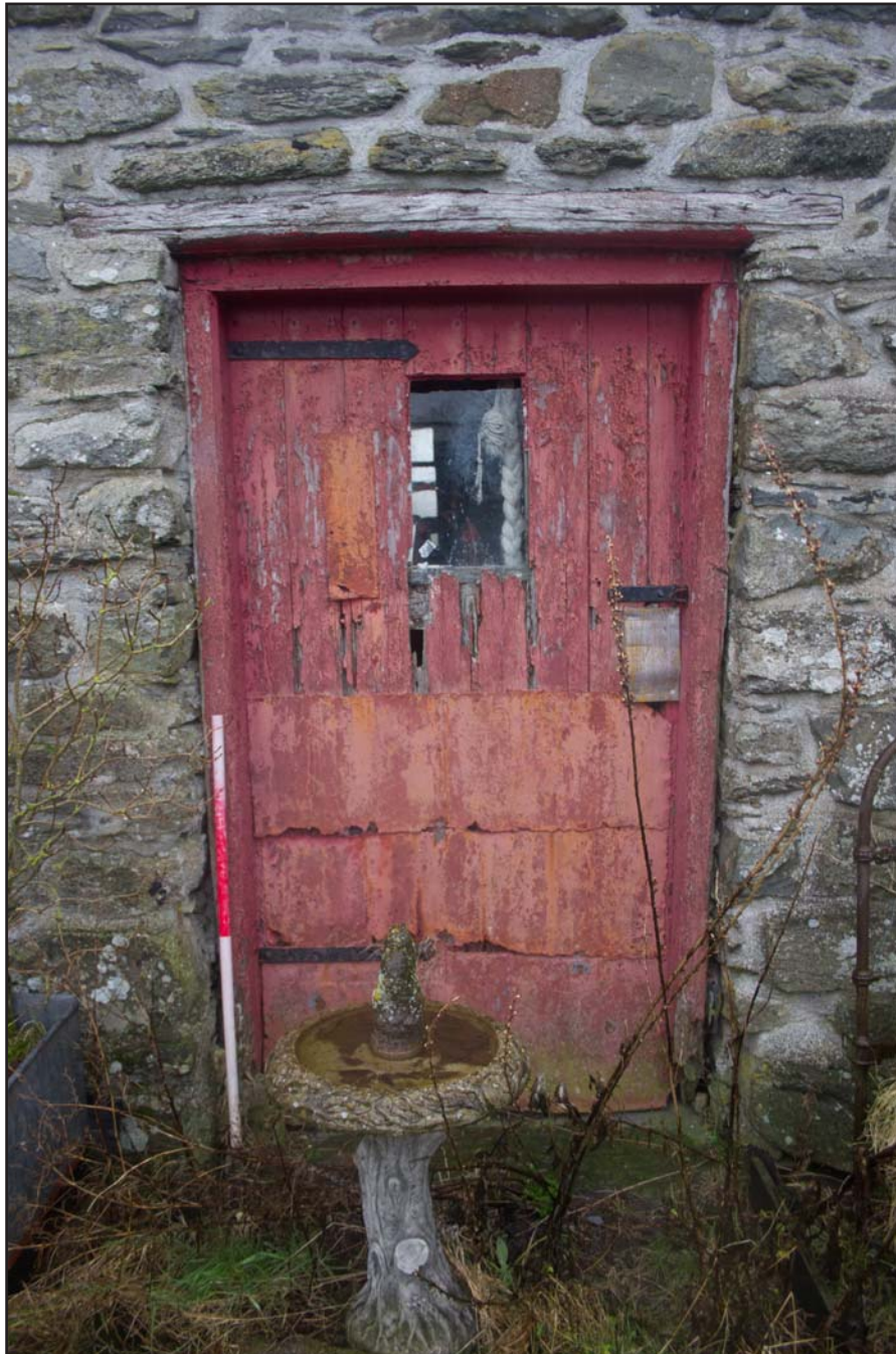
Plate 06: Doorway (Primary phase) of the post medieval farmhouse at Penrhyn Garn, Rhydlydan, Pentrefeolas, Conwy - from the southeast - 1.00m scale
