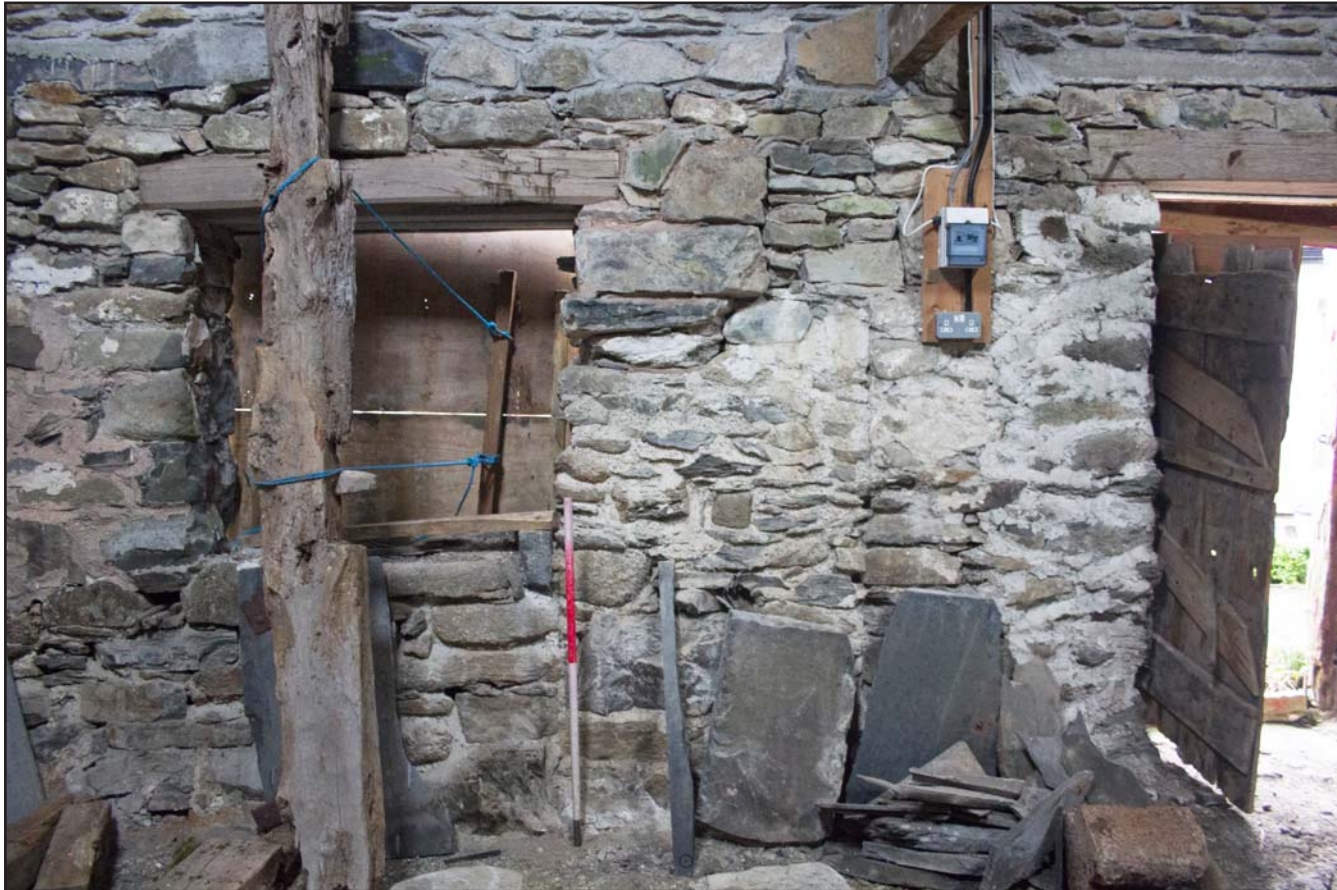
Plate 37: Internal shot, blocked up doorway in southeast elevation, (secondary phase room) of the post medieval farmhouse at Penrhyn Garn, Rhydlydan, Pentrefeolas, Conwy - from the northwest - 1.00m scale
