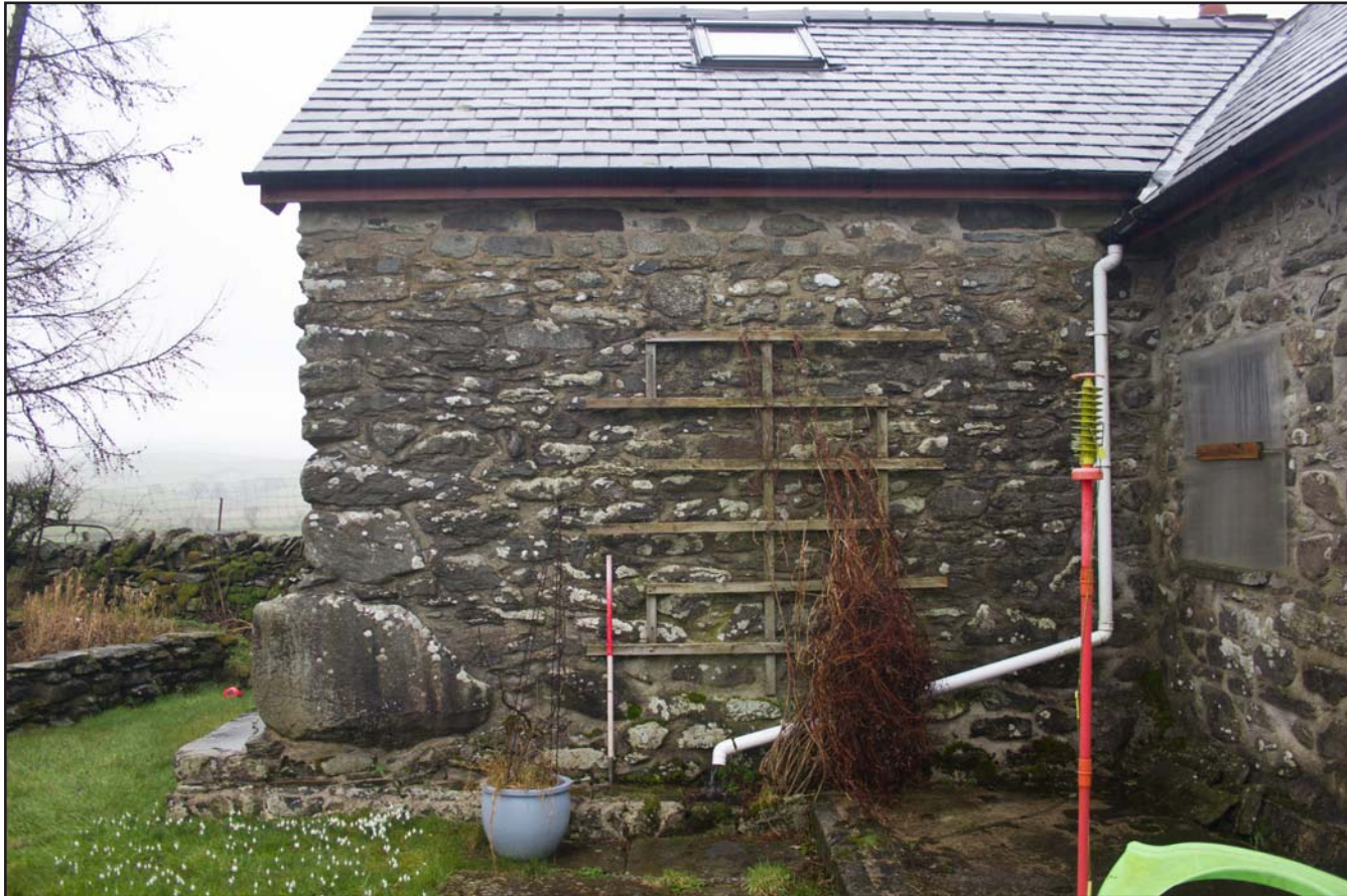
Plate 15: Southwest elevation of the north western extension to post medieval farmhouse at Penrhyn Garn, Rhydlydan, Pentrefeolas, Conwy - from the northwest - 1.00m scale
