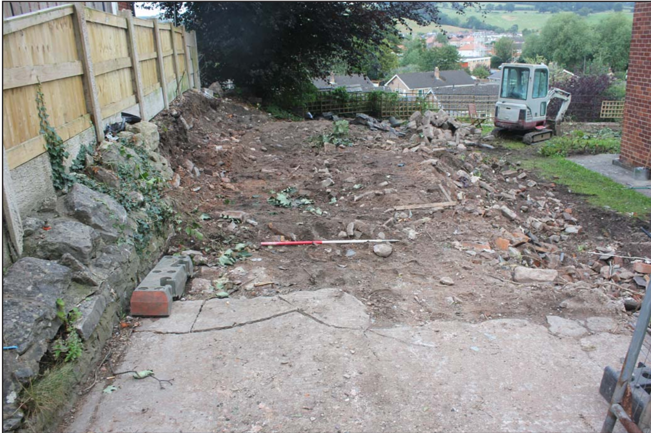
Plate 01: Pre excavation shot of site, on land at Crannog, Prior Street, Ruthin, Denbighshire - from the east - 1.00m scale
