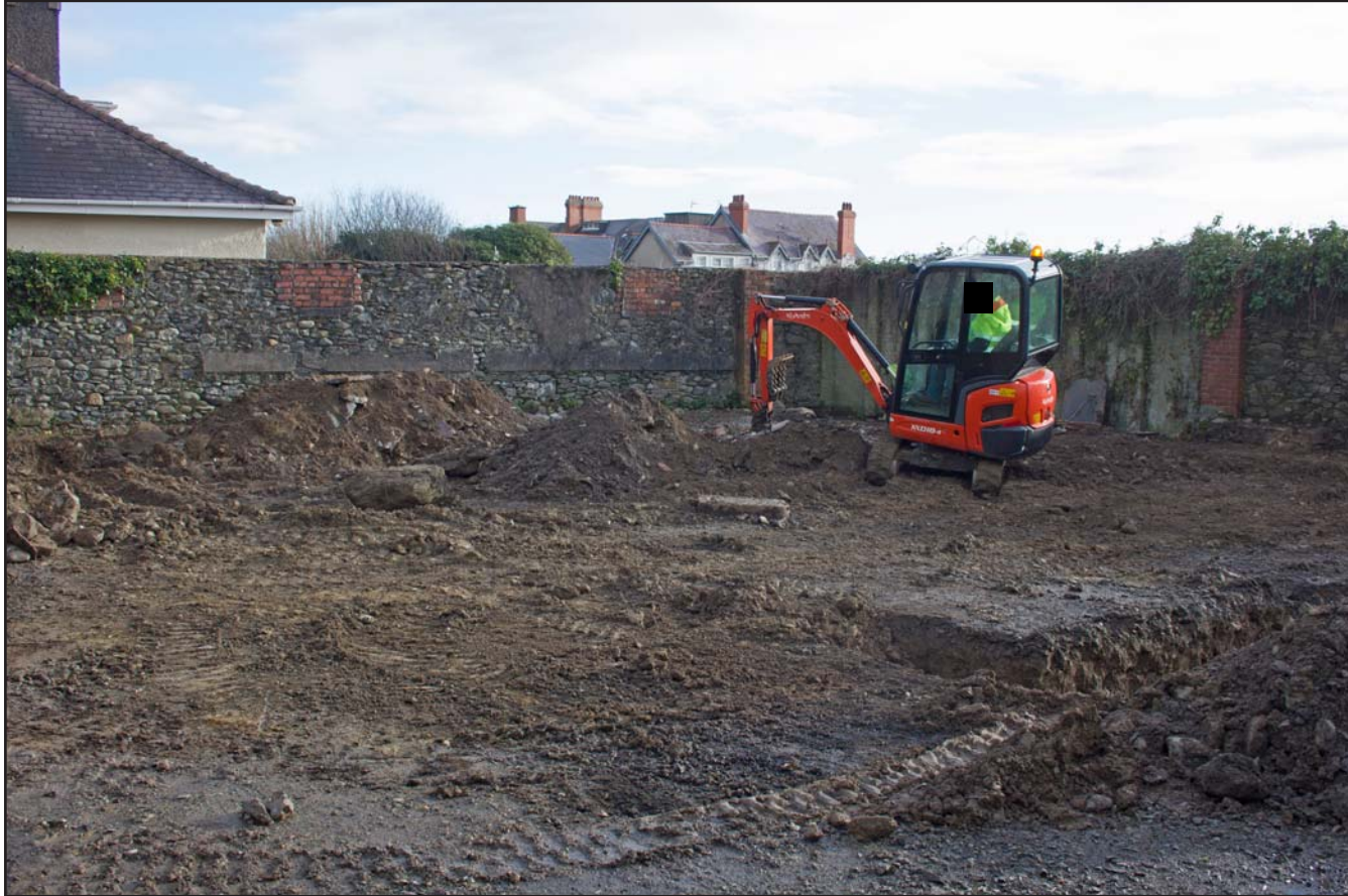
Plate 37: Working shot closing down of trenches, at Former Prince of Wales Car Park, High Street, Criccieth - from the northwest - no scale
