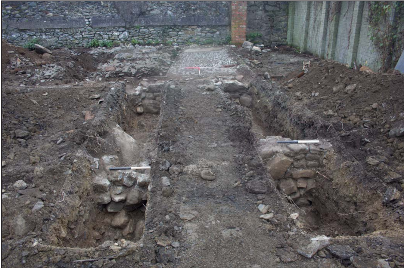
Plate 11: Wall foundation (1003/1004), at Former Prince of Wales Car Park, High Street, Criccieth - from the west - (2x) 1.00m scale, (2x) 0.50m scale
