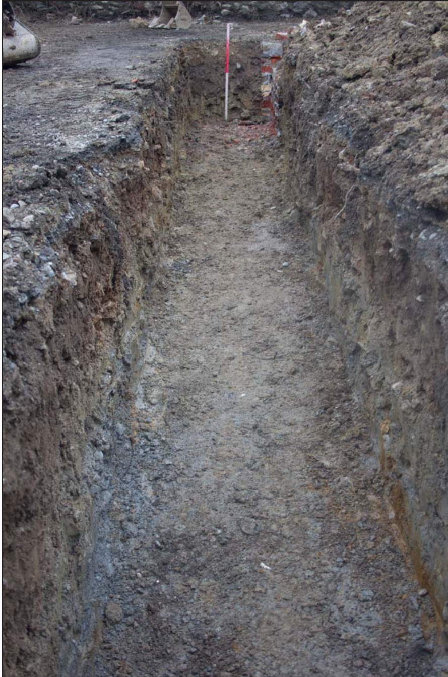
Plate 28: Trench A post excavation shot, at Former Prince of Wales Car Park, High Street, Criccieth - from the north - 1.00m scale
