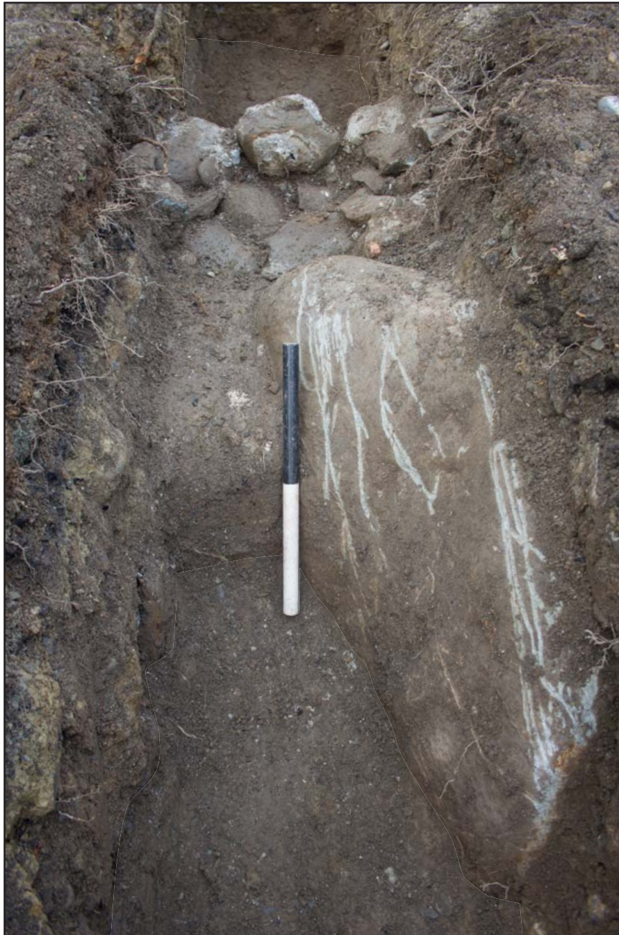
Plate 17: Wall foundation (1003) elevation shot, at Former Prince of Wales Car Park, High Street, Crickieth - from the east - 0.50m scale
