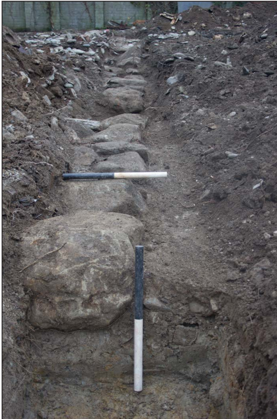
Plate 21: Wall foundation (1002) elevation, at Former Prince of Wales Car Park, High Street, Crickieth - from the north - (2x) 0.50m scale
