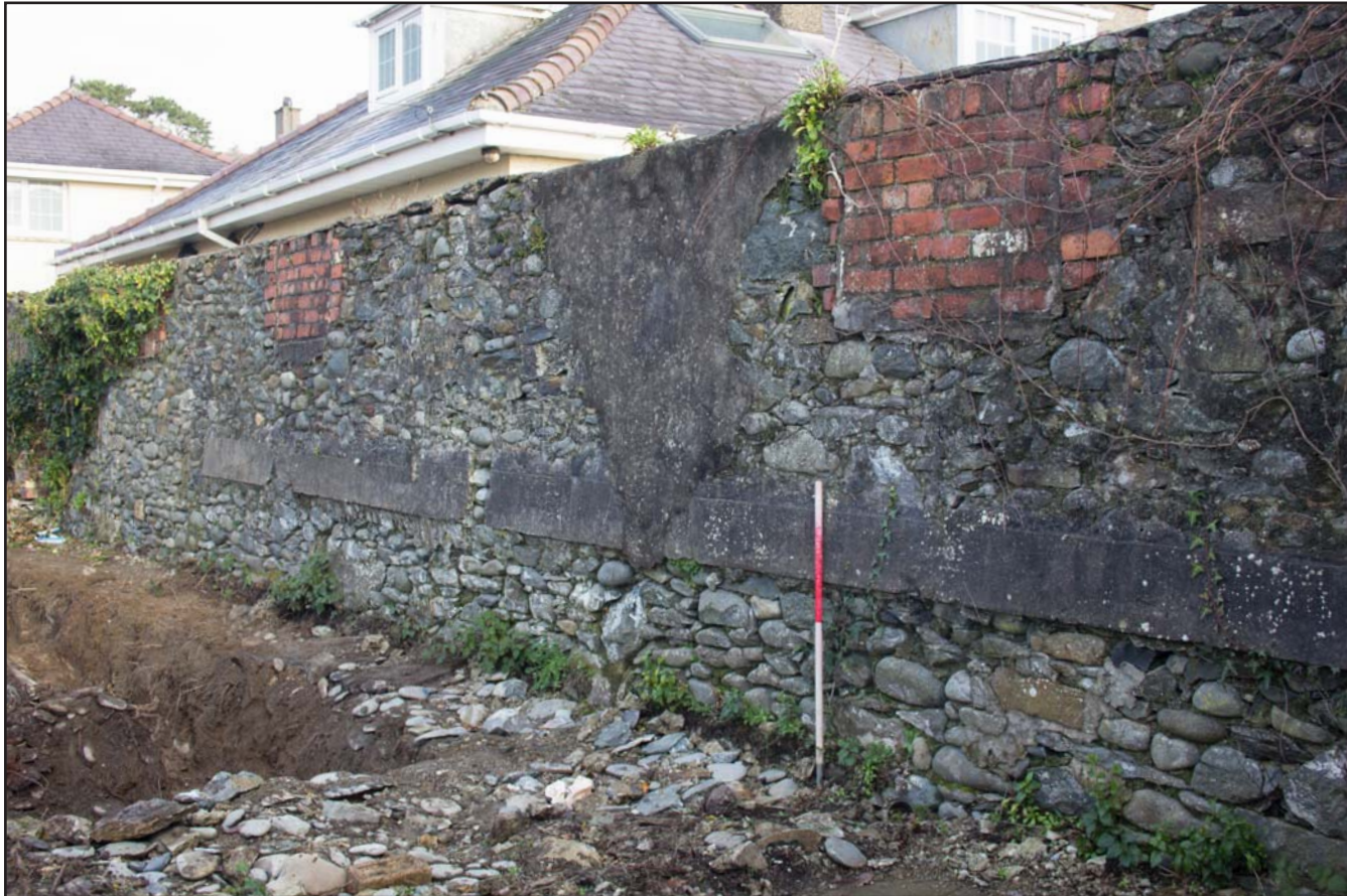
Plate 26: Surviving eastern perimeter wall of the site, at Former Prince of Wales Car Park, High Street, Criccieth - from the southwest - 1.00m scale
