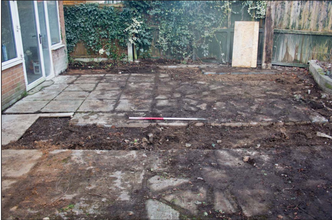
Plate 08: Pre excavation shot of rear extension, at no 4. Oaklands Avenue, Rhosnesney, Wrexham - from the northeast - 1.00m scale
