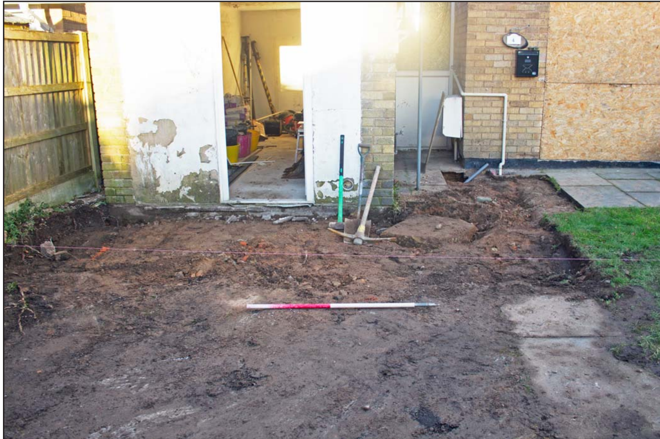
Plate 01: Pre excavation shot of front extension, at no 4. Oaklands Avenue, Rhosnesney, Wrexham - from the southeast - 1.00m scale
