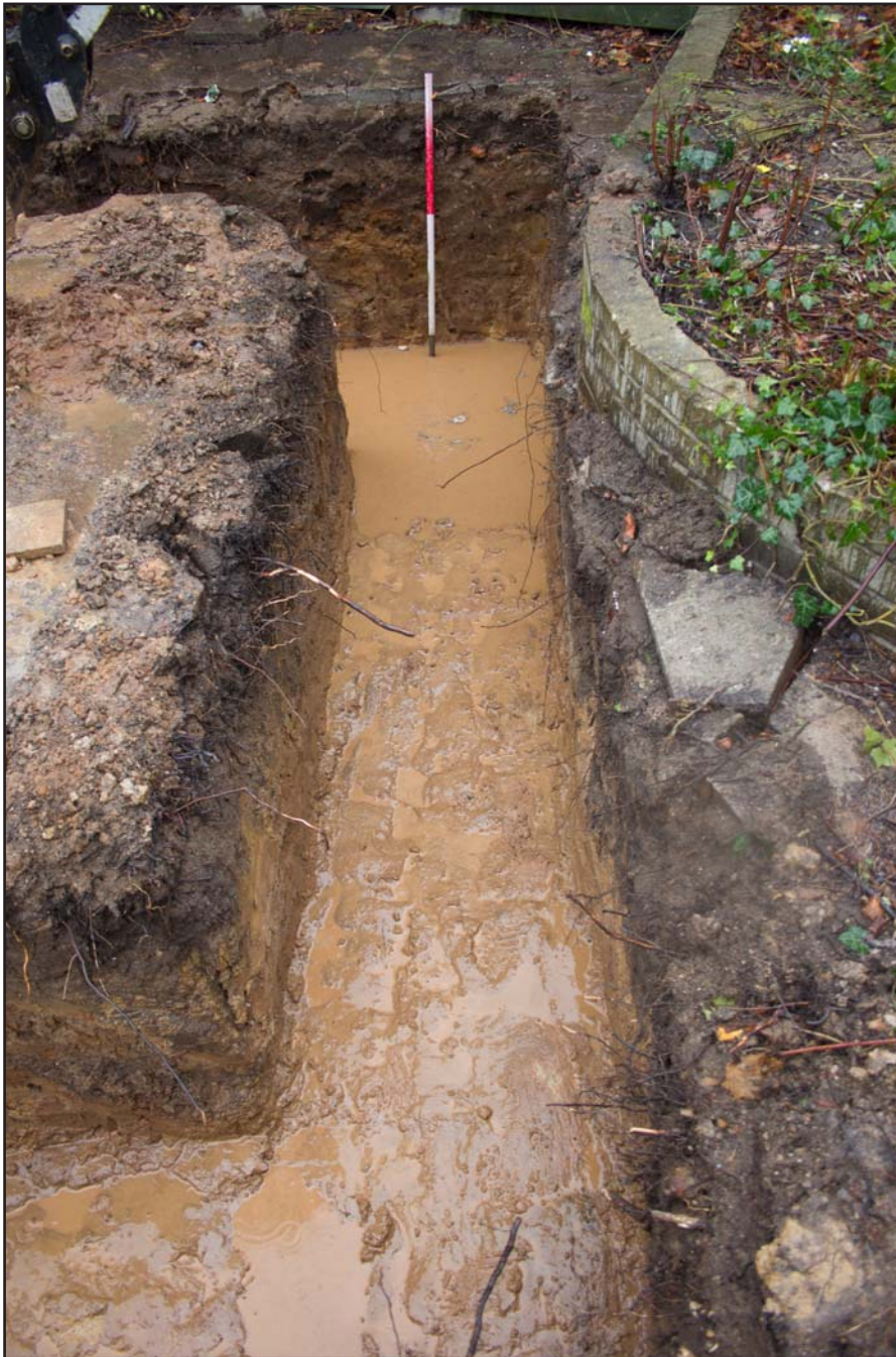
Plate 13: Post excavation shot of north western trench (rear extension), at no 4. Oaklands Avenue, Rhosnesney, Wrexham - from the northeast - 1.00m scale
