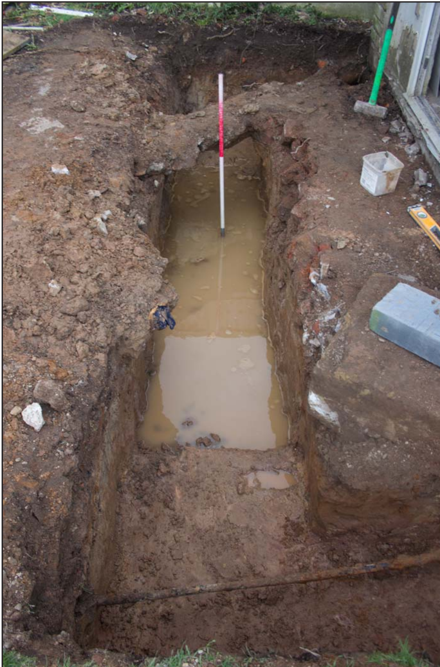
Plate 03: Post excavation shot of SW trench (front extension), at no 4. Oaklands Avenue, Rhosnesney, Wrexham - from the northeast - 1.00m scale
