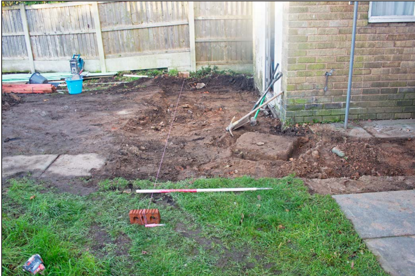
Plate 02: Pre excavation shot of front extension, at no 4. Oaklands Avenue, Rhosnesney, Wrexham - from the northeast - 1.00m scale
