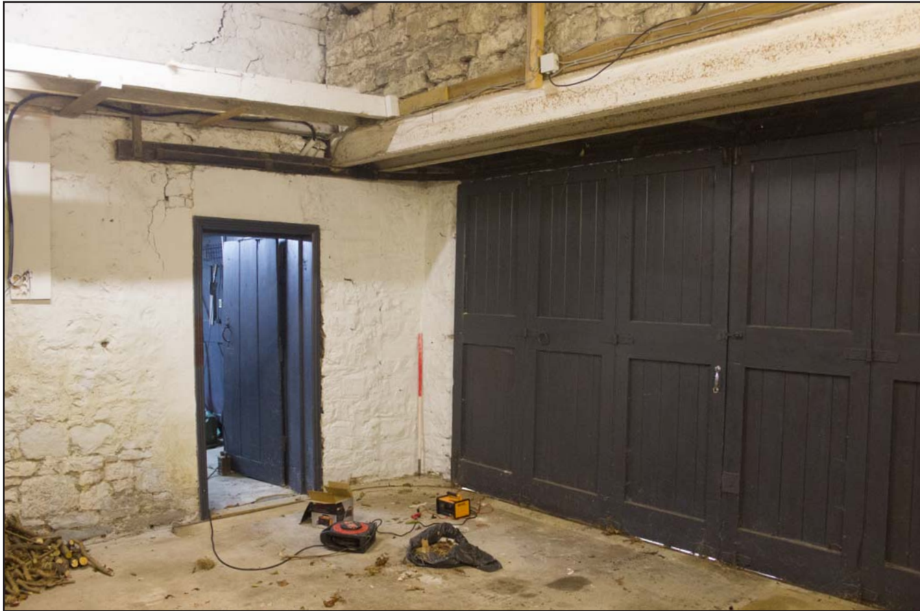
Plate 22: Ground Floor, Main Garage, of Coach House at Hafod Ynys, Rhewl, Denbighshire - from the northwest - 1.00m scale
