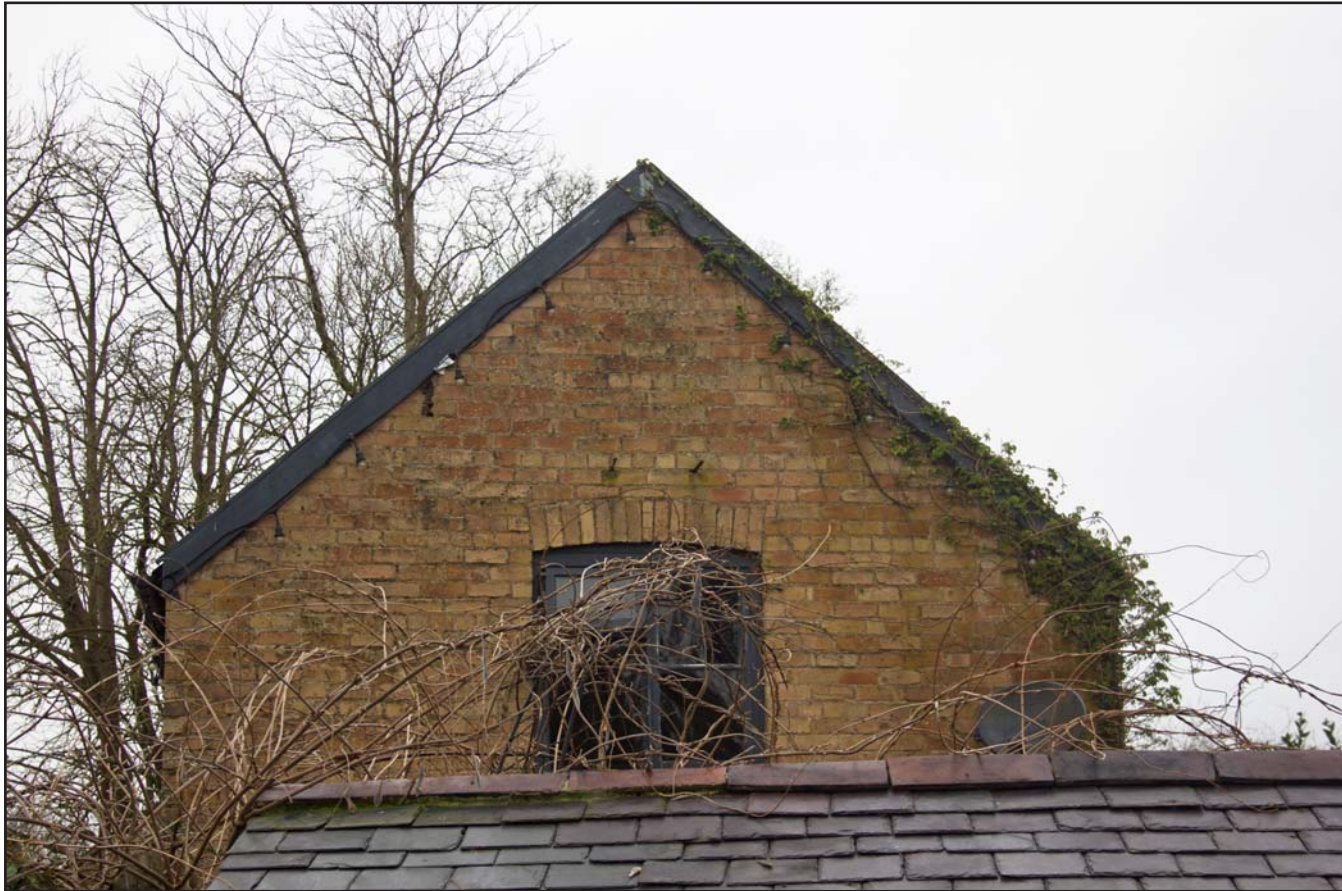
Plate 06: Eastern elevation (upper part), of Coach House at Hafod Ynys, Rhewl, Denbighshire - from the east - 1.00m scale
