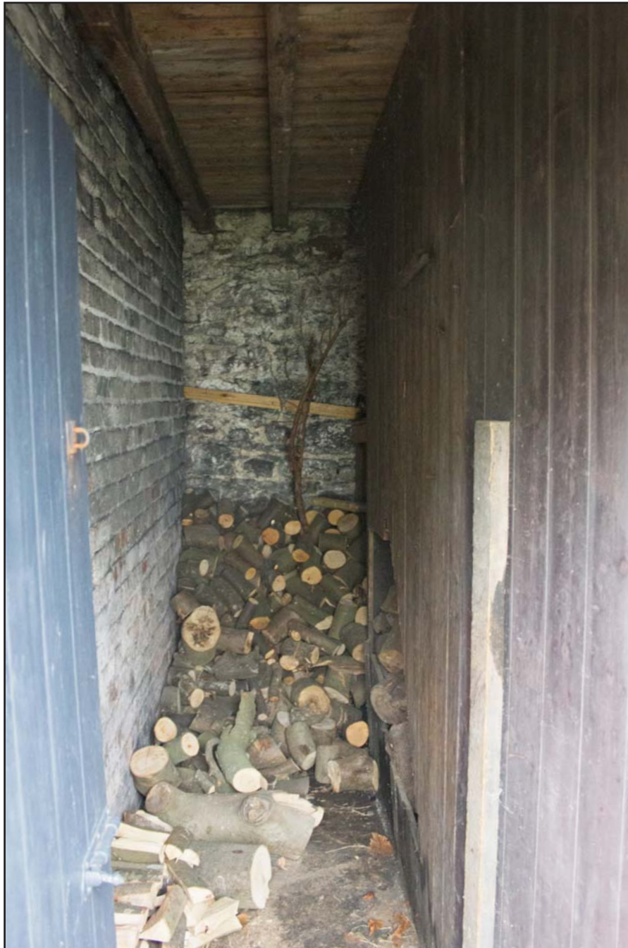
Plate 21: Ground Floor, log store, of Coach House at Hafod Ynys, Rhewl, Denbighshire - from the south - no scale
