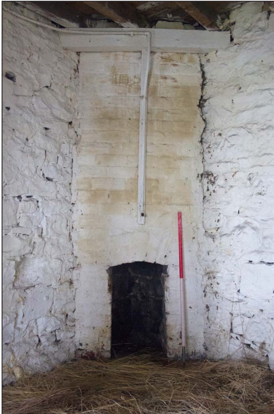
Plate 20: Ground Floor, western room, of Coach House at Hafod Ynys, Rhewl, Denbighshire - from the southeast - 1.00m scale
