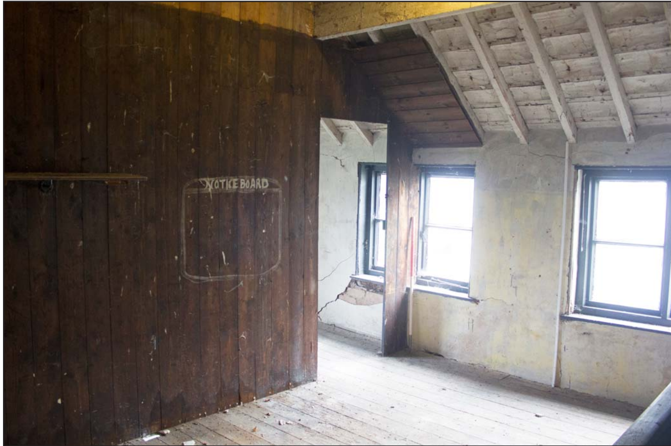
Plate 32: First Floor, eastern room, of Coach House at Hafod Ynys, Rhewl, Denbighshire - from the northwest - 1.00m scale
