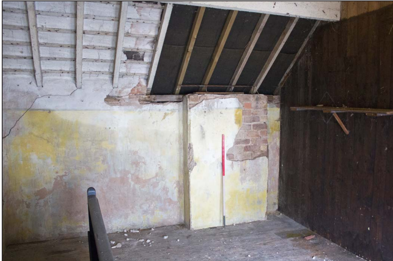
Plate 33: First Floor, eastern room, of Coach House at Hafod Ynys, Rhewl, Denbighshire - from the southwest - 1.00m scale
