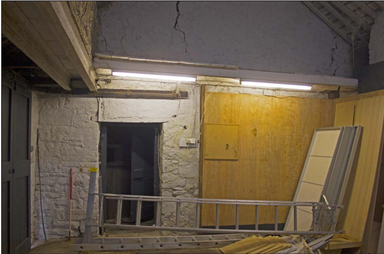
Plate 23: Ground Floor, Main Garage, of Coach House at Hafod Ynys, Rhewl, Denbighshire - from the east - 1.00m scale
