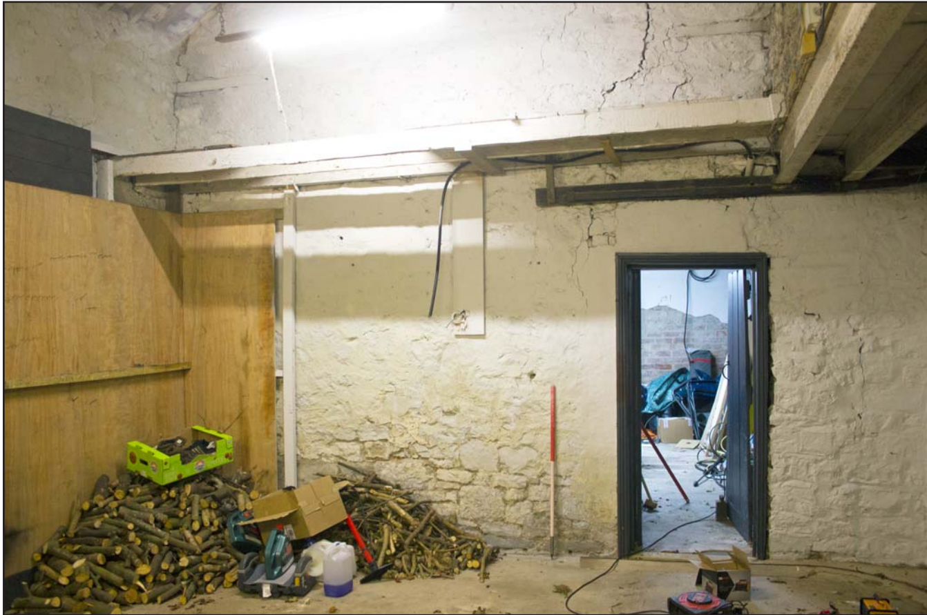
Plate 25: Ground Floor, Main Garage, of Coach House at Hafod Ynys, Rhewl, Denbighshire - from the west - 1.00m scale
