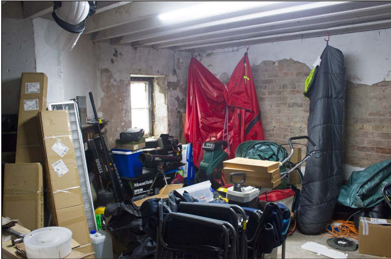
Plate 26: Ground Floor, eastern room, of Coach House at Hafod Ynys, Rhewl, Denbighshire - from the southwest - no scale
