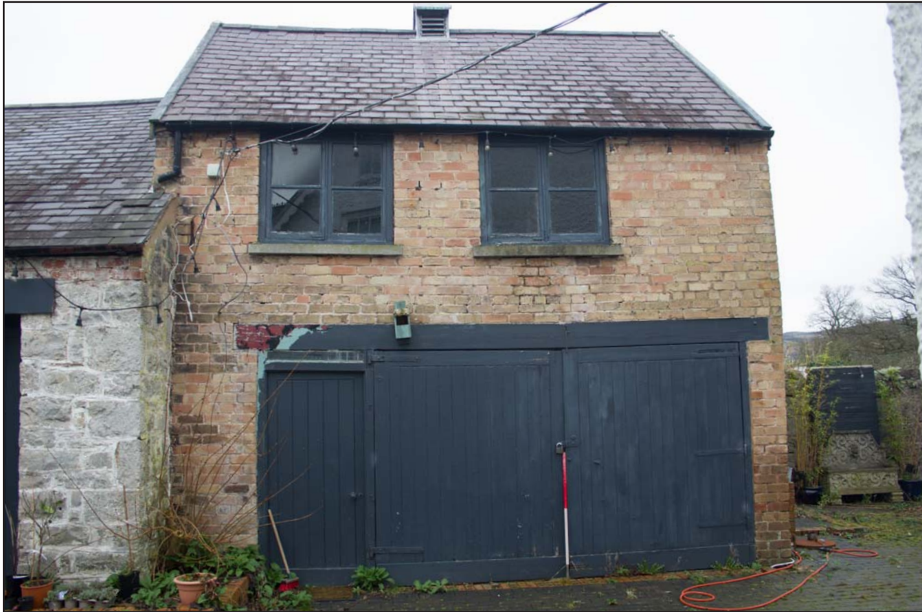
Plate 11: Southern elevation (right), of Coach House at Hafod Ynys, Rhewl, Denbighshire - from the south - 1.00m scale
