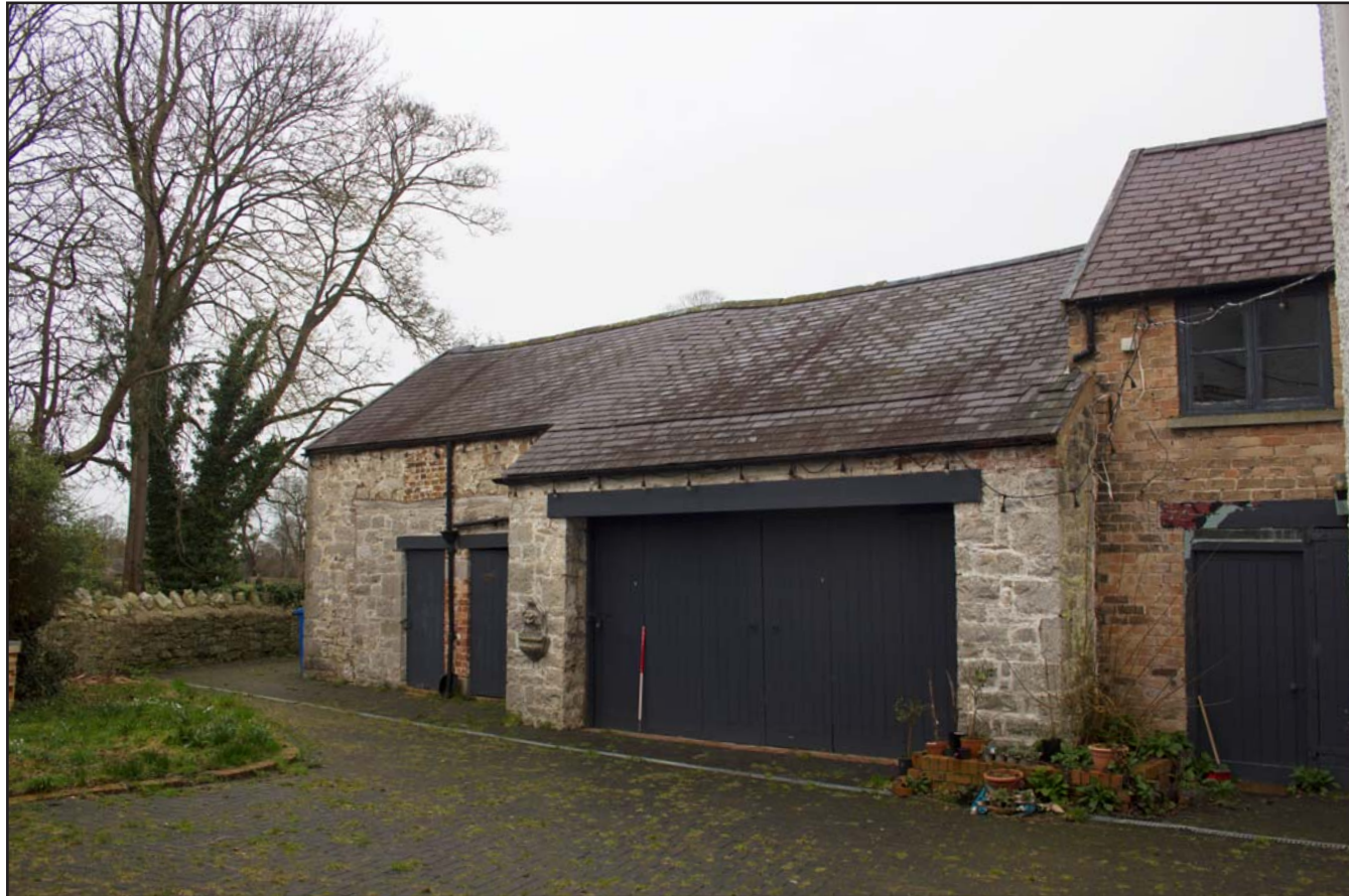
Plate 10: Oblique shot of southern elevation of Coach House at Hafod Ynys, Rhewl, Denbighshire - from the south- 1.00m scale
