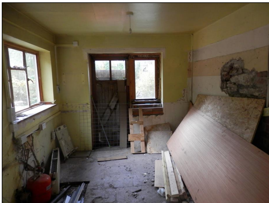
Plate 16: View looking SW across the interior of the lean-to extension to the rear of Brecon Lodge
