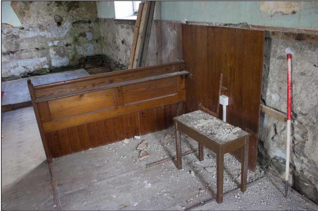
Plate 28: Example of pine timber panelling on south western elevation, Tŷ Capel, Denbigh Road, Llanfairtalhaiarn, Conwy - from the north - 1.00m scale
