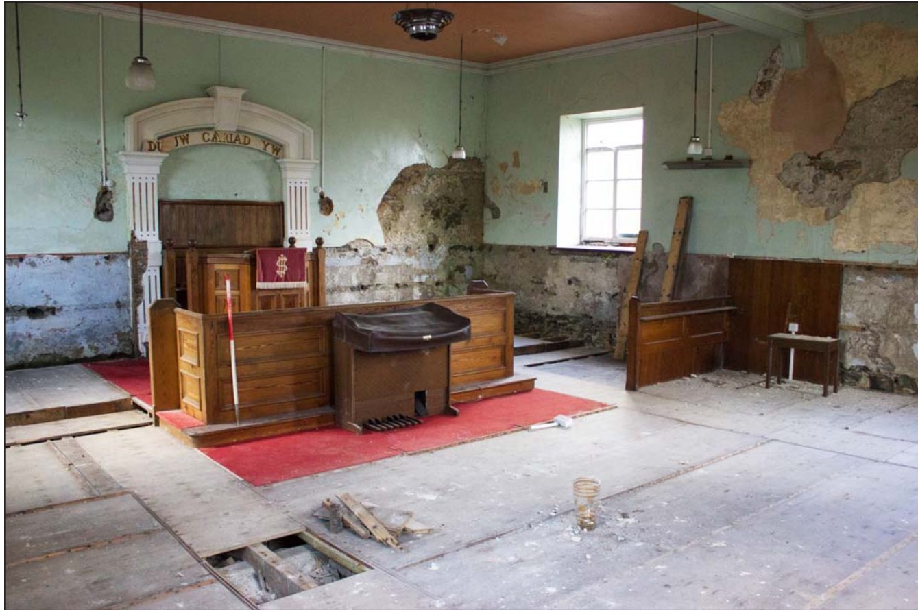
Plate 31: Oblique shot of chapel floor, Tŷ Capel, Denbigh Road, Llanfairtalhaiarn, Conwy - from the north - 1.00m scale
