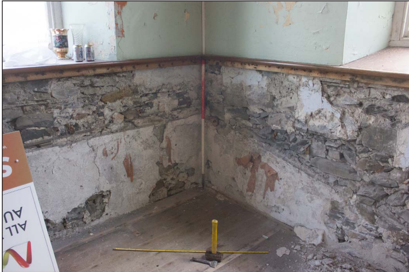
Plate 20: Internal shot, plaster line on north eastern elevation showing where tiered seating was previously located, Tŷ Capel, Denbigh Road, Llanfairtalhaiarn, Conwy - from the south - 1.00m scale
