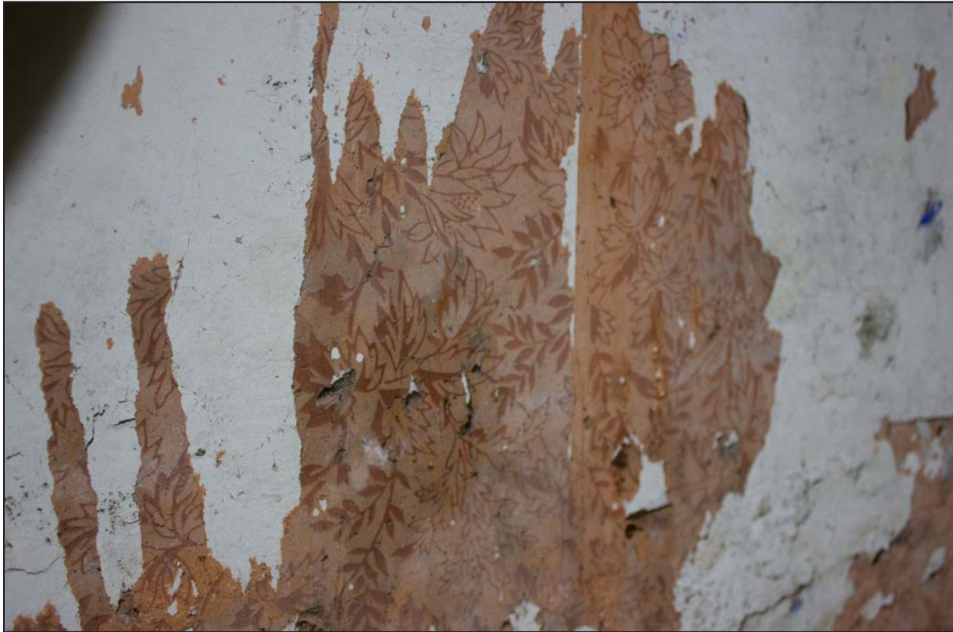
Plate 40: Example of wall paper on southeast elevation , Tŷ Capel, Denbigh Road, Llanfairtalhaiarn, Conwy - from the northwest - 1.00m scale
