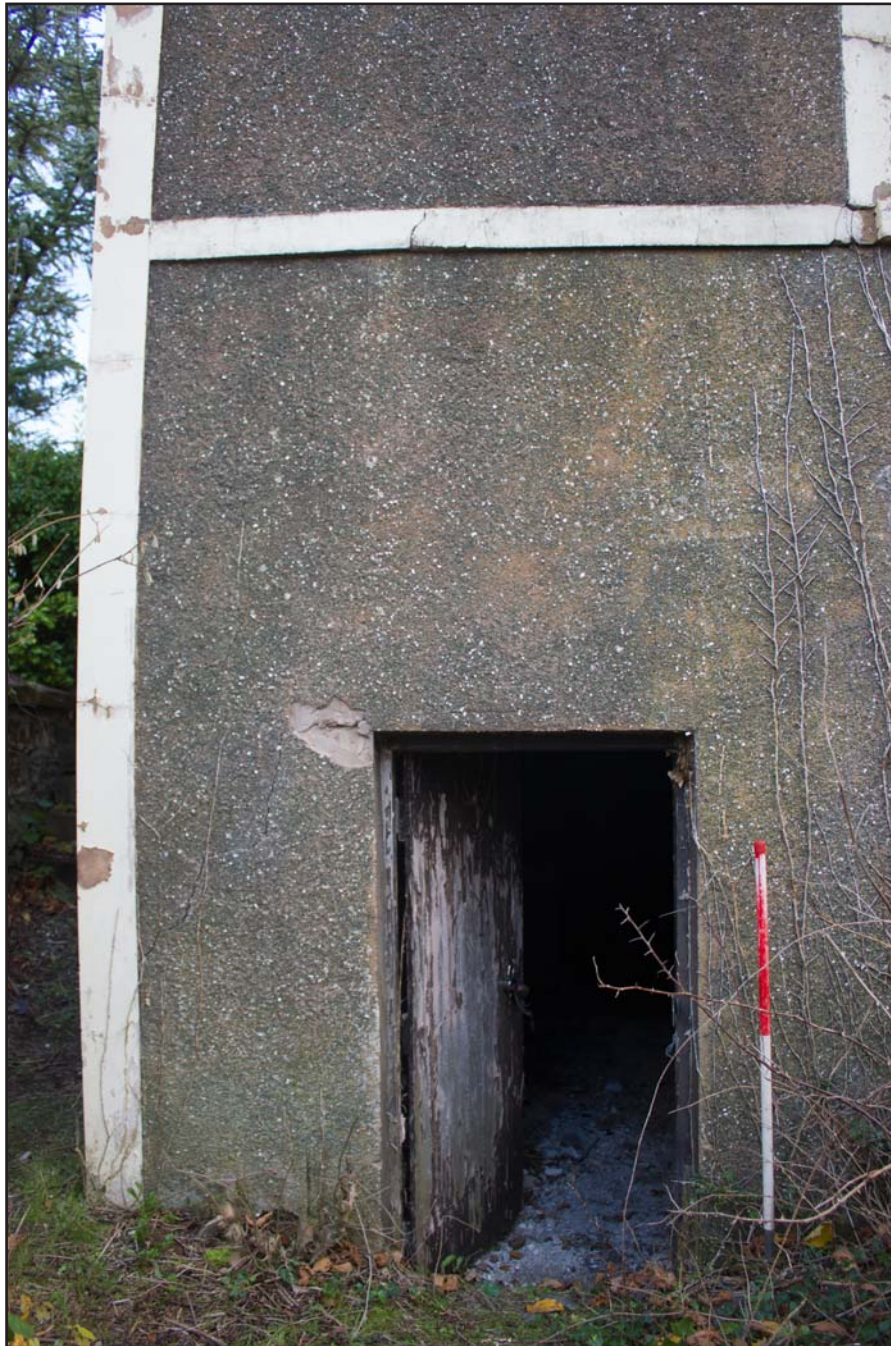
Plate 04: Door access to basement at left end of south western elevation, Tŷ Capel, Denbigh Road, Llanfairtalhaiarn, Conwy - from the southwest - 1.00m scale
