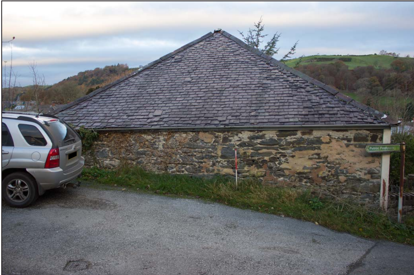
Plate 15: External shot of south eastern elevation, Tŷ Capel, Denbigh Road, Llanfairtalhaiarn, Conwy - from the southeast - 1.00m scale
