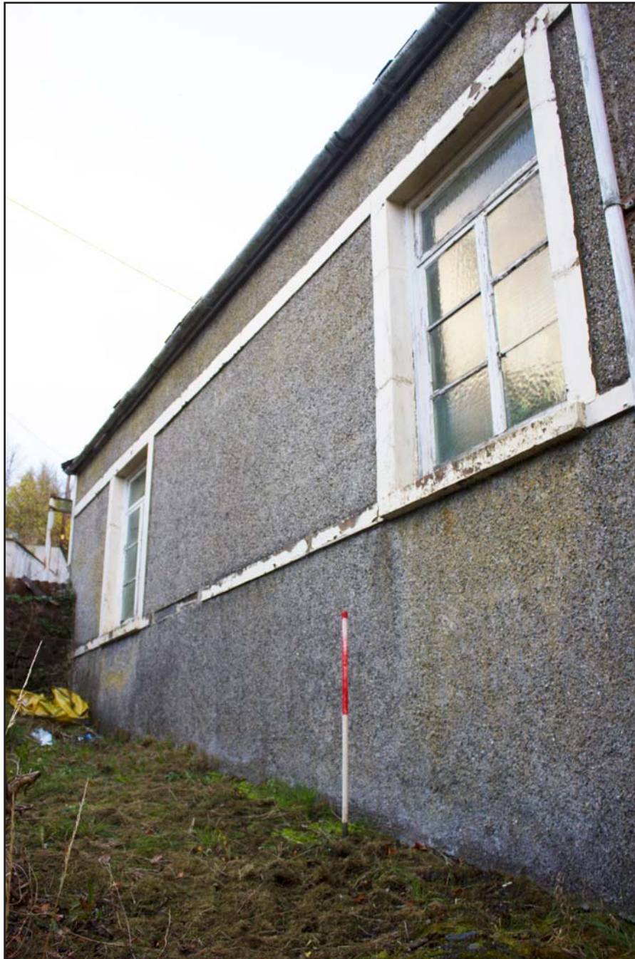
Plate 10: External oblique shot of north eastern elevation, Tŷ Capel, Denbigh Road, Llanfairtalhaiarn, Conwy - from the north - 1.00m scale
