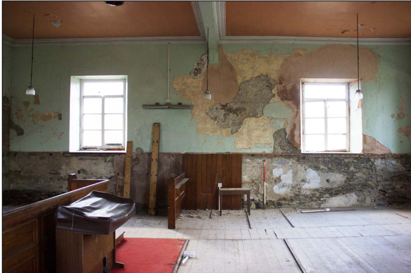
Plate 27: Internal shot south western elevation, Tŷ Capel, Denbigh Road, Llanfairtalhaiarn, Conwy - from the northeast - 1.00m scale
