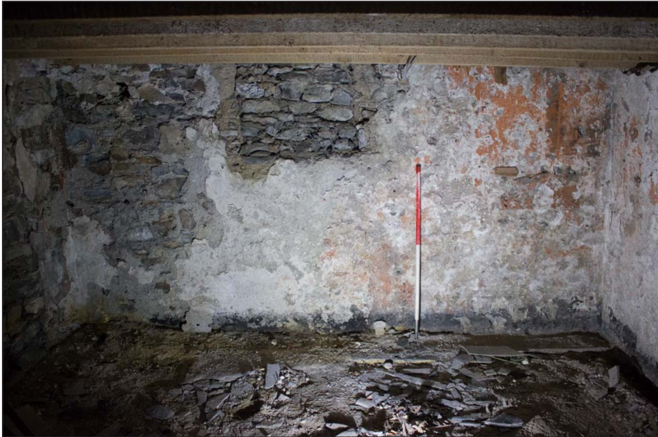
Plate 38: North eastern elevation within basement , Tŷ Capel, Denbigh Road, Llanfairtalhaiarn, Conwy - from the southwest - 1.00m scale
