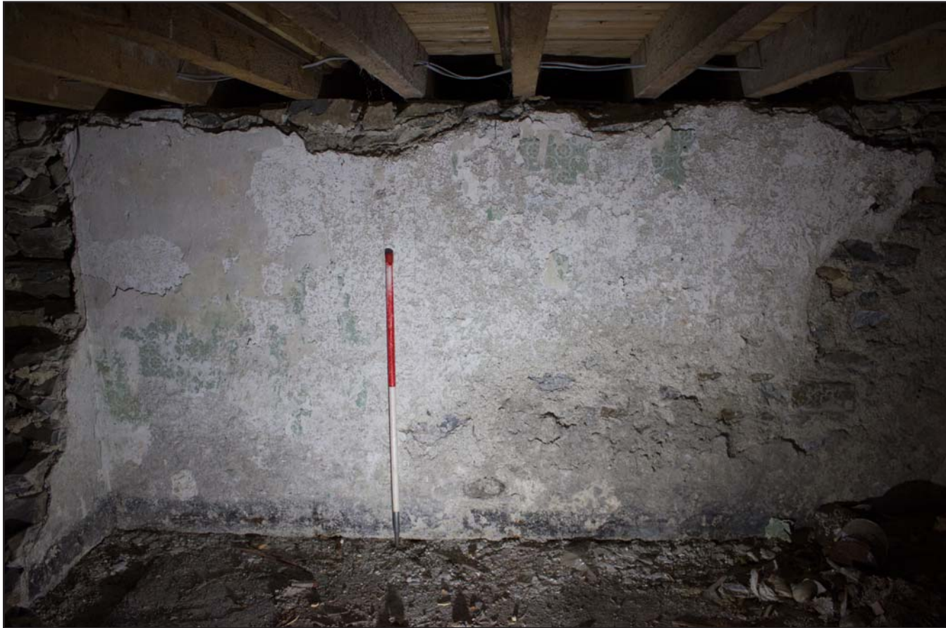
Plate 41: South eastern elevation (right) within basement , Tŷ Capel, Denbigh Road, Llanfairtalhaiarn, Conwy - from the northwest - 1.00m scale
