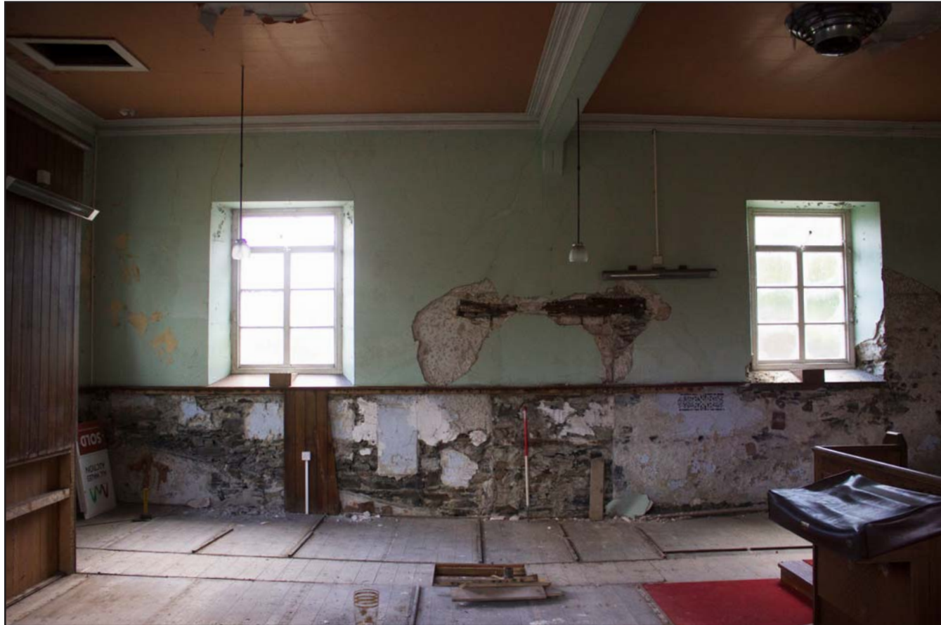
Plate 19: Internal shot of northeast elevation within Chapel, Tŷ Capel, Denbigh Road, Llanfairtalhaiarn, Conwy - from the southeast - 1.00m scale
