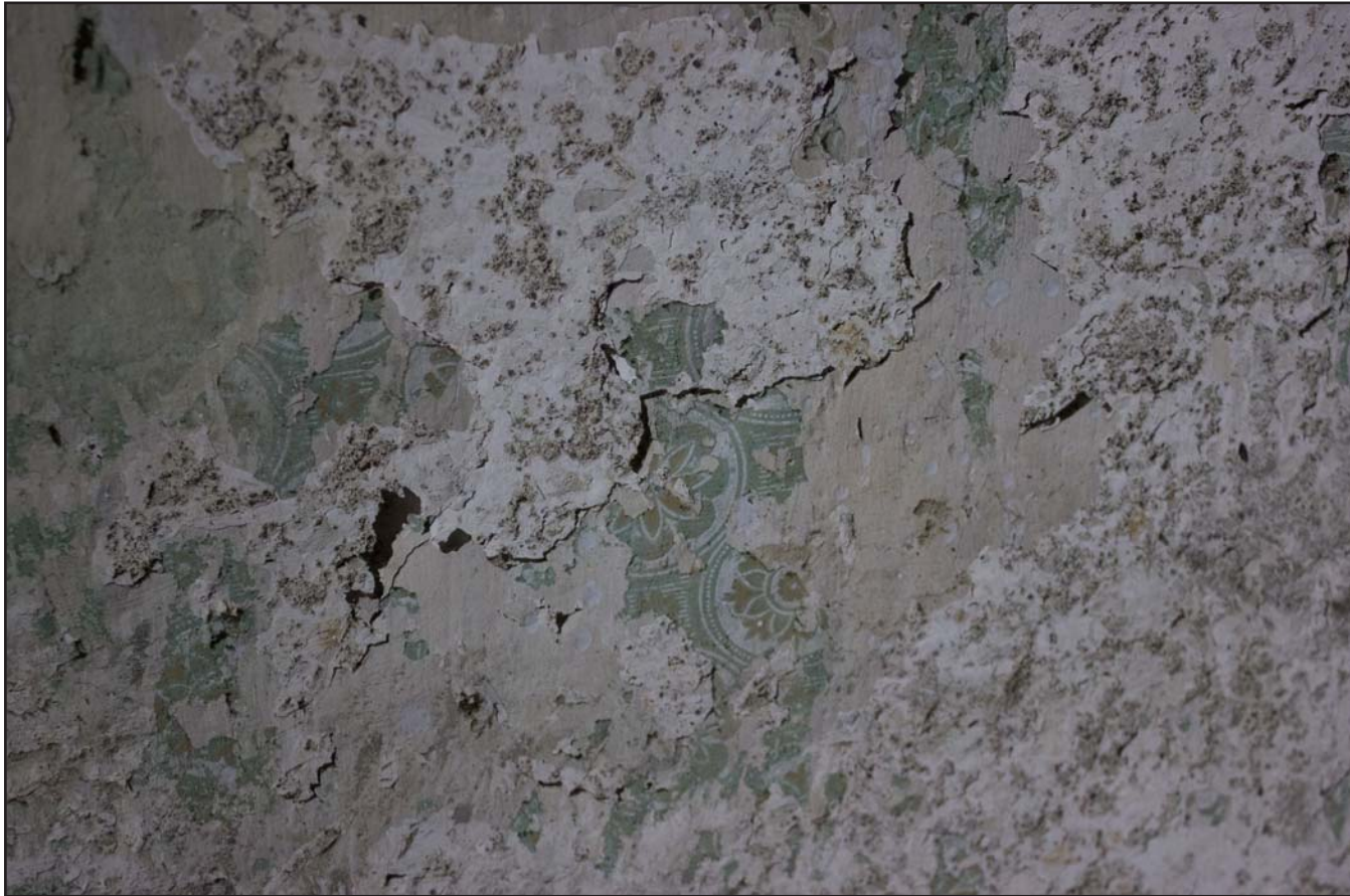
Plate 42: Example of wall paper on southeast elevation , Tŷ Capel, Denbigh Road, Llanfairtalhaiarn, Conwy - from the northwest - 1.00m scale
