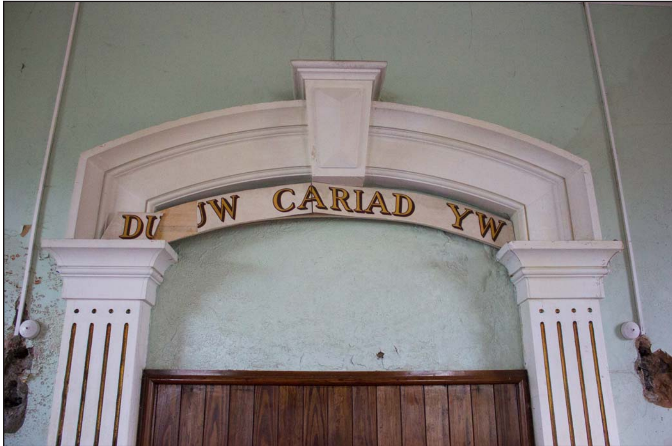
Plate 26: Painted banner above pulpit "DUW CARIAD YW", Tŷ Capel, Denbigh Road, Llanfairtalhaiarn, Conwy - from the northwest - no scale
