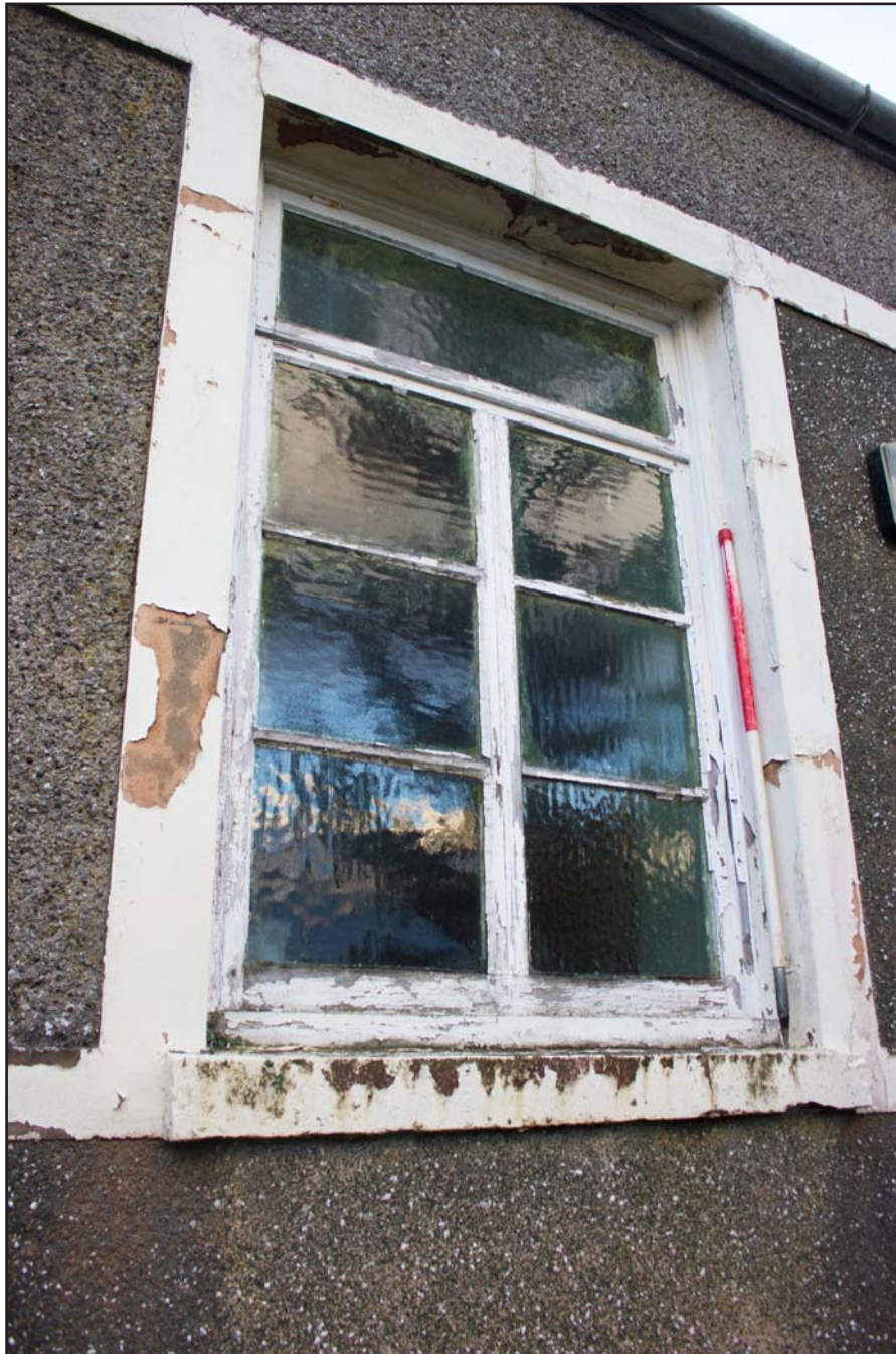
Plate 08: Window on north western elevation, Tŷ Capel, Denbigh Road, Llanfairtalhaiarn, Conwy - from the northwest - 1.00m
