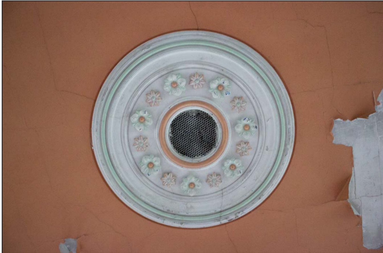
Plate 35: Internal shot of southern ceiling rose, Tŷ Capel, Denbigh Road, Llanfairtalhaiarn, Conwy - from the southeast - no scale
