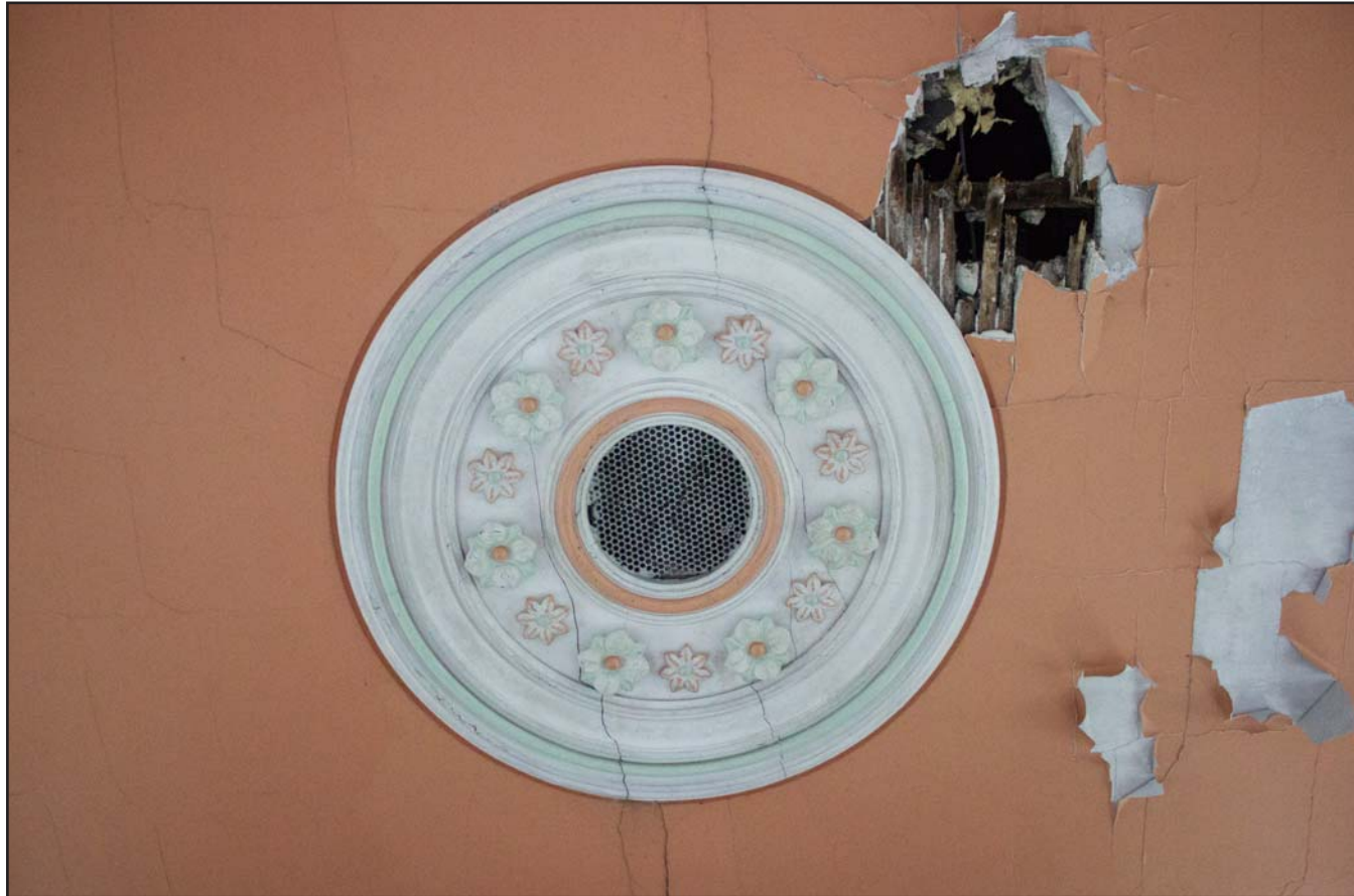
Plate 37: Internal shot of southern ceiling rose, Tŷ Capel, Denbigh Road, Llanfairtalhaiarn, Conwy - from the southeast - no scale
