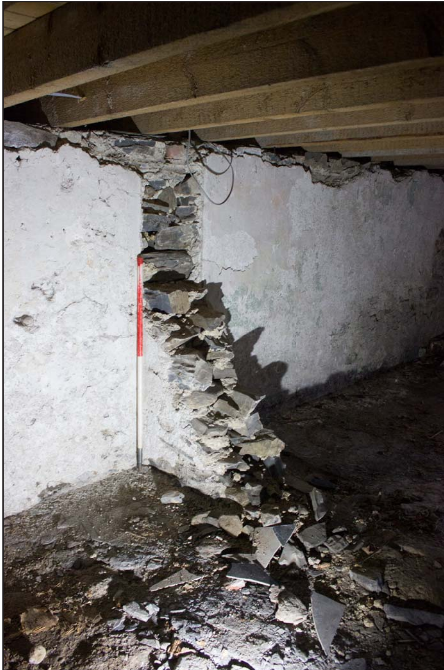
Plate 48: Former partition wall remains on the south eastern elevation within basement , Tŷ Capel, Denbigh Road, Llanfairtalhaiarn, Conwy - from the north - 1.00m scale
