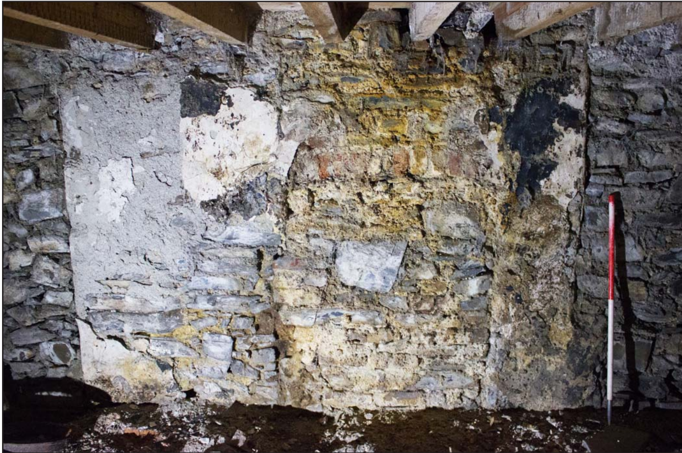
Plate 46: Former fireplace on the south eastern elevation within basement , Tŷ Capel, Denbigh Road, Llanfairtalhaiarn, Conwy - from the southeast - 1.00m scale
