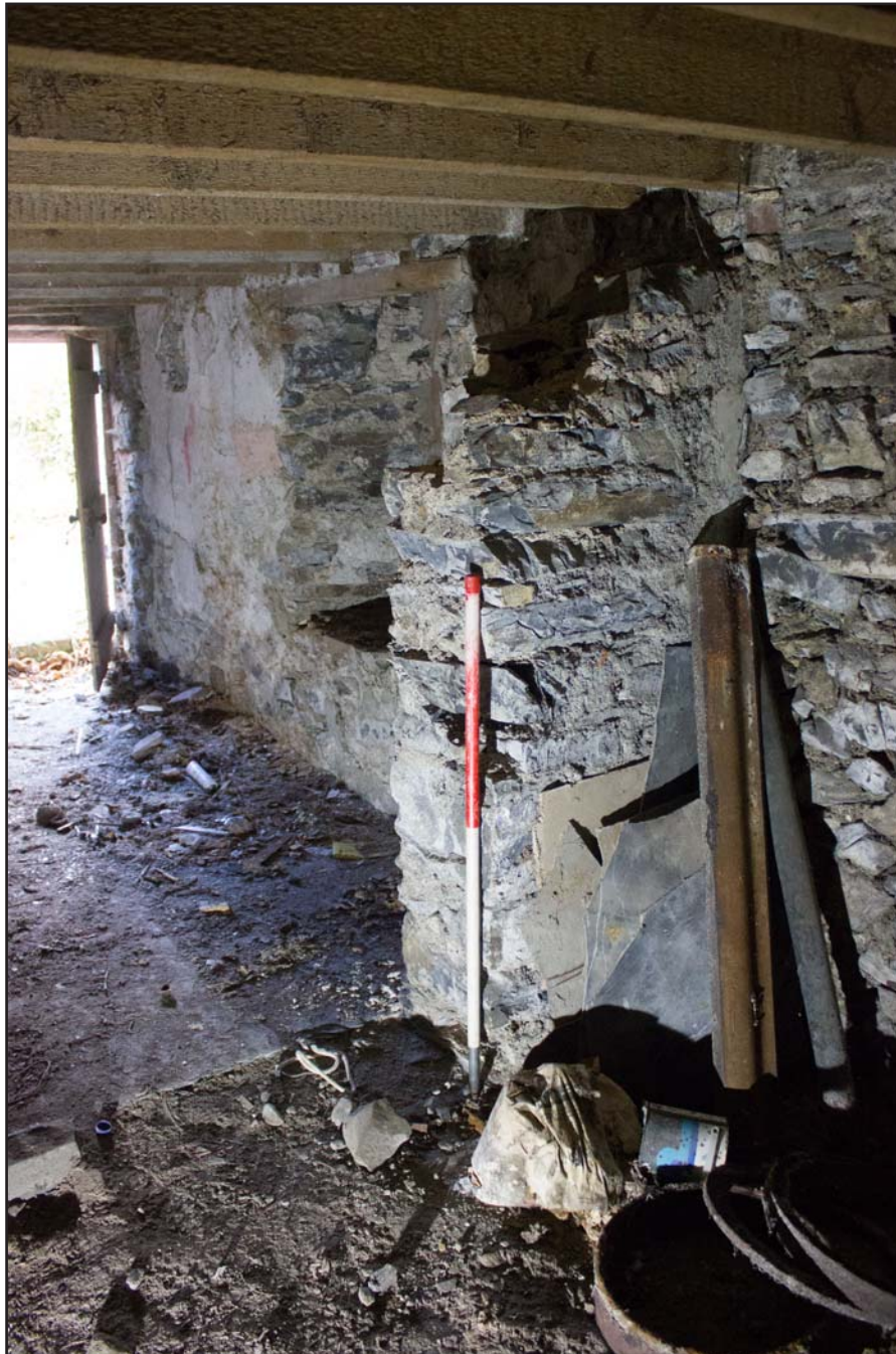
Plate 47: Former partition wall remains on the north western elevation within basement , Tŷ Capel, Denbigh Road, Llanfairtalhaiarn, Conwy - from the east - 1.00m scale
