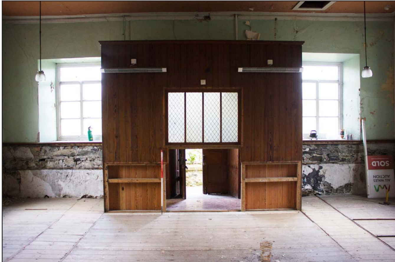
Plate 16: Internal shot Chapel entrance with wooden partition vestibule, Tŷ Capel, Denbigh Road, Llanfairtalhaiarn, Conwy - from the southeast - 1.00m scale
