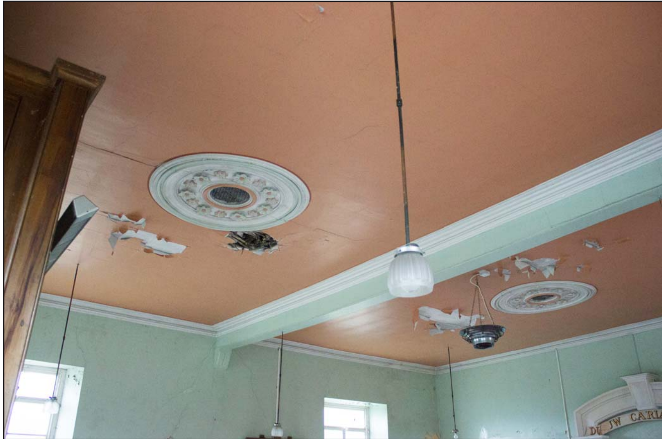
Plate 36: Internal shot of northern ceiling, Tŷ Capel, Denbigh Road, Llanfairtalhaiarn, Conwy - from the west - no scale
