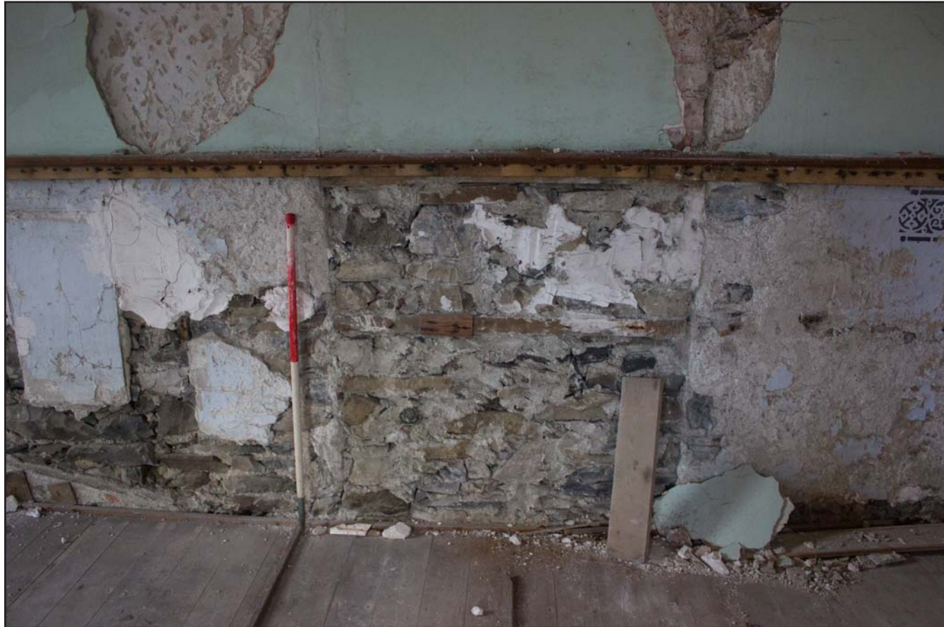
Plate 21: Internal shot, suspected former entranceway on north eastern elevation, Tŷ Capel, Denbigh Road, Llanfairtalhaiarn, Conwy - from the southwest - 1.00m scale
