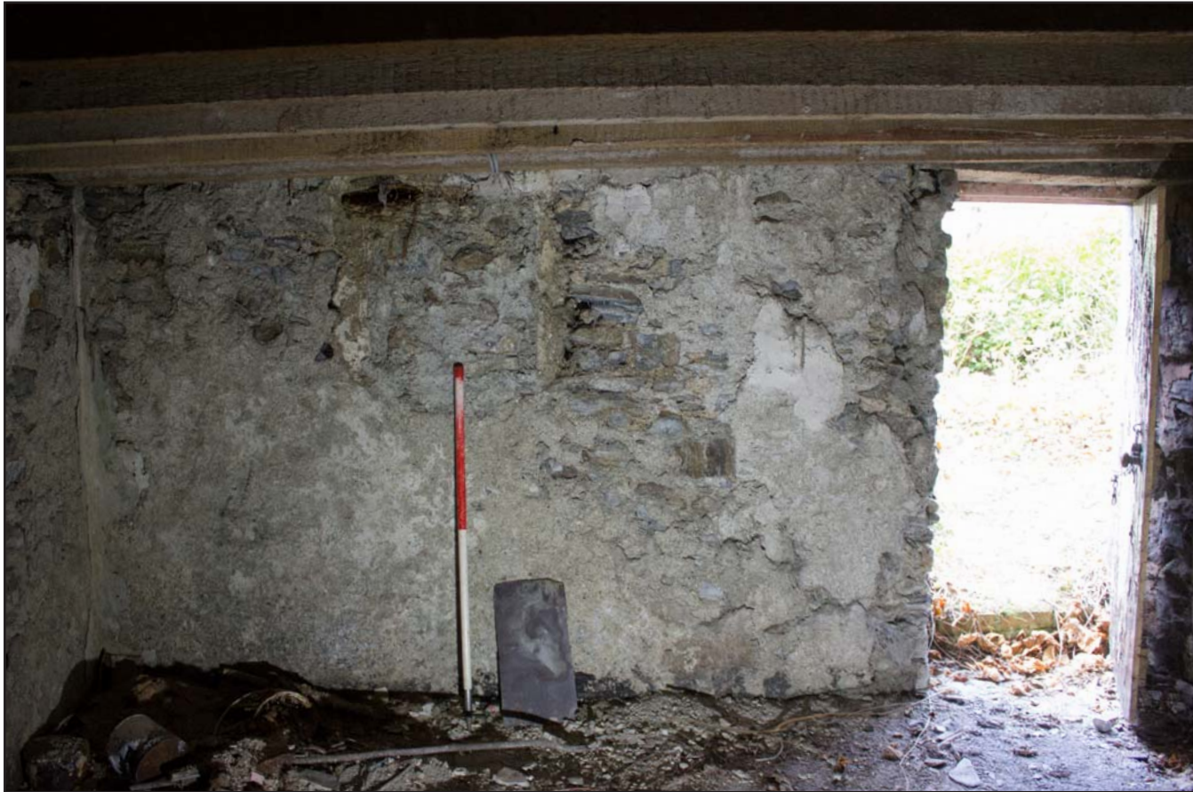
Plate 43: South western elevation within basement , Tŷ Capel, Denbigh Road, Llanfairtalhaiarn, Conwy - from the northeast - 1.00m scale
