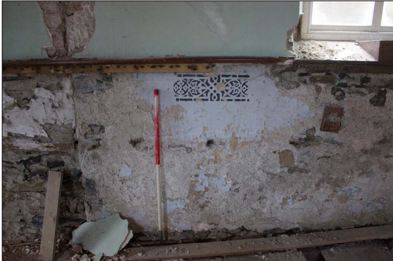
Plate 22: Internal shot, stencil visible below dado line on north eastern elevation, Tŷ Capel, Denbigh Road, Llanfairtalhaiarn, Conwy - from the southwest - 1.00m scale
