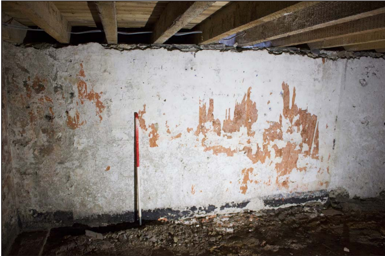
Plate 39: South eastern elevation (left) within basement , Tŷ Capel, Denbigh Road, Llanfairtalhaiarn, Conwy - from the northwest - 1.00m scale
