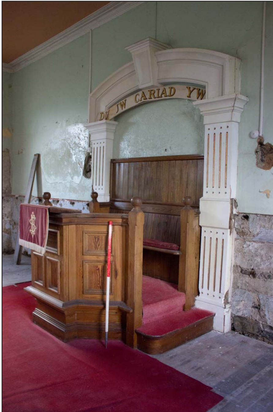
Plate 25: Oblique shot of pulpit on south eastern elevation, Tŷ Capel, Denbigh Road, Llanfairtalhaiarn, Conwy - from the west - 1.00m scale
