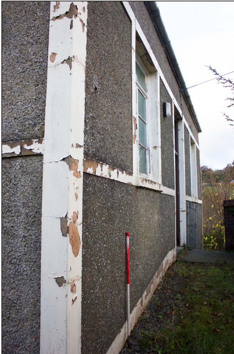
Plate 07: External oblique shot of north western elevation, Tŷ Capel, Denbigh Road, Llanfairtalhaiarn, Conwy - from the north - 1.00m scale
