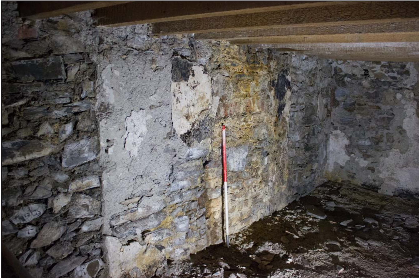
Plate 45: North western elevation (right) within basement , Tŷ Capel, Denbigh Road, Llanfairtalhaiarn, Conwy - from the south - 1.00m scale
