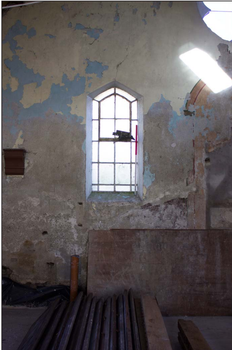
Plate 24: Example of internal view of window on northeast elevation within Bethesda Chapel, Back Chapel Street, Llanrhaeadr ym Mochnant - from the southwest - 1.00m scale
