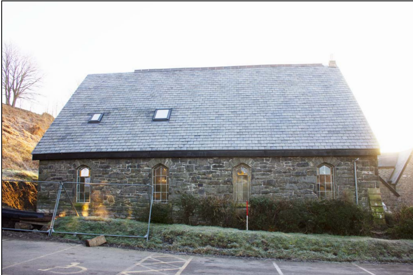
Plate 06: Northwest facing elevation of Bethesda Chapel, Back Chapel Street, Llanrhaeadr ym Mochnant - from the west/northwest - 1.00m scale
