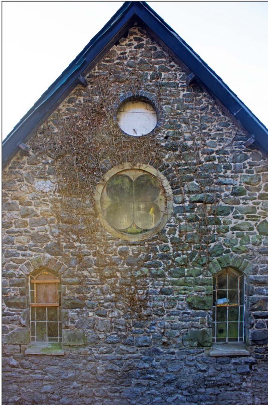
Plate 21: Window arrangement on northeast facing elevation of Bethesda Chapel, Back Chapel Street, Llanrhaeadr ym Mochnant - from the northeast - no scale
