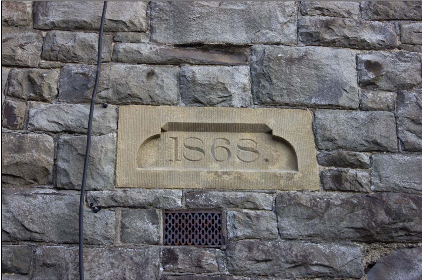
Plate 16: Date stone on southwest elevation of the Vestry extension at Bethesda Chapel, Back Chapel Street, Llanrhoadr ym Mochnant - from the southwest - no scale
