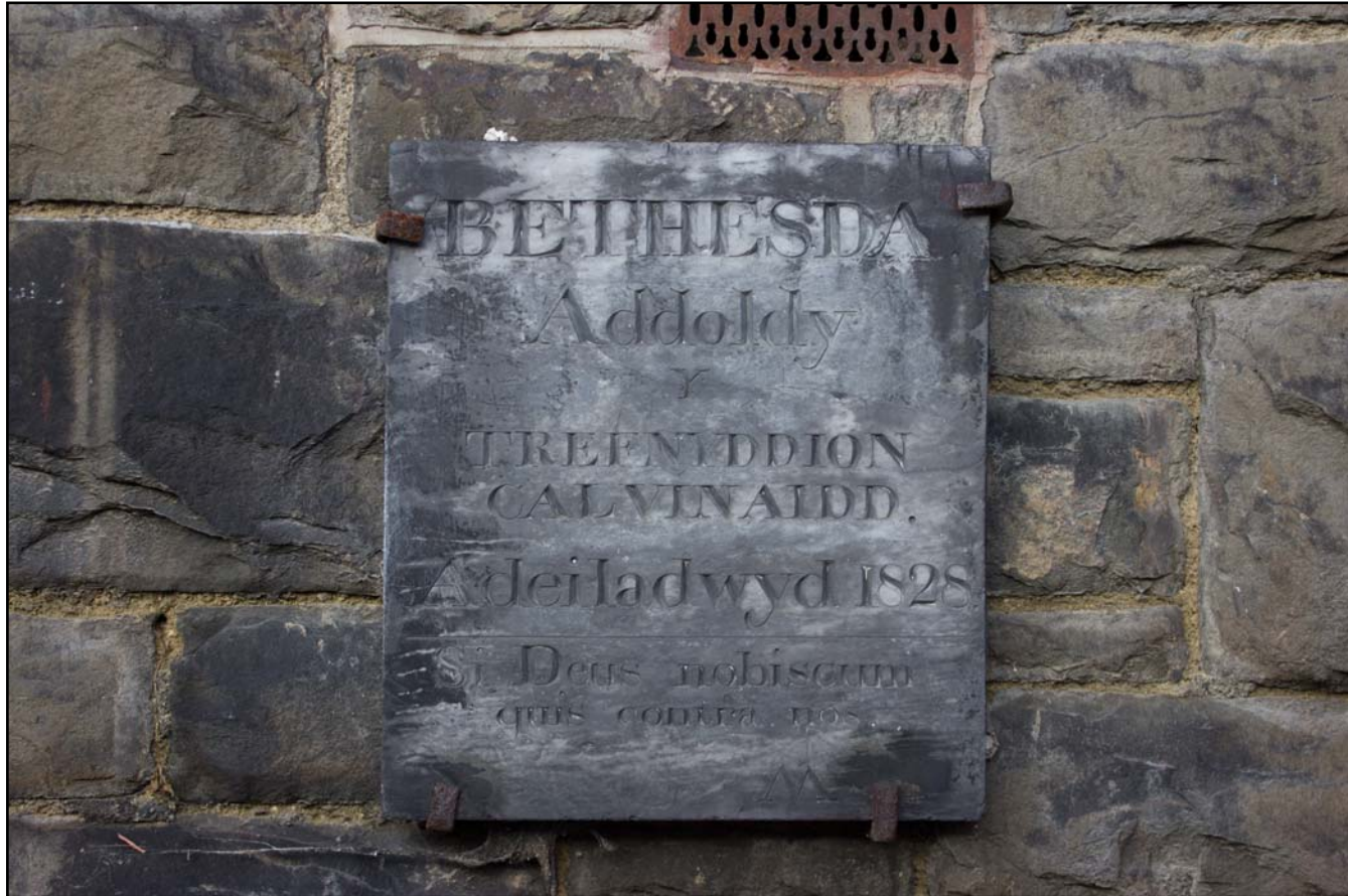
Plate 17: Slate inscribed plaque on southeast facing elevation of Bethesda Chapel, Back Chapel Street, Llanrhaeadr ym Mochnant - from the southeast - no scale
