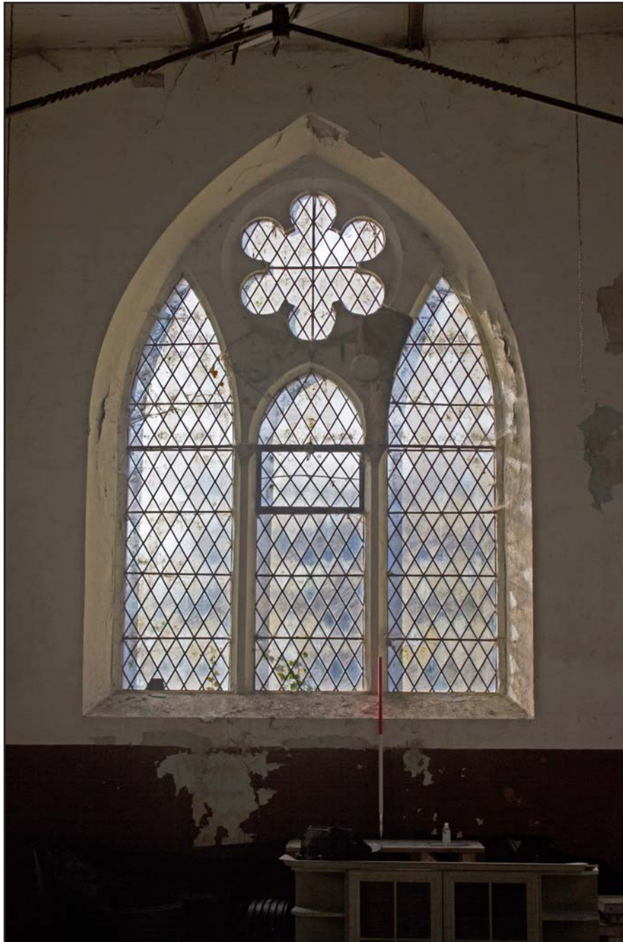
Plate 29: Internal view of main window within southwest (principal) elevation within Bethesda Chapel, Back Chapel Street, Llanrhaeadr ym Mochnant - from the northeast - 1.00m scale
