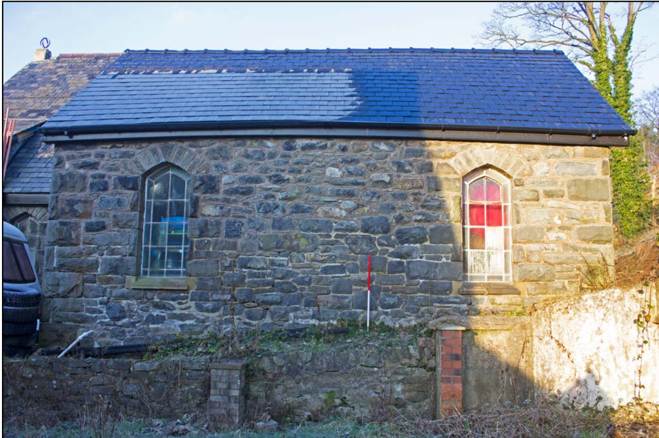
Plate 10: Southeast facing elevation of the Vestry at Bethesda Chapel, Back Chapel Street, Llanrhaeadr ym Mochnant - from the southeast - 1.00m scale
