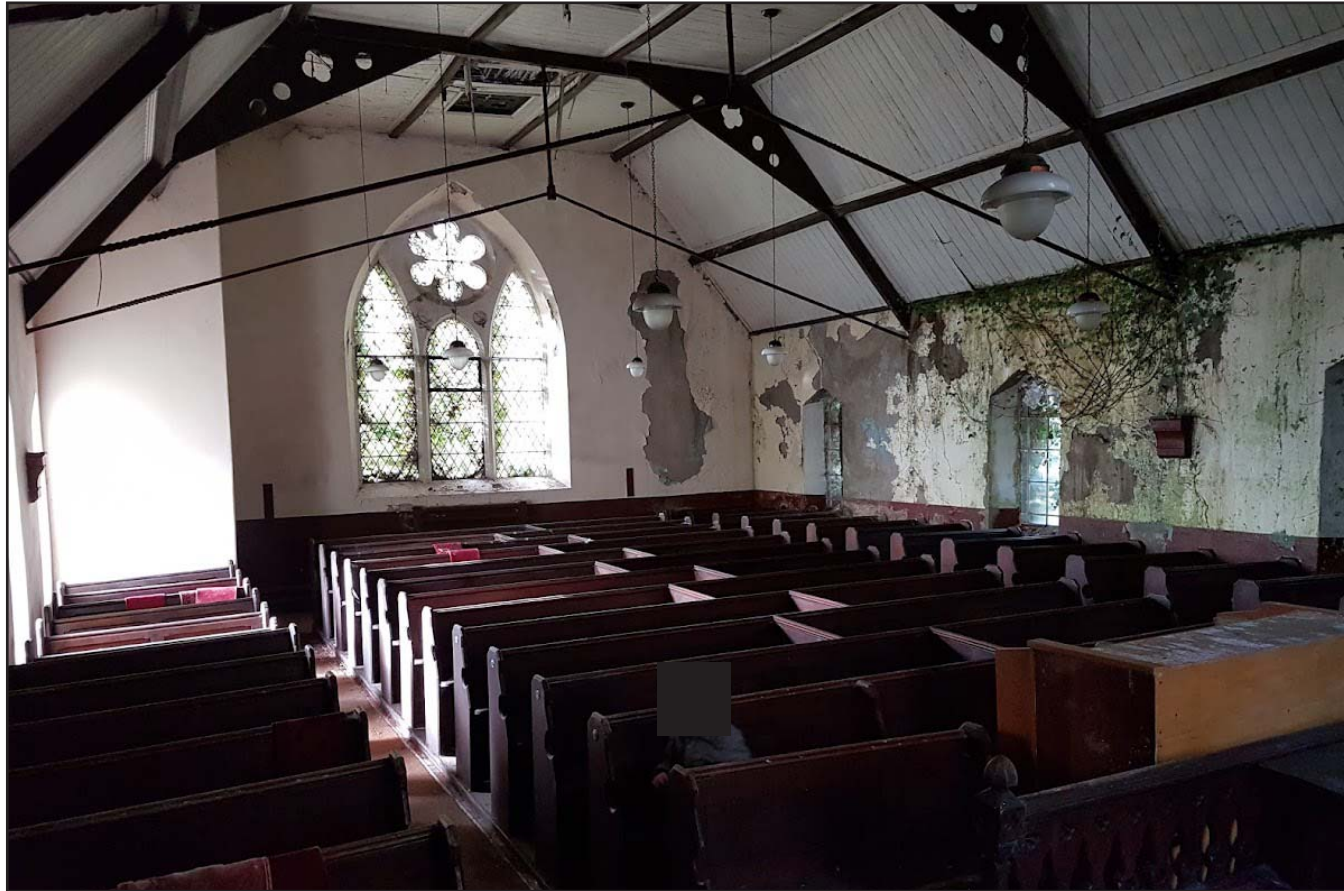
Plate C: View across chapel body showing the arrangement of pews - from the northeast.
