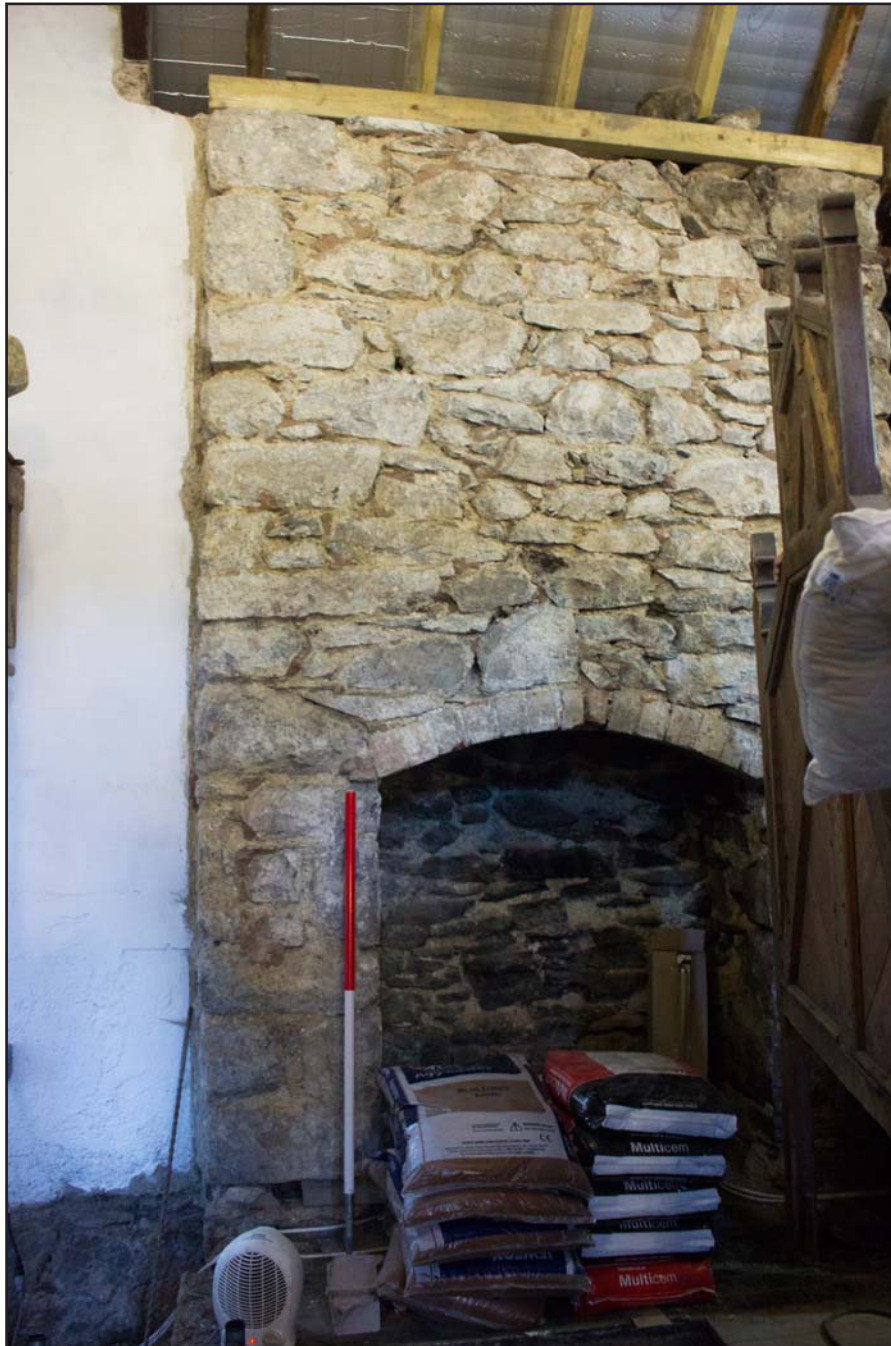
Plate 41: Fireplace within Vestry extension at Bethesda Chapel, Back Chapel Street, Llanrhaeadr ym Mochnant - from the northwest- 1.00m scale
