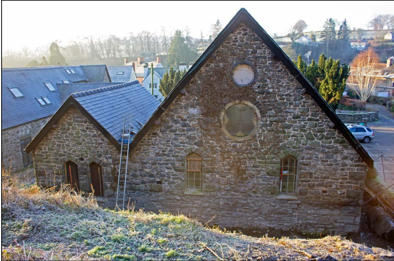
Plate 08: Northeast facing elevation of Bethesda Chapel, Back Chapel Street, Llanrhaeadr ym Mochnant - from the north/northeast - 1.00m scale
