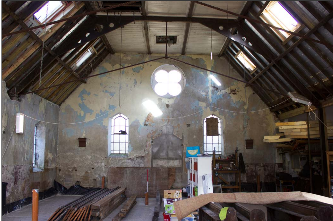
Plate 23: Internal shot across chapel body within Bethesda Chapel, Back Chapel Street, Llanrhaeadr ym Mochnant - from the southwest - 1.00m scale
