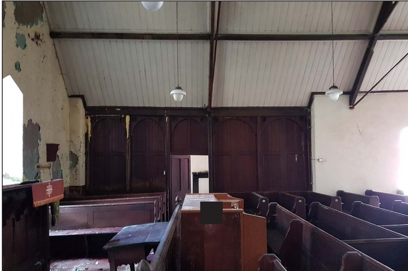
Plate E: View of (left end) south eastern elevation showing wooden screen and doorway to Vestry - from the northwest.
