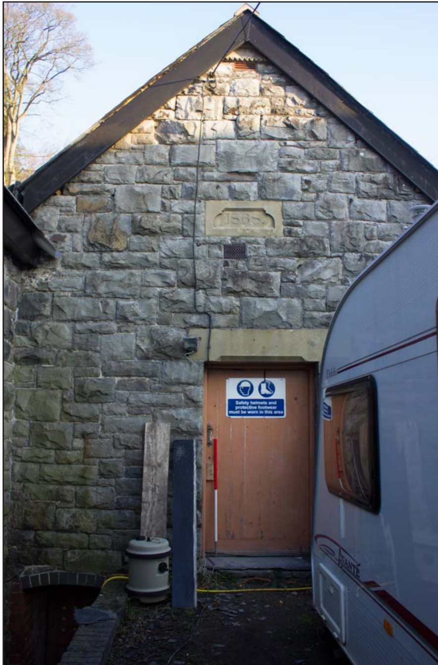
Plate 15: Southwest facing elevation of the Vestry at Bethesda Chapel, Back Chapel Street, Llanrhaeadr ym Mochnant - from the southwest - 1.00m scale
