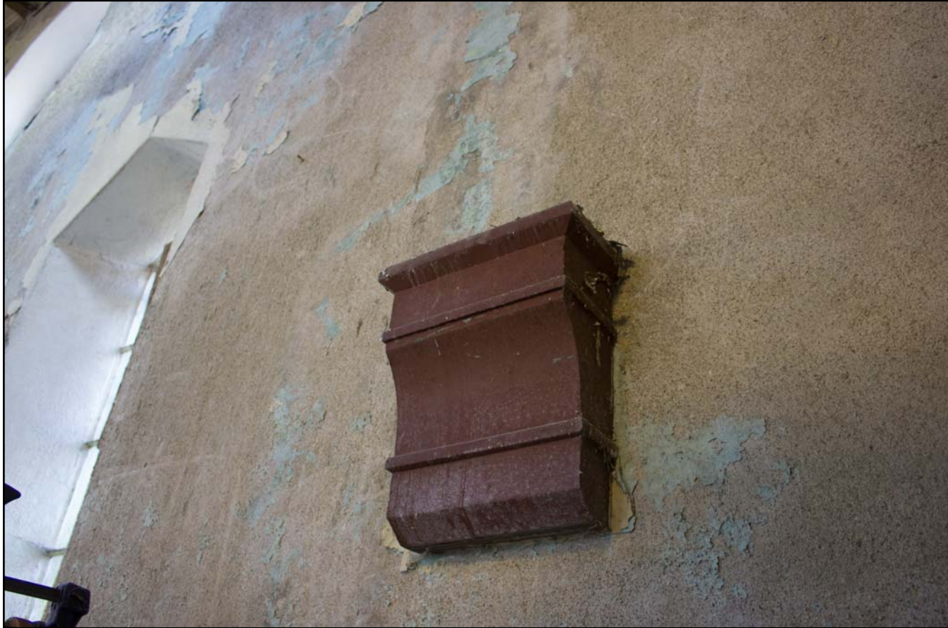
Plate 38: Decorative tin sconse ventilation brick cover within Bethesda Chapel, Back Chapel Street, Llanrhaeadr ym Mochnant - from the southeast - no scale
