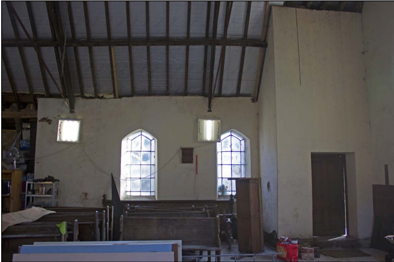
Plate 30: Internal shot of right side of southeast elevation within Bethesda Chapel, Back Chapel Street, Llanrhaeadr ym Mochnant - from the northwest - 1.00m scale
