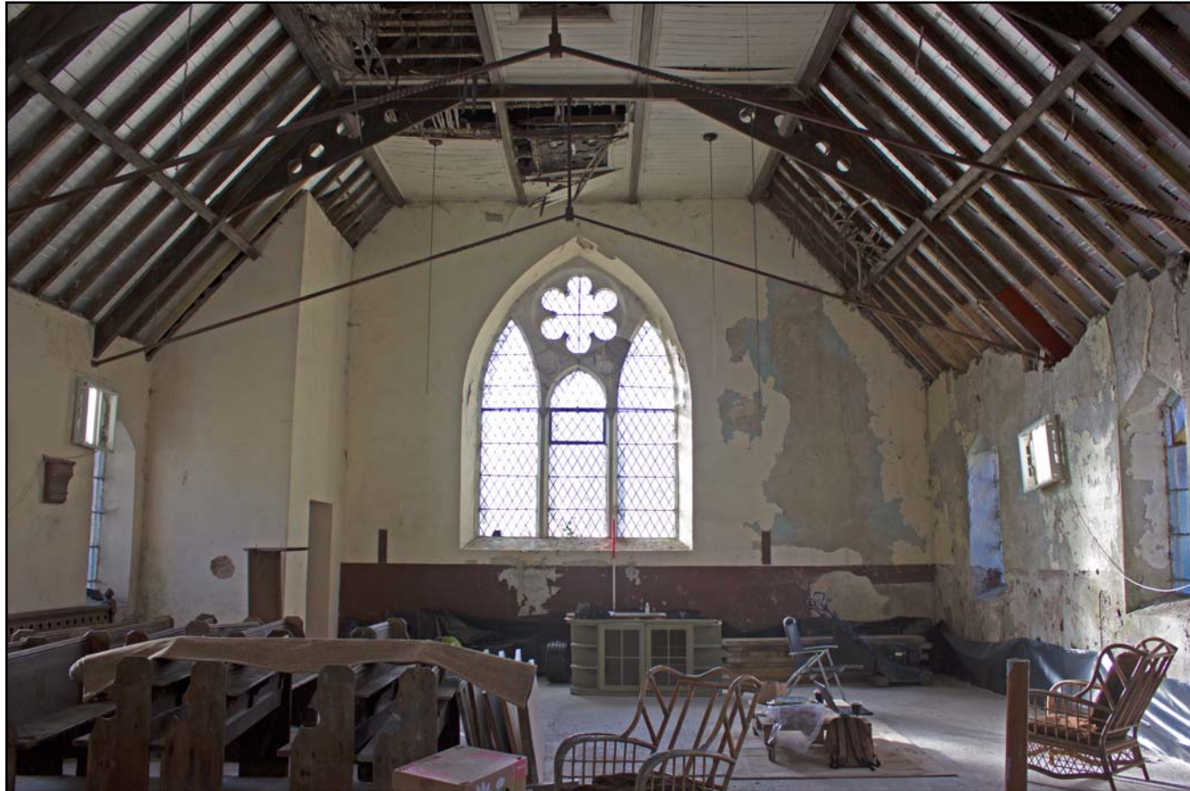
Plate 28: Internal shot across chapel body to Main Window within southwest elevation at Bethesda Chapel, Back Chapel Street, Llanrhaeadr ym Mochnant - from the southwest - 1.00m scale
