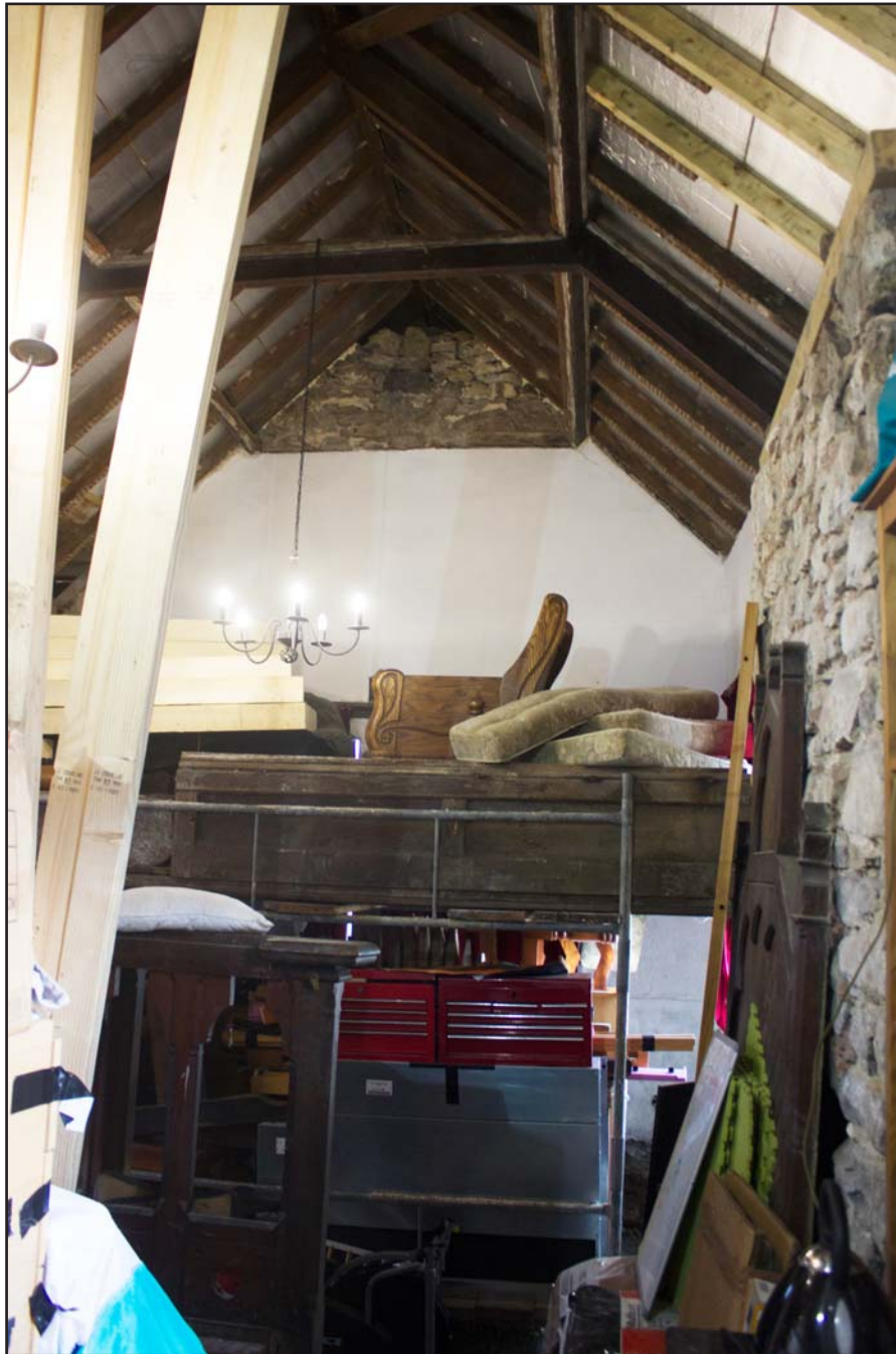
Plate 39: Internal shot of Vestry extension within Bethesda Chapel, Back Chapel Street, Llanrhaeadr ym Mochnant - from the southwest - no scale
