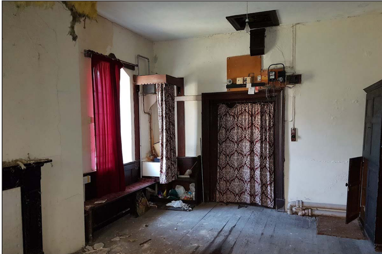
Plate F: View of the Vestry prior to removal of fixtures and fittings - from the north.
