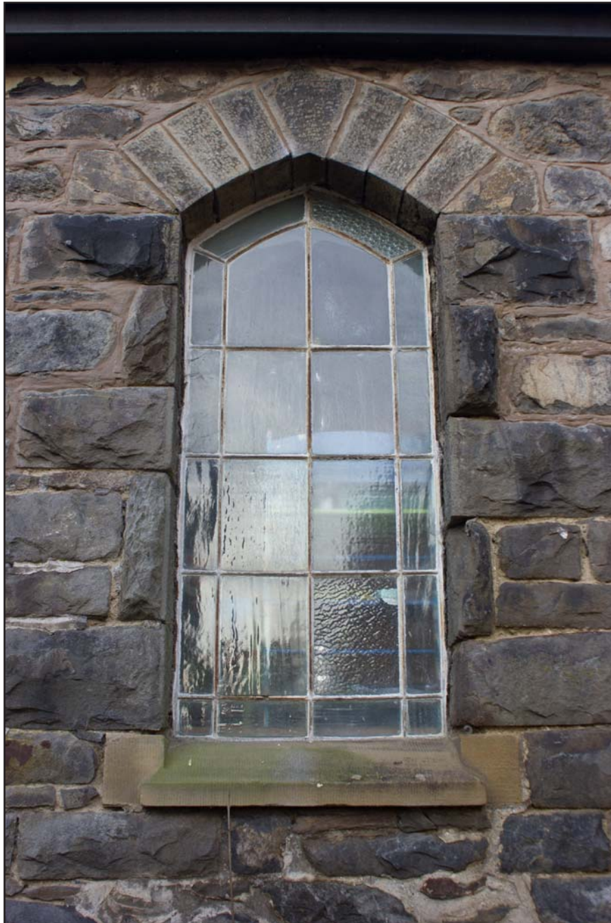
Plate 18: Example of window on southeast facing elevation of Bethesda Chapel, Back Chapel Street, Llanrhaeadr ym Mochnant - from the southeast - no scale
