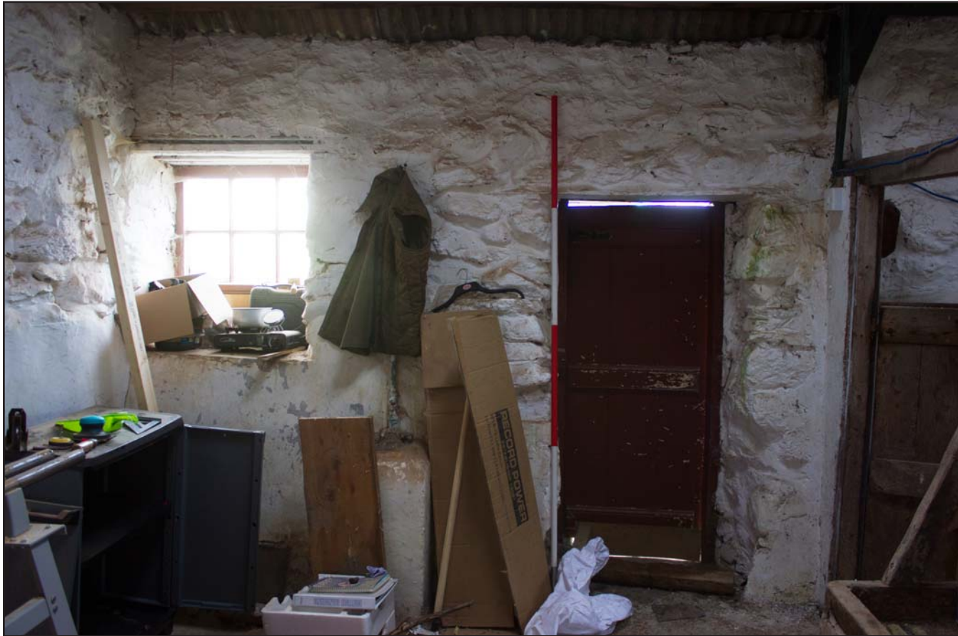
Plate 28: Manger in Room 1 within outbuilding at Penrhyn Garn, Rhydlydan, Pentrefeolas, Conwy - from the south - 2.00m scale
