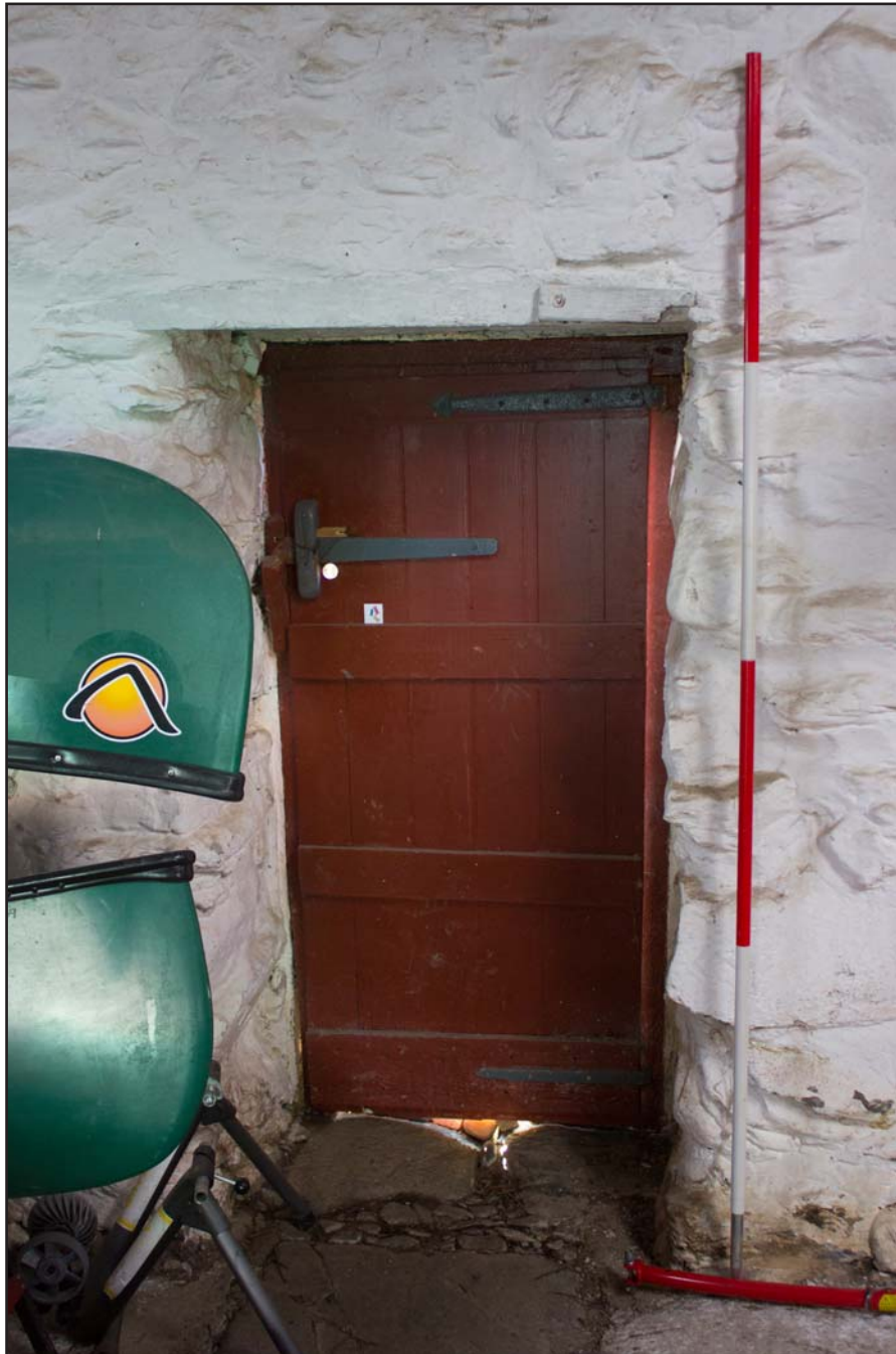
Plate 25: Example door in Room 1 within outbuilding at Penrhyn Garn, Rhydlydan, Pentrefeolas, Conwy - from the north - 2.00m scale
