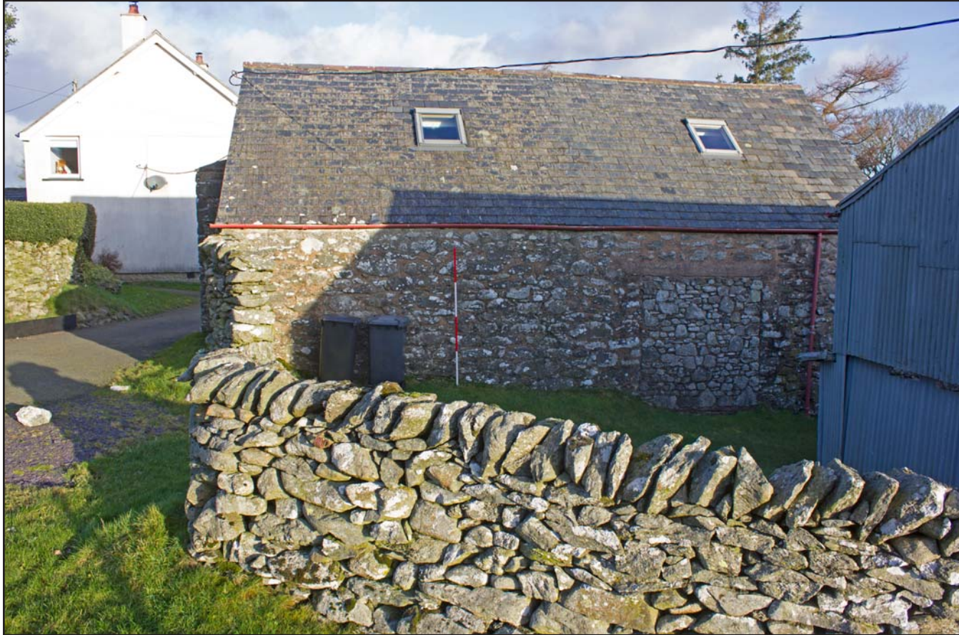
Plate 05: Southern elevation (left side) of outbuilding at Penrhyn Garn, Rhydlydan, Pentrefeolas, Conwy - from the south - 2.00m scale
