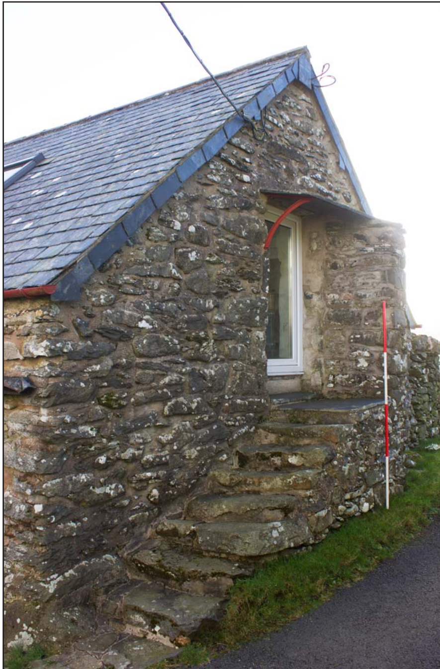
Plate 20: Western gable elevation (right) of outbuilding at Penrhyn Garn, Rhydlydan, Pentrefeolas, Conwy - from the west - 2.00m scale
