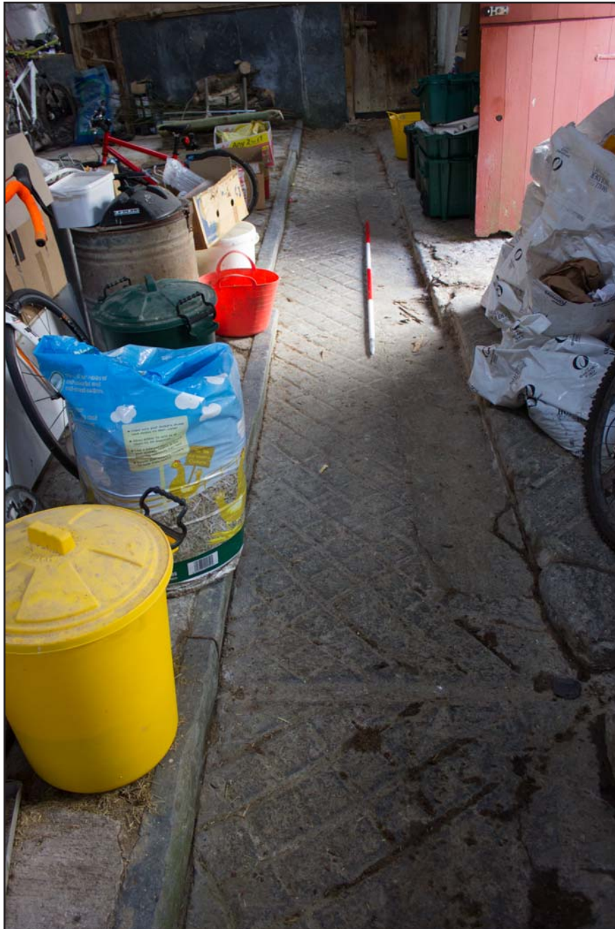
Plate 24: Slurry channel in Room 1 within outbuilding at Penrhyn Garn, Rhydlydan, Pentrefeolas, Conwy - from the east - 2.00m scale
