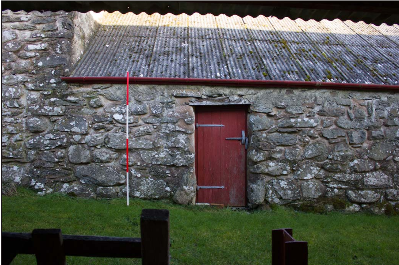
Plate 07: Southern elevation (centre left) of outbuilding at Penrhyn Garn, Rhydlydan, Pentrefeolas, Conwy - from the south - 2.00m scale
