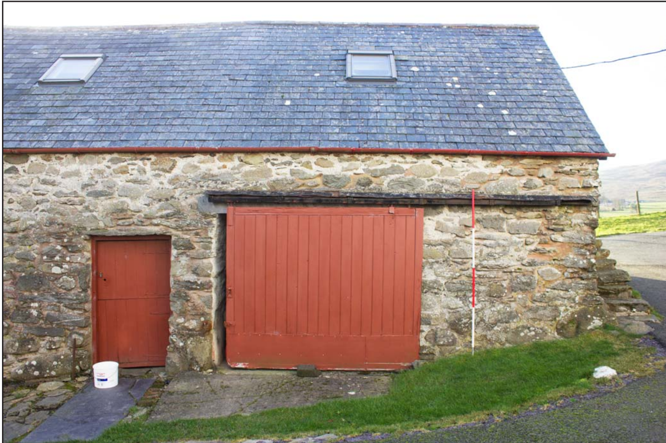
Plate 18: Northern elevation (right) of outbuilding at Penrhyn Garn, Rhydlydan, Pentrefeolas, Conwy - from the north - 2.00m scale
