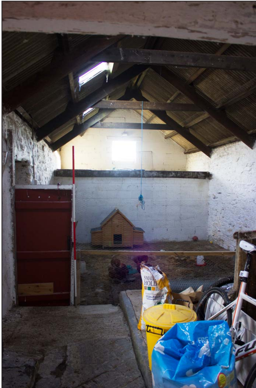
Plate 21: Eastern end of Room 1 within outbuilding at Penrhyn Garn, Rhydlydan, Pentrefeolas, Conwy - from the west - 2.00m scale
