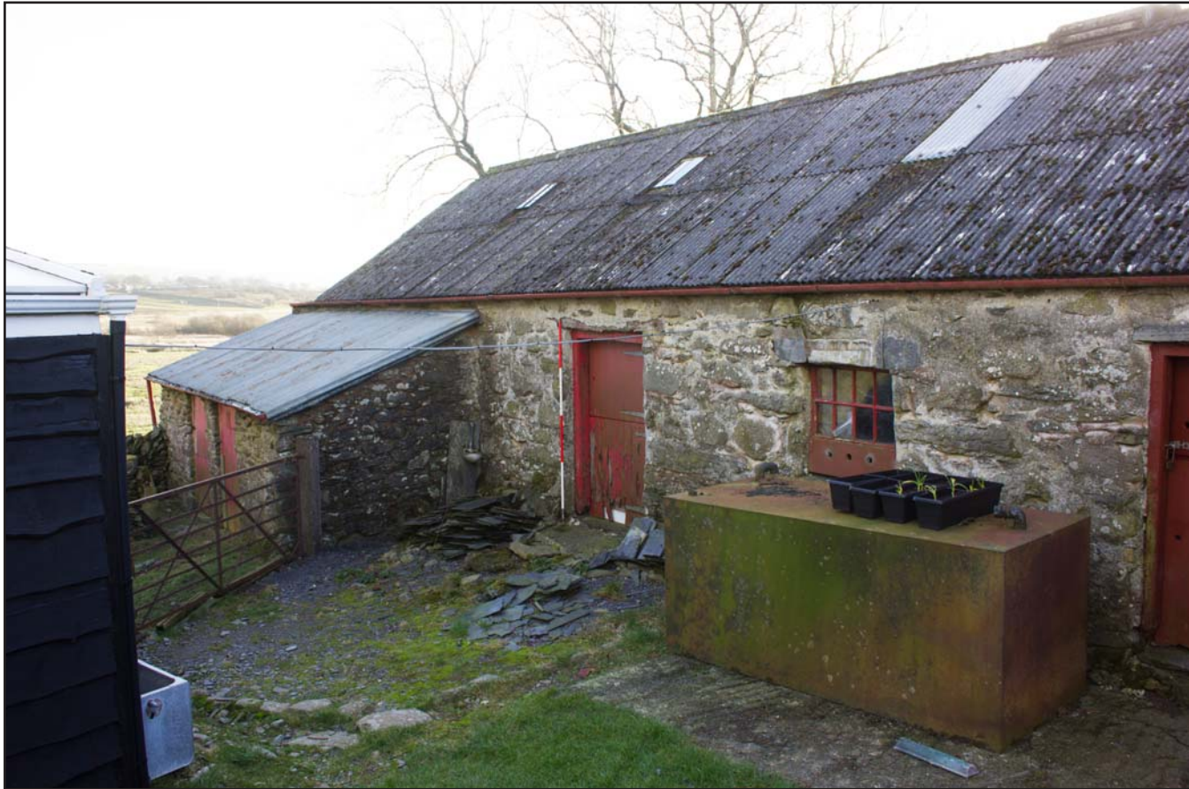
Plate 15: Northern elevation (left centre), oblique shot, of outbuilding at Penrhyn Garn, Rhydlydan, Pentrefeolas, Conwy - from the north - 2.00m scale
