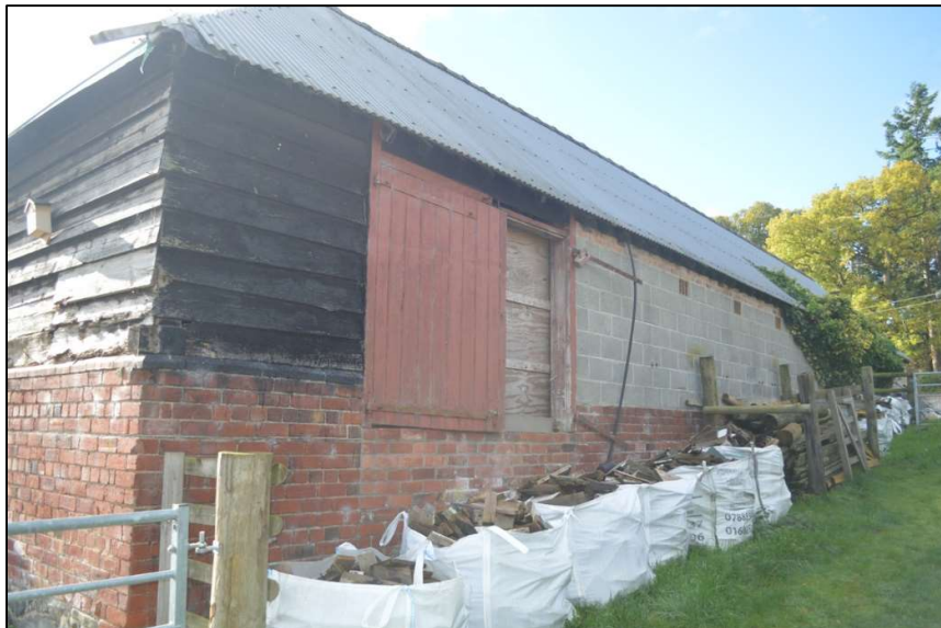
Fig. 8 View from the east looking along the north elevation of the north range Photo CPAT 5031_088
