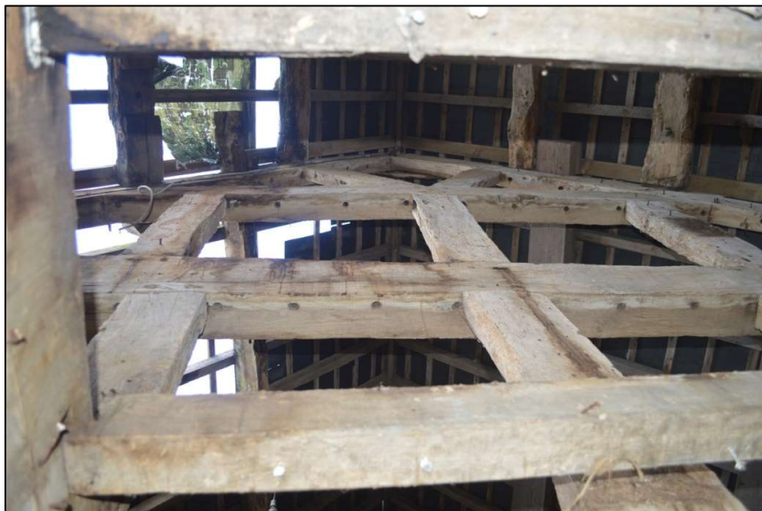
Fig. 15 Stave holes in one of the internal roof trusses Photo CPAT 5031_106
