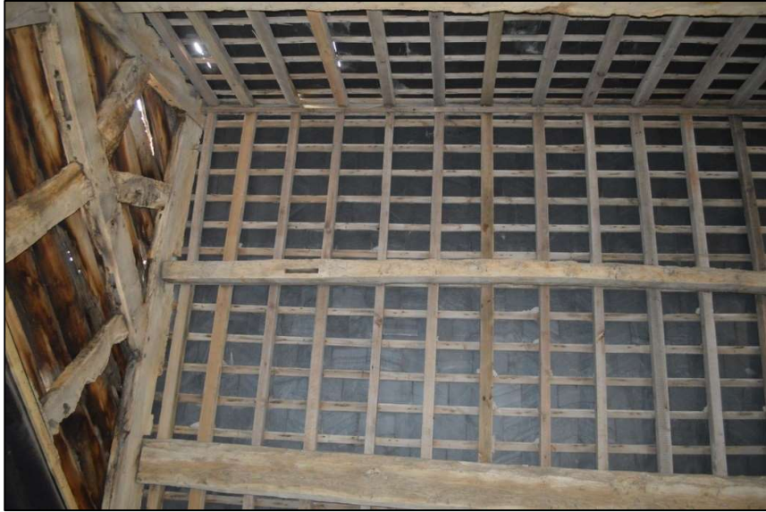
Fig. 14 Roof structure in the threshing barn (note reused wall timber in centre of shot) Photo CPAT 5031_097
