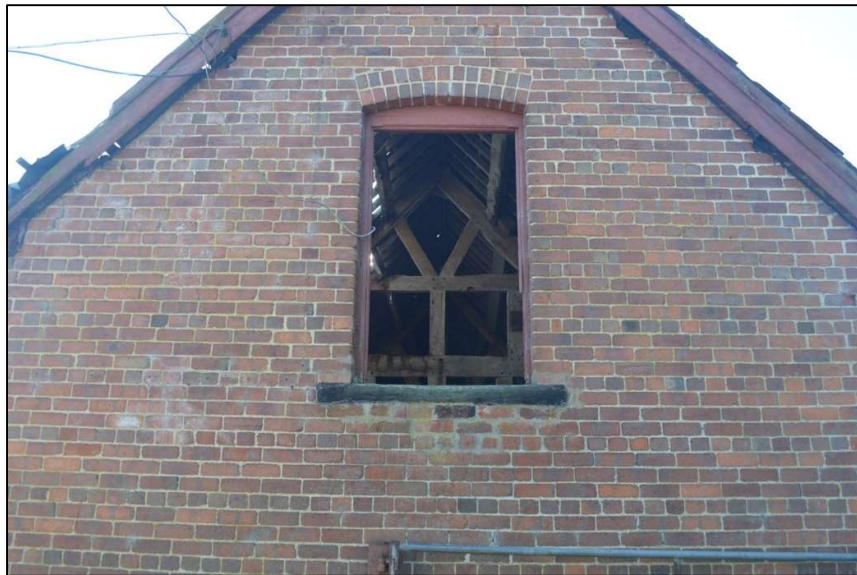
Fig. 13 High level doorway to the loft on the northern gable end of the west range Photo CPAT 5031_031
