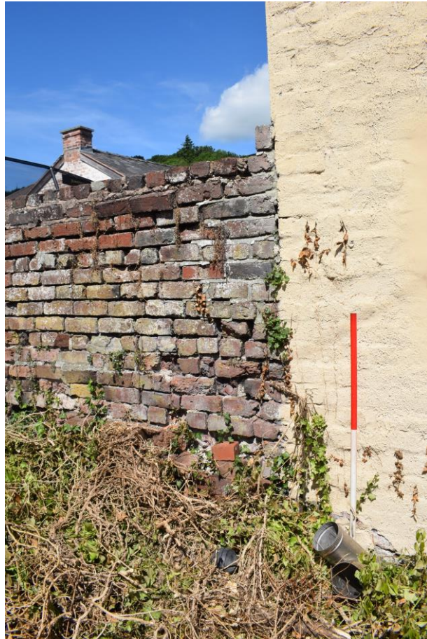
Fig. 7 Join between the Gable wall of Number 10 and the south-facing yard wall. CPAT Photograph 4998_20
