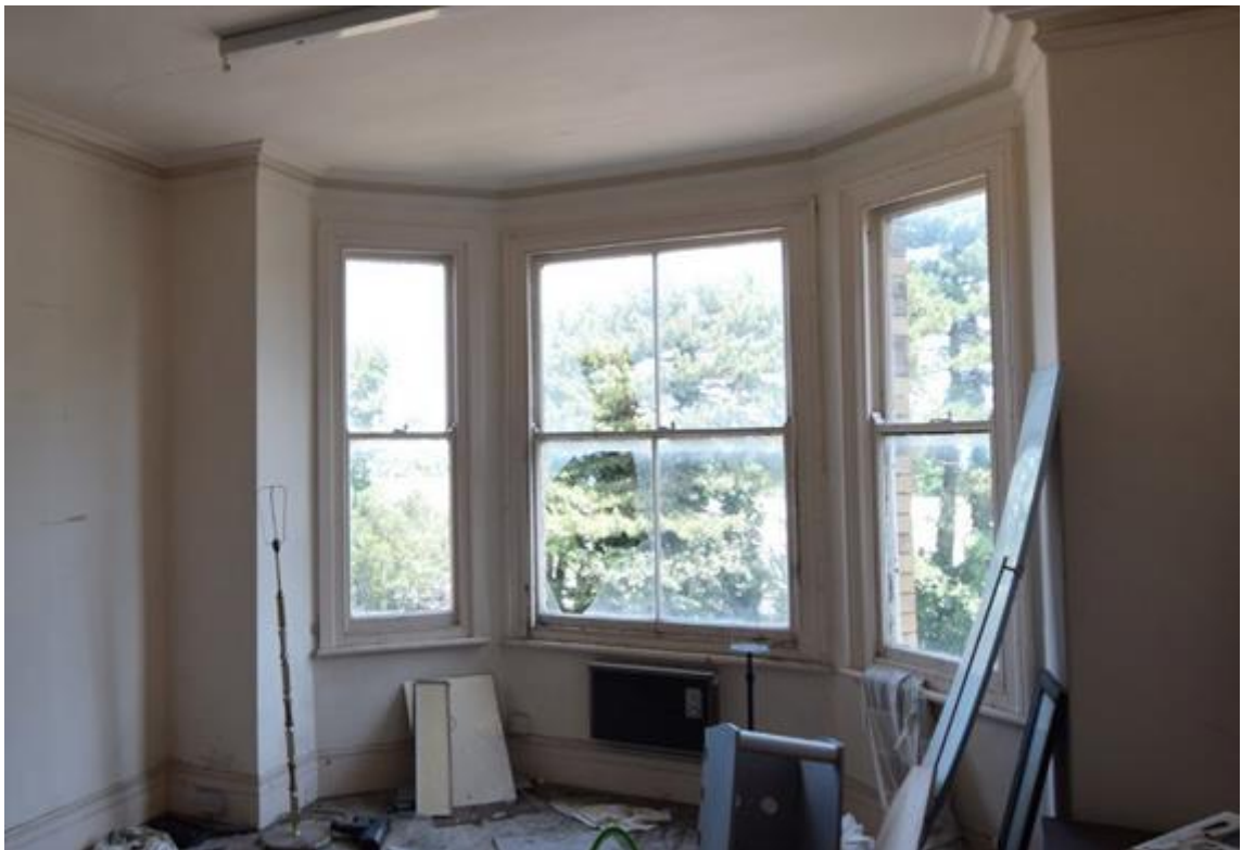
Fig. 12 1 st floor original sash windows and surviving coving and skirting board Photo CPAT 5077_101
