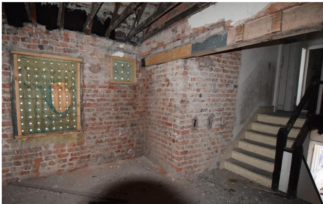
Fig 14 2 nd floor showing rafters and brick walls, with stairs to other floors CPAT 5077-155
