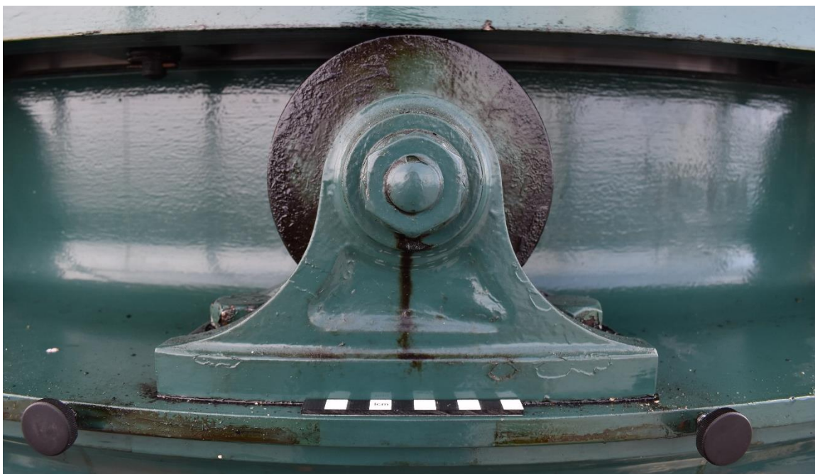
Figure 4.7: Detail of support wheel and bracket, scale is 10cm (© Crown Copyright: RCAHMW).
