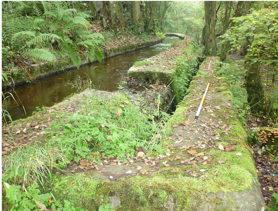
a. Overflow No. 1
