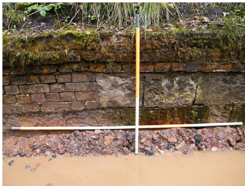
Fig. 30 Evidence of repairs to the leat
