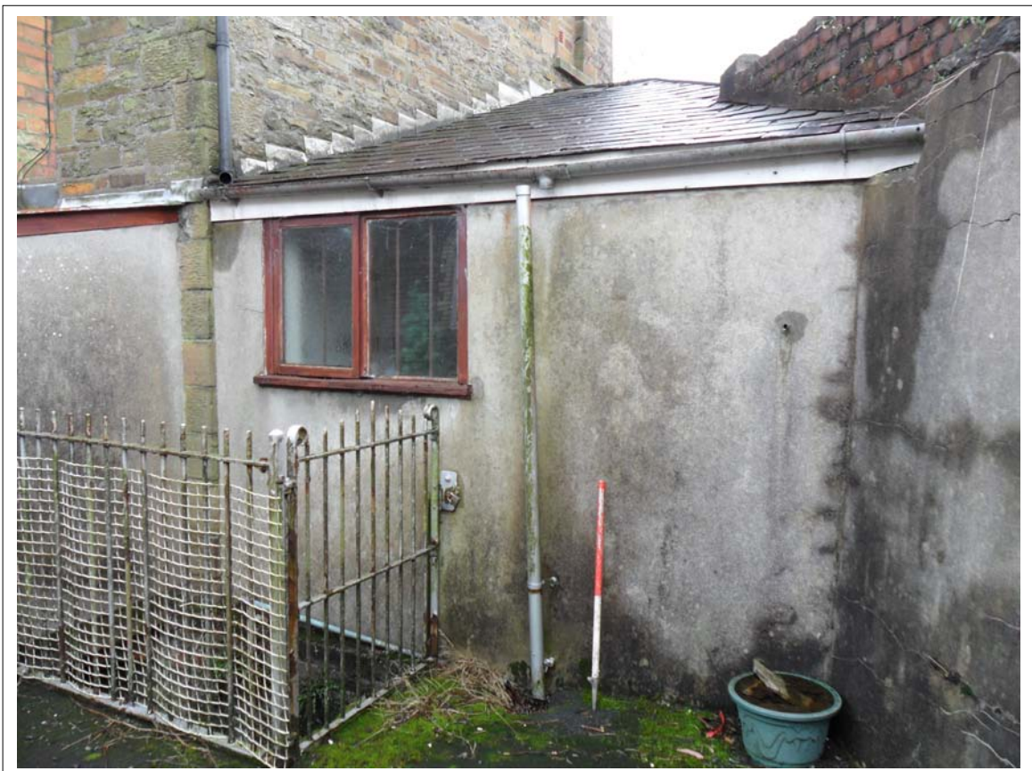
Plate 42:View of outside wall of Bathroom adjacent to access to Boiler tunnel
