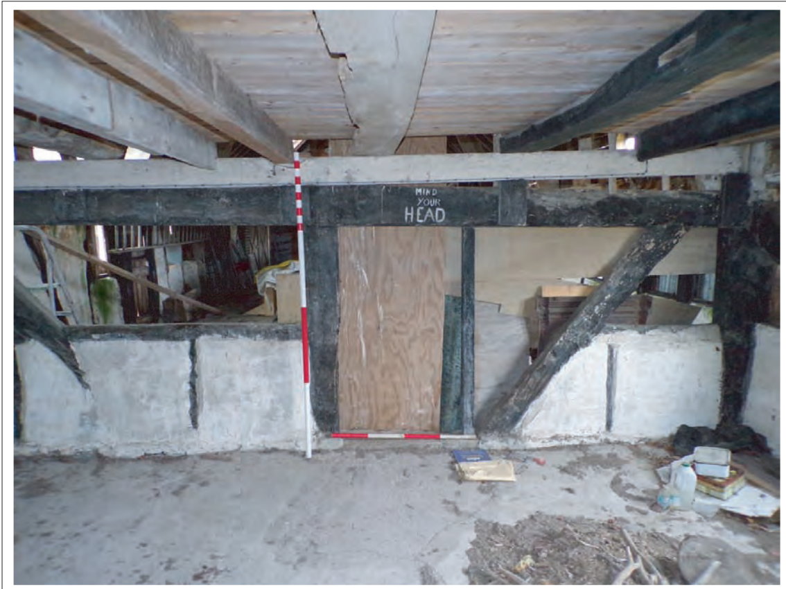
Plate 51: View of surviving 1772 partition and reused floor joists in loft above. Note poured concrete floor obscuring sill beam. Looking west, Scale 1x1m & 1x2m
