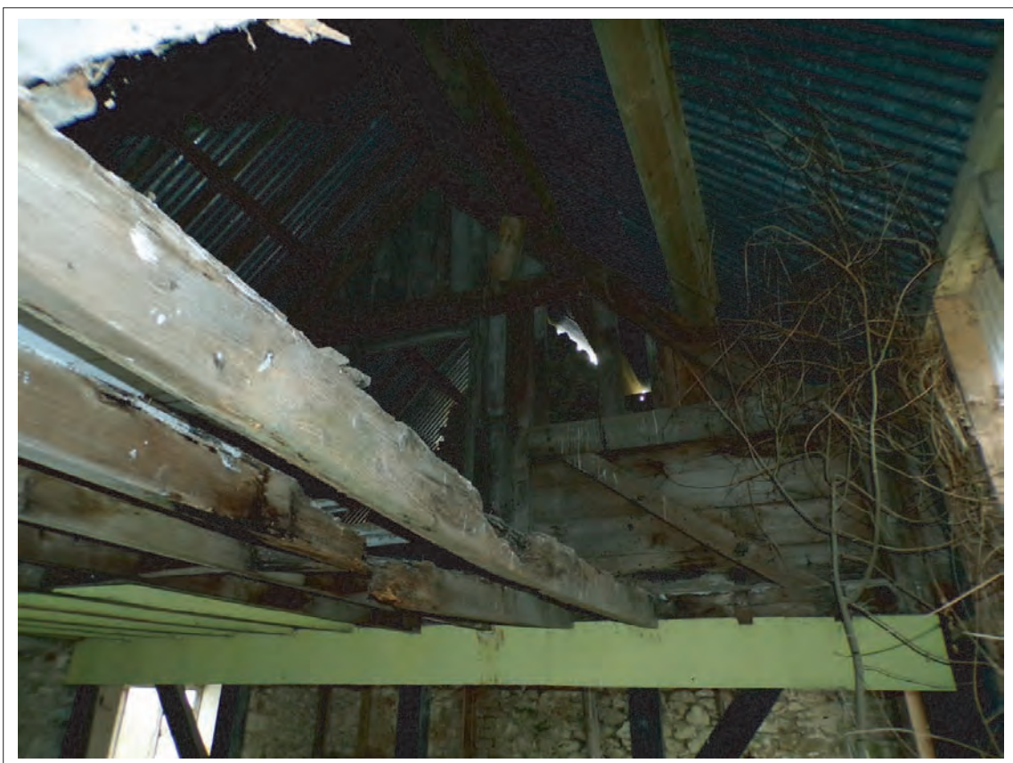
Plate 76: View of damaged loft flooring within eastern end of 1870s extension
