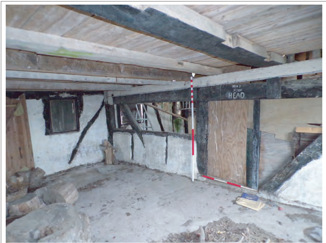
Plate 50: Oblique view south west of eastern face of surviving partition. Note reused and modern timbers forming floor joists of loft space above. Scales 1x1m & 1x2m
