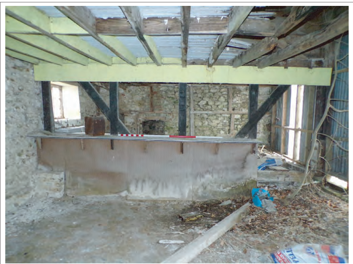
Plate 64: View east into semi-domestic partitioned off area within end of 1870s extension. Scale 1x2m
