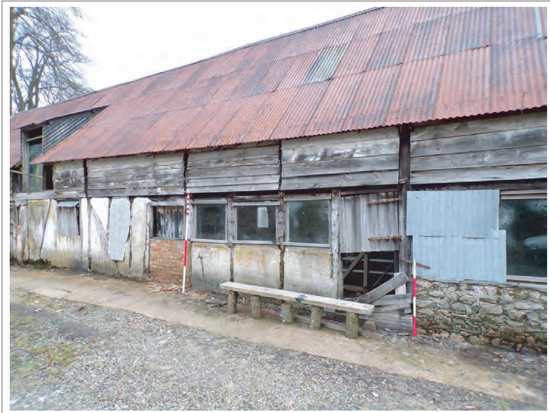
Plate 7: Oblique view of doorways within southern elevation Looking north west, Scales 1x1m & 1x2m
