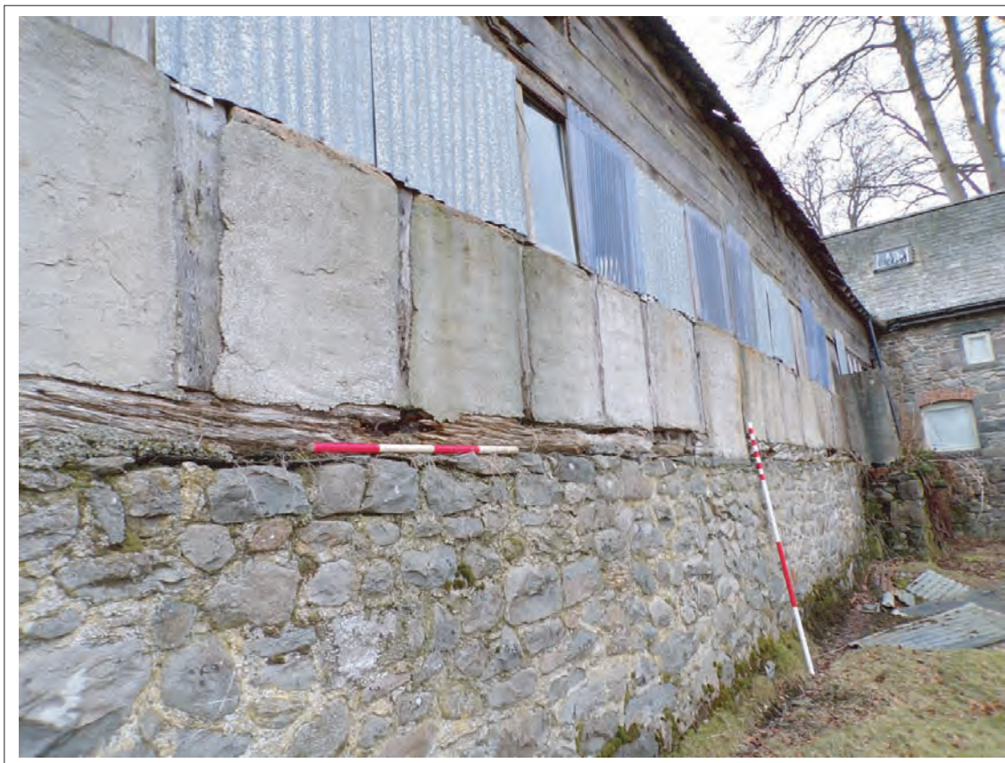
Plate 21: View of timber frame within south elevation. Looking south west Scales 1x1m & 1x2m
