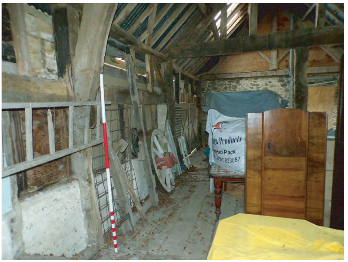
Plate 38: View west along internal face of southern elevation. Note planked area on floor. Scale 1x2m
