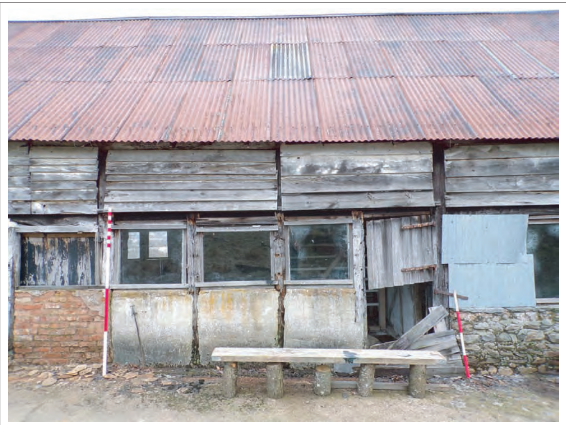
Plate 6: View of 1772 timber frame structure with original doorways on left and right within southern elevation. Looking north, Scales 1x1m & 1x2m
