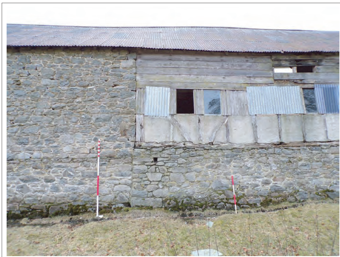
Plate 22: View of butt joint between 1772 structure (right) and 1870s extension (left) Looking south, Scales 1x1m & 1x2m
