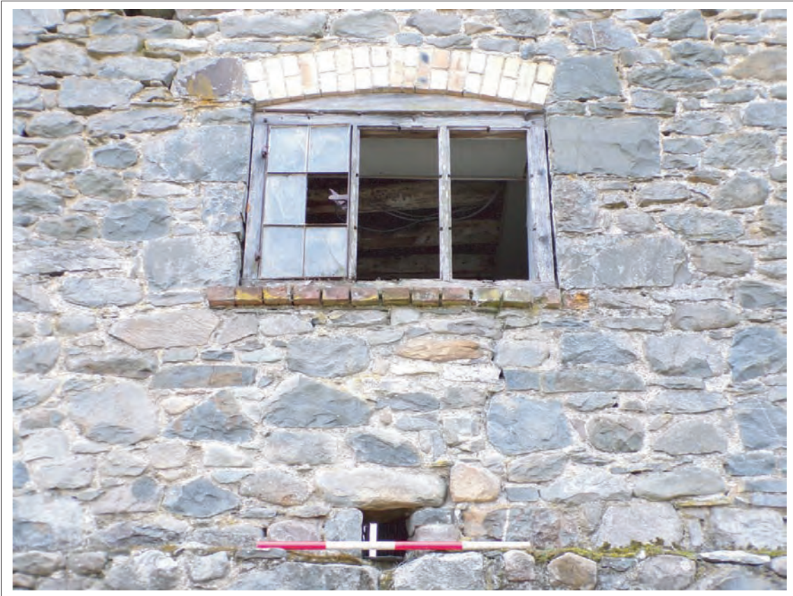
Plate 28: View of window opening within eastern end of southern elevation Scale 1x1m
