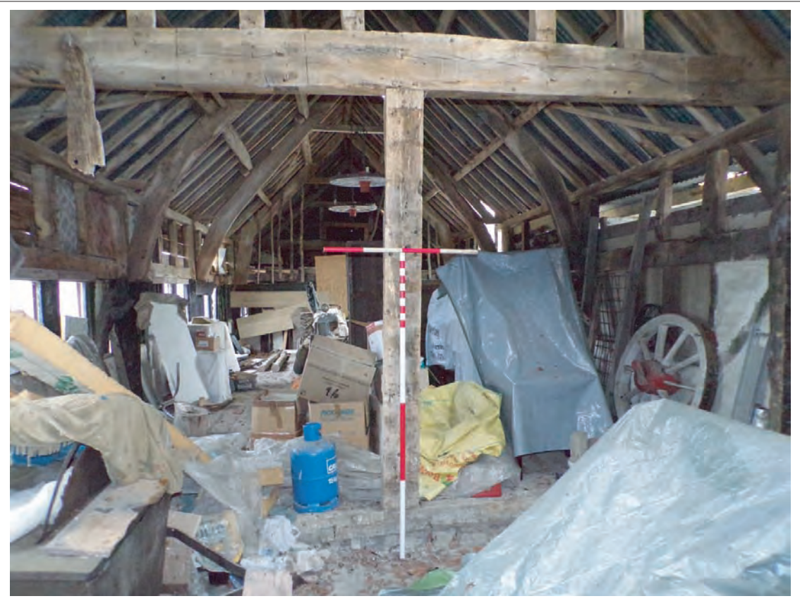
Plate 34: View east along original 1772 cowhouse with box frame gable end in foreground. Note exposed sill beam and change in ground level beyond. Scales 1x1m & 1x2m
