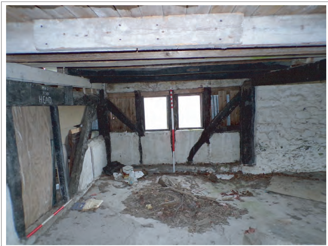
Plate 54: View of rear (north) wall of westernmost bay. Note 1870s stone extension to right butting easternmost gable end box frame, Scale 1x1m & 1x2m
