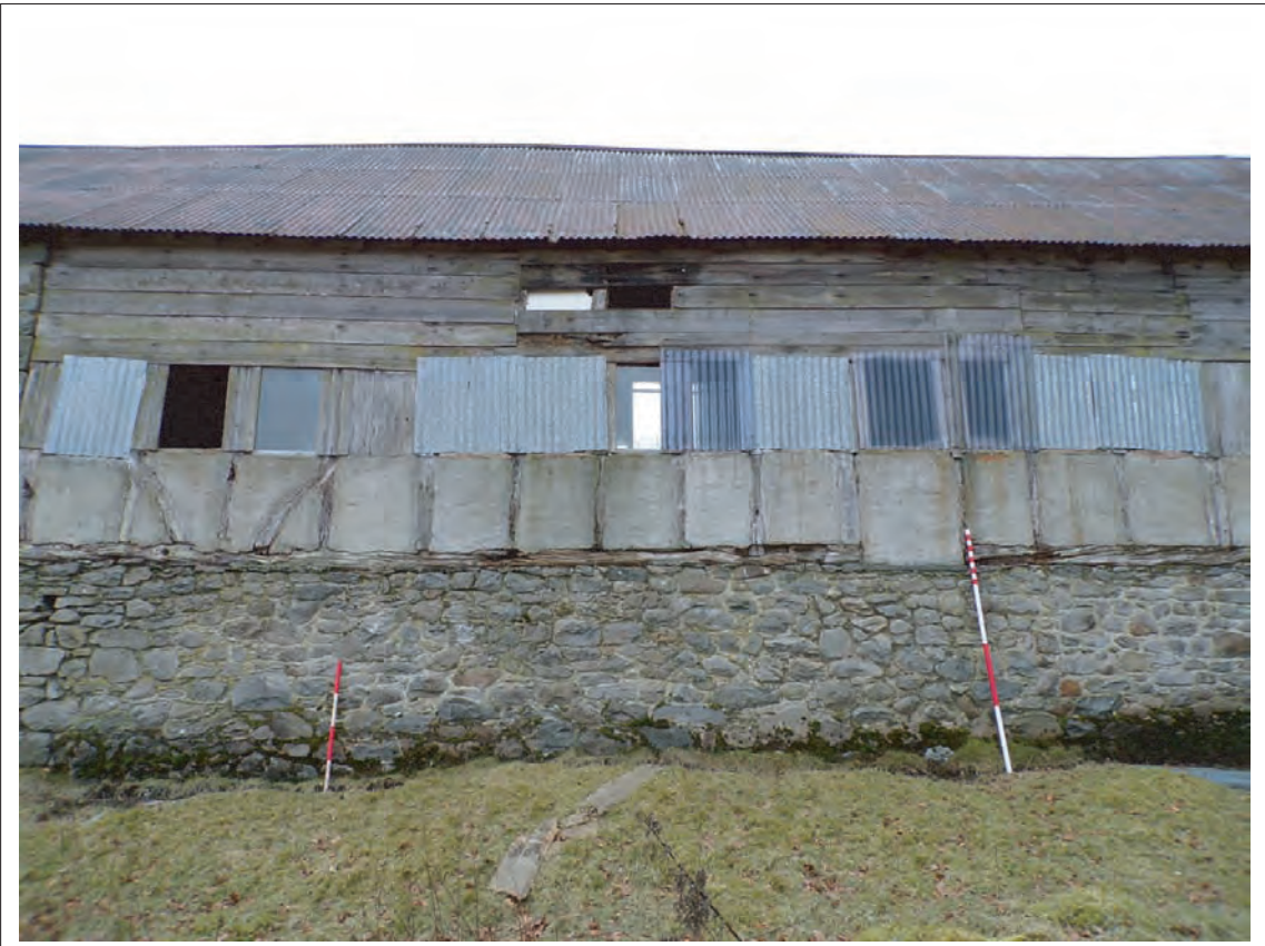
Plate 18: View within south elevation of 1772 timber frame sat on stone platform Looking south, Scales 1x1m & 1x2m
