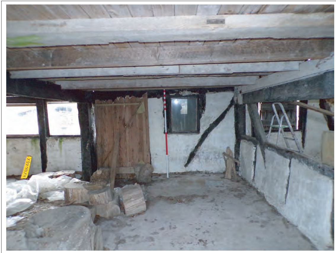
Plate 53: View of original entrance into westernmost bay in southern elevation Looking south, Scale 1x2m
