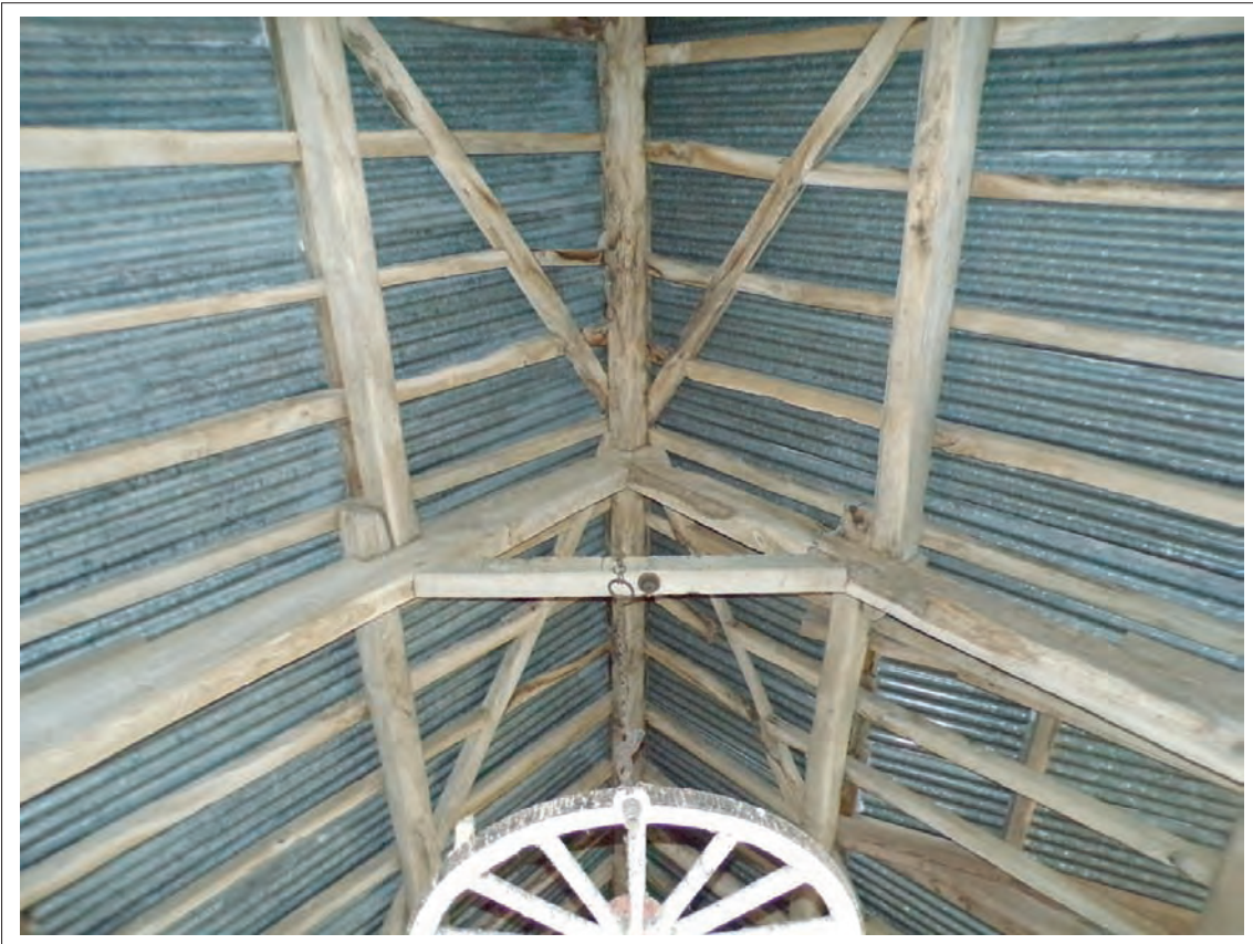
Plate 45: View of roofing detail within centre of 1772 structure including wind brace forming diagonal cross across rafters.
