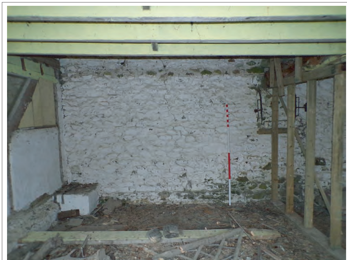
Plate 62: View north of internal face of northern elevation within 1870s extension Scale 1x2m
