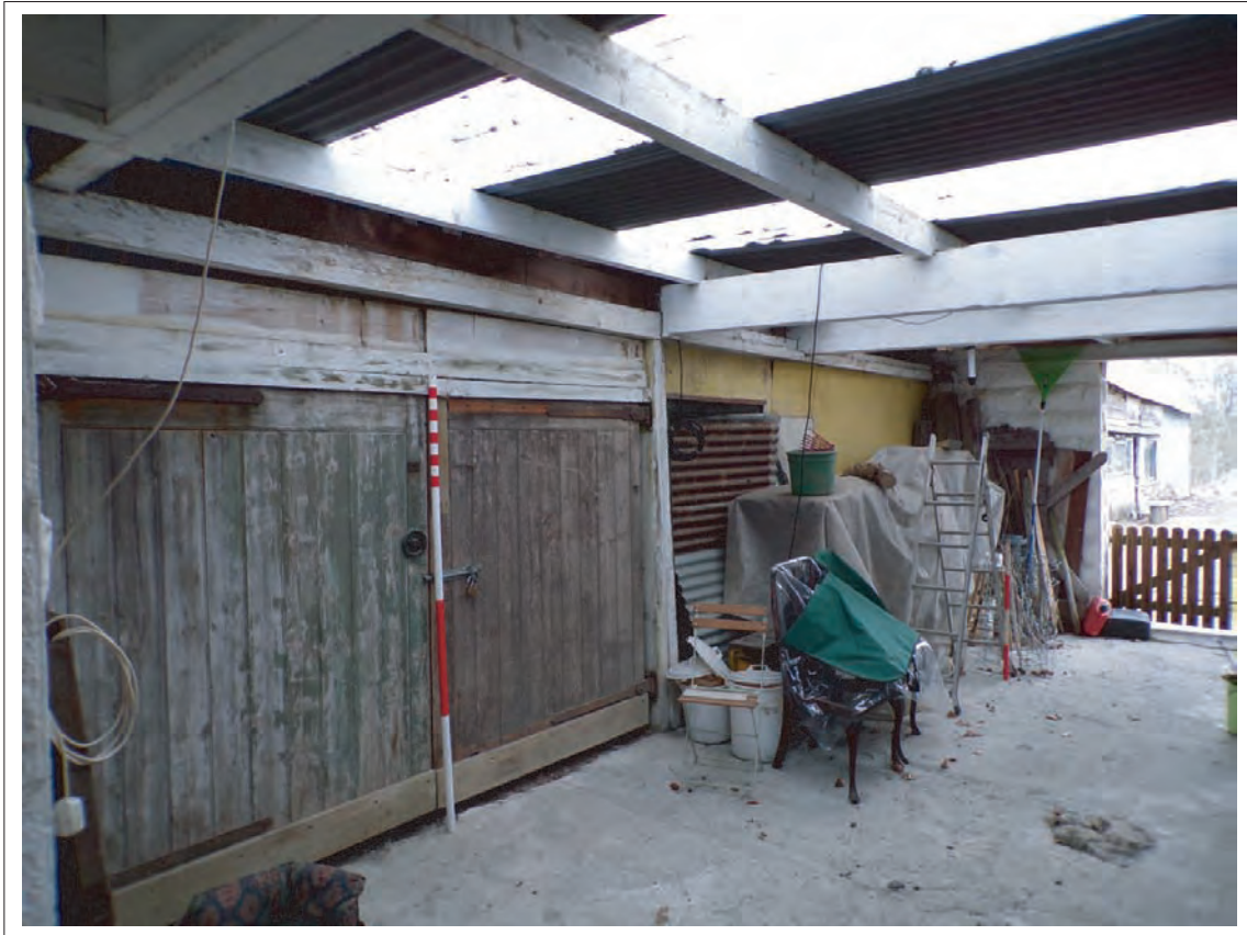
Plate 13: View of current entrance within 1870s western extension. Looking north east Scales 1x1m & 1x2m
