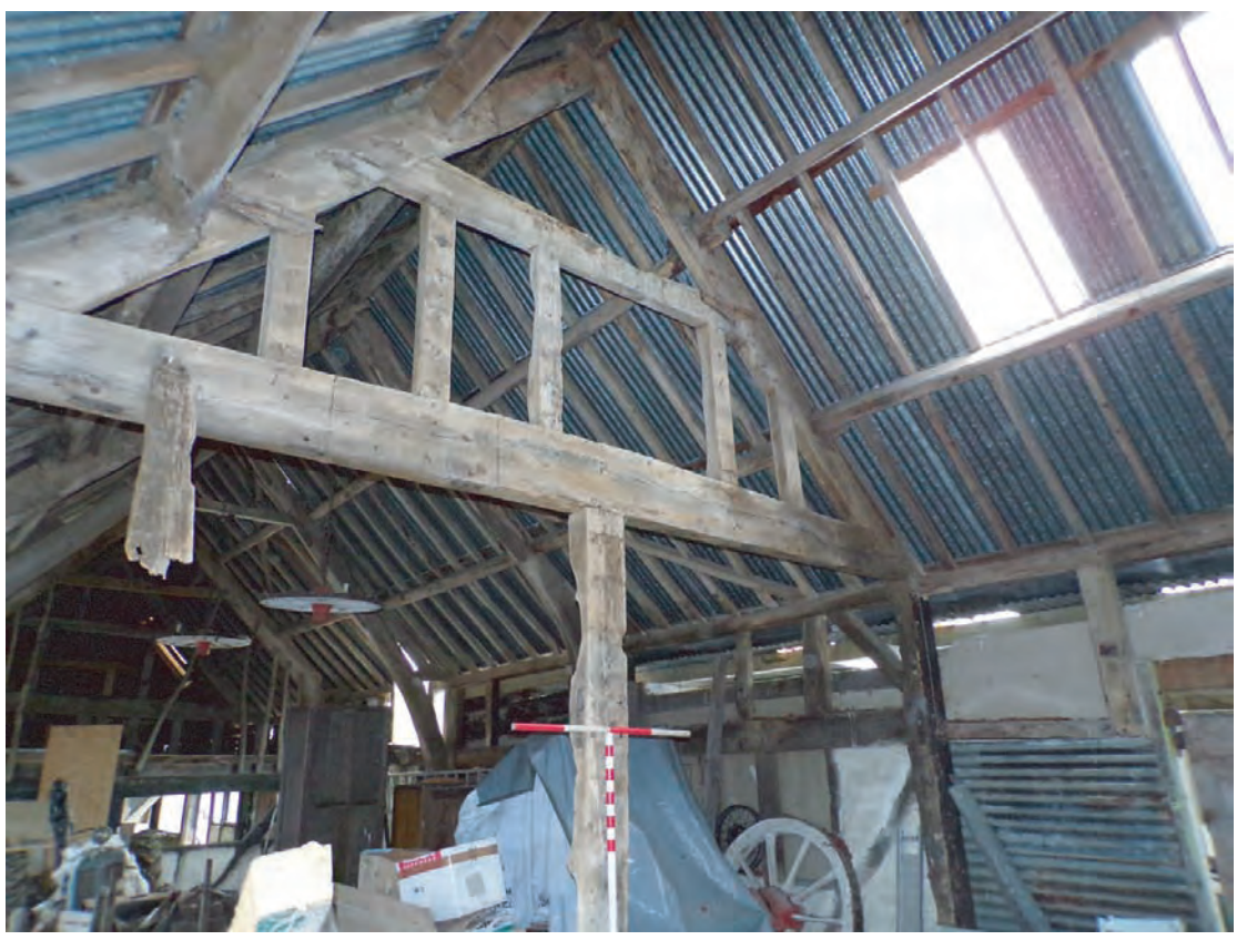
Plate 37: Oblique view south east of upper surviving timbers of 1772 box frame gable end. Scales 2x1m
