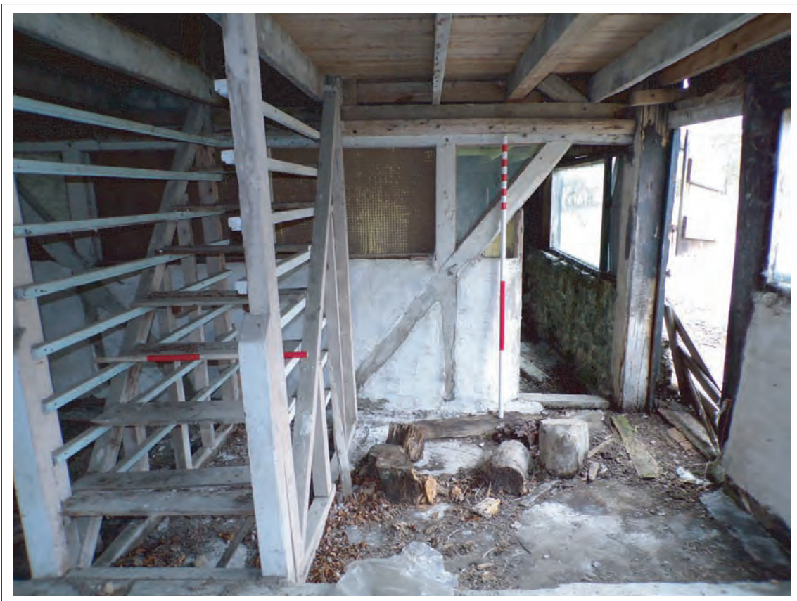
Plate 57: View of westernmost timber partition within 1870s extension and access to loft space above. Looking east, Scales 1x1m & 1x2m
