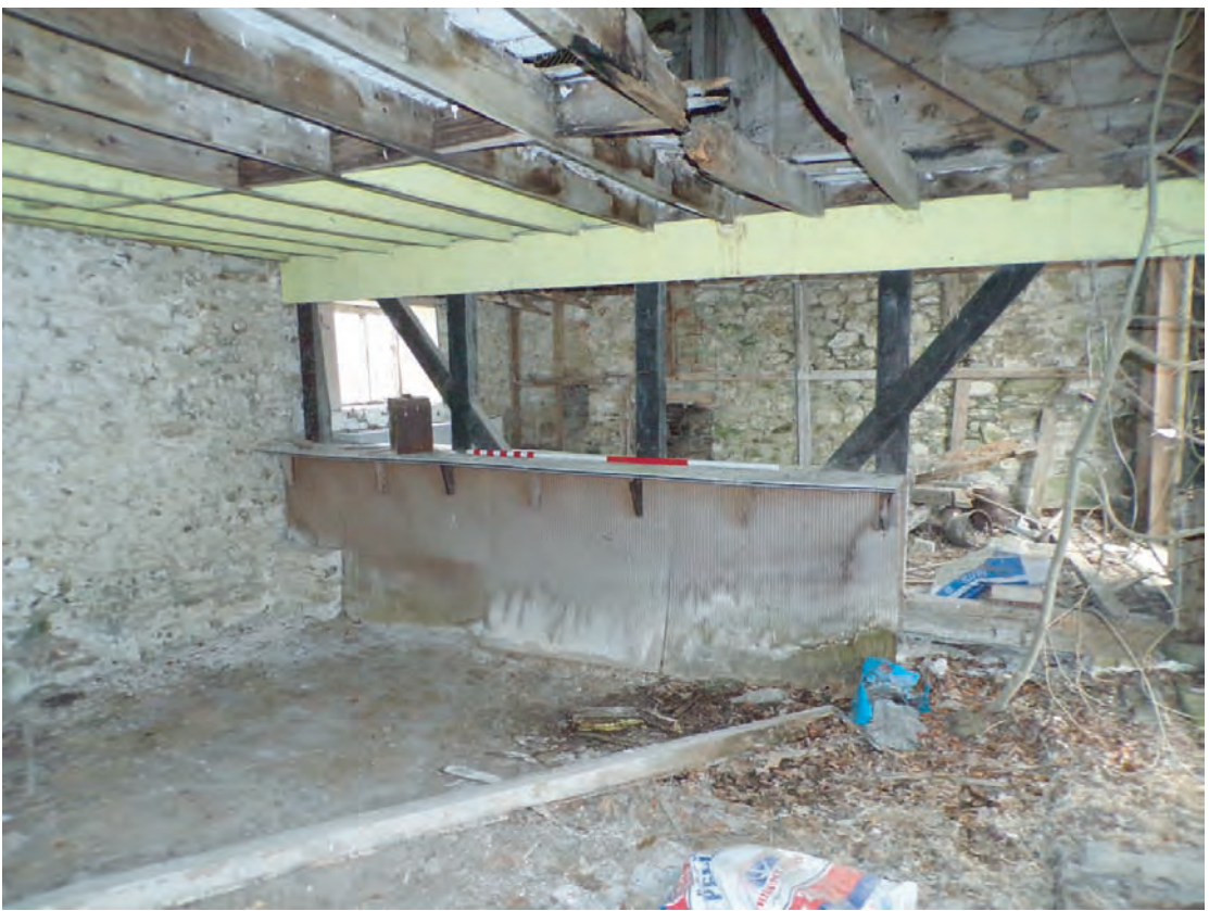
Plate 70: View of easternmost partition within 1870s extension. Looking north east Scale 1x2m. Note state of floor joists above
