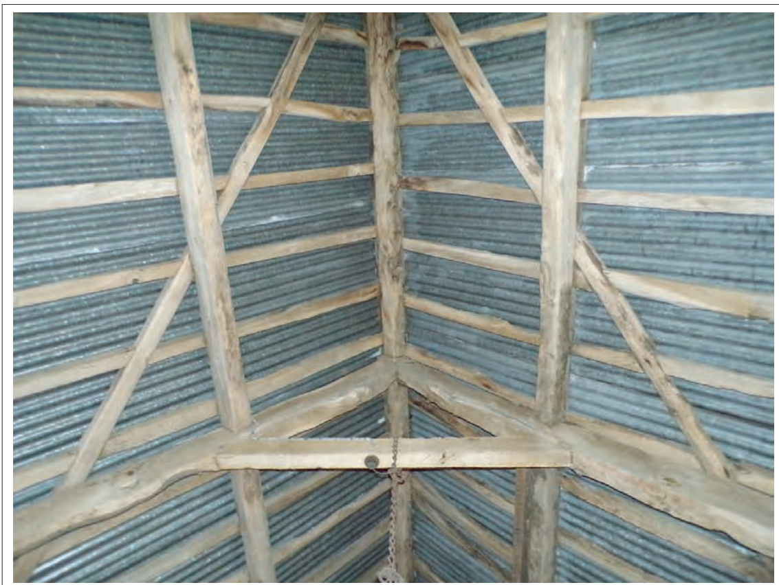
Plate 46: View of roofing detail showing wind brace crossing principal rafters of cruck
