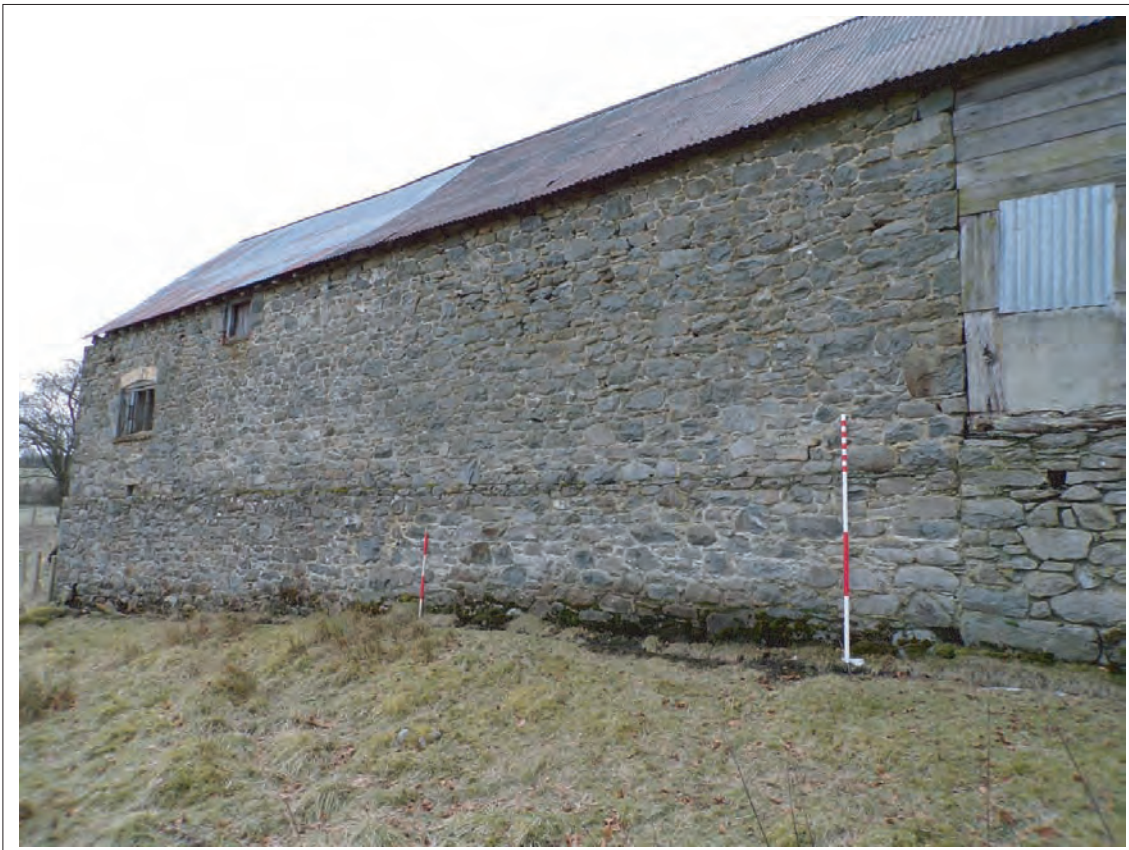
Plate 24: View of southern elevation of 1870s extension Looking south east, Scales 1x1m & 1x2m
