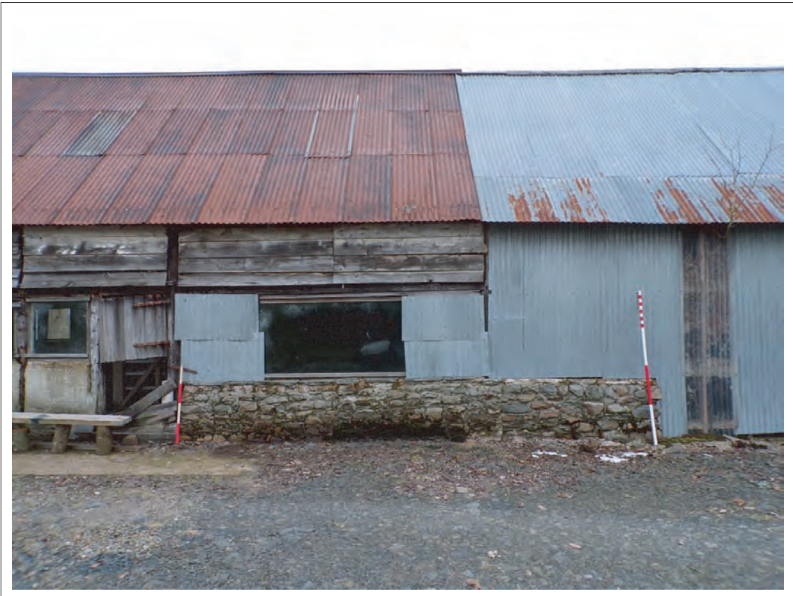
Plate 5: View of southern elevation where 1870s extension butts 1772 cowhouse Looking north, Scales 1x1m & 1x2m
