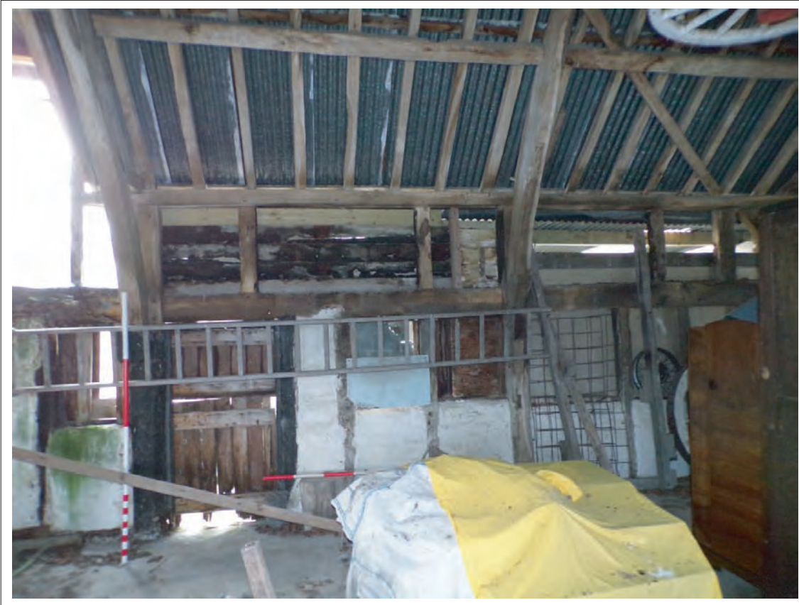
Plate 47: View of original doorway into bay between two crucks within southern elevation. Looking south, Scales 1x1m & 1x2m
