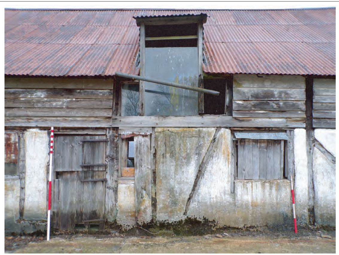
Plate 10: View of blocked (right) and original entrance (left) within southern elevation as well as modern window above middle. Looking north, Scales 1x1m & 1x2m
