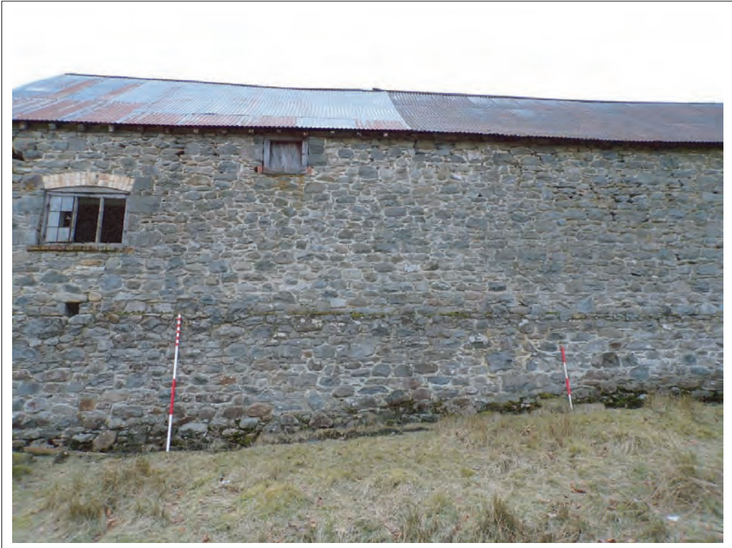
Plate 25: View of southern elevation of 1870s extension Looking south, Scales 1x1m & 1x2m
