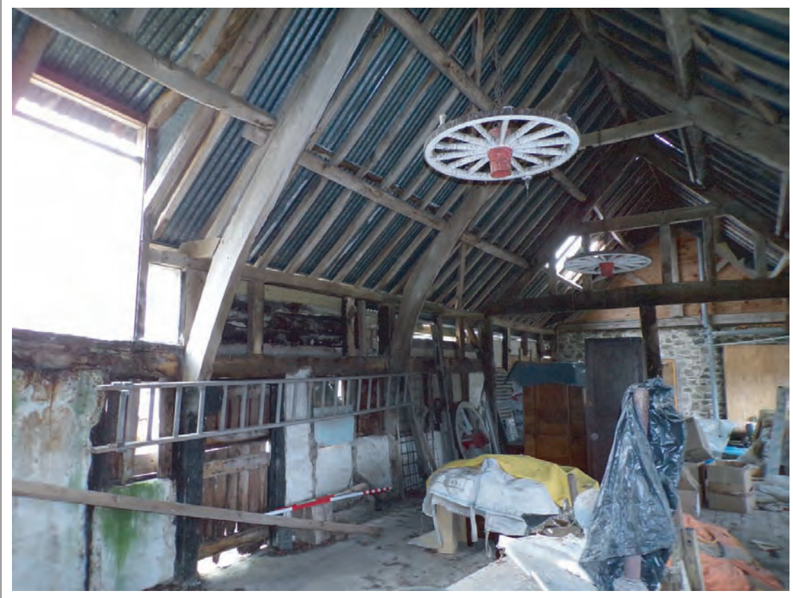
Plate 43: Oblique view looking south east along internal face of southern elevation Scale 1x2m
