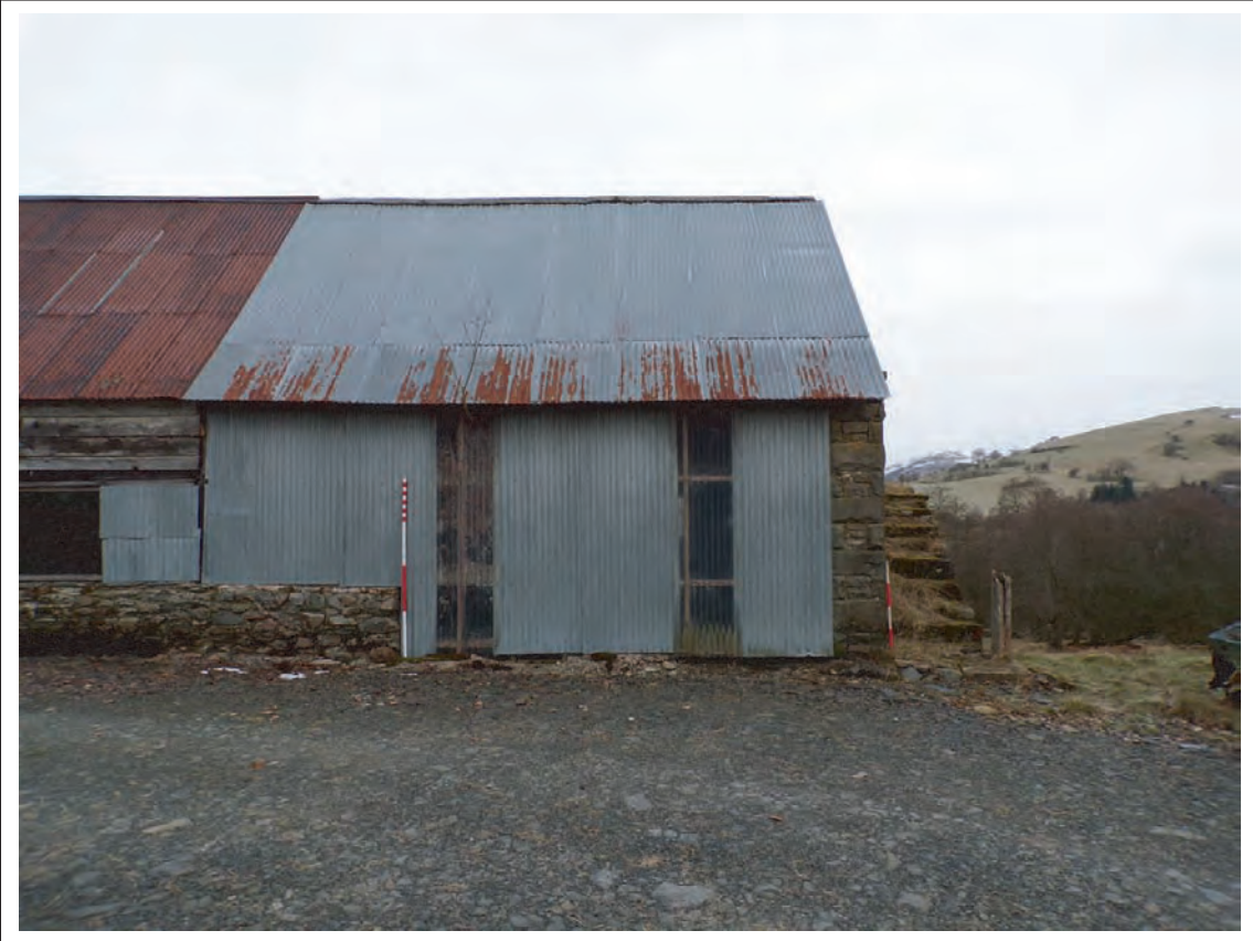
Plate 3: View of eastern end of south facing elevation, looking north Scales 1x1 & 1x2m
