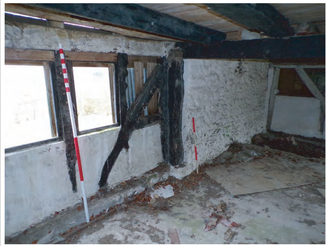
Plate 55: View north east showing butt joint between timber 1772 structure and 1870s stone extension. Scales 1x2m & 1x1m
