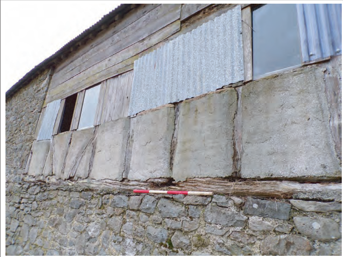
Plate 20: Detail view of timber frame deterioration within north elevation Note cement infill/repair. Looking south east, Scale 1x1m
