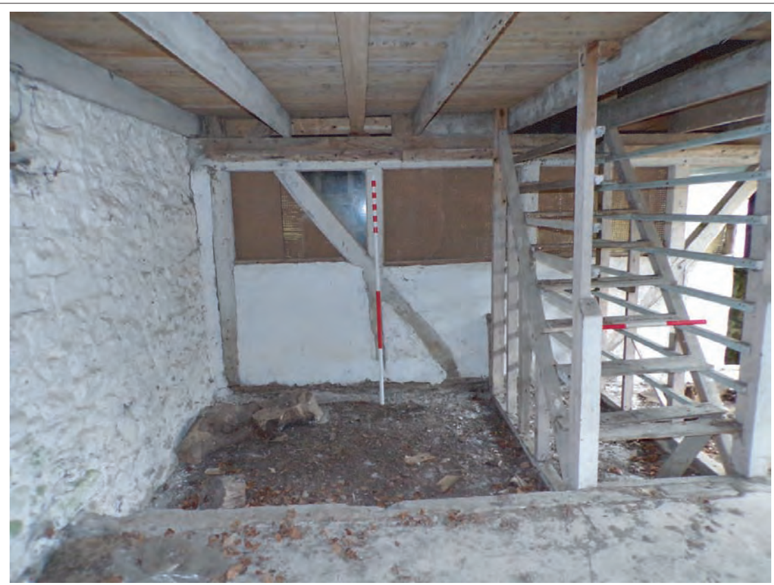
Plate 56: View of westernmost timber partition within 1870s extension and access to loft space above. Looking east, Scales 1x1m & 1x2m
