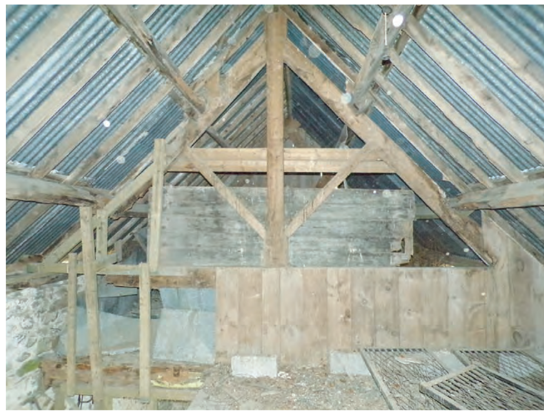
Plate 74: View of upper timbers of king post partition of 1870s extension (lower timbers removed) within loft space, looking east
