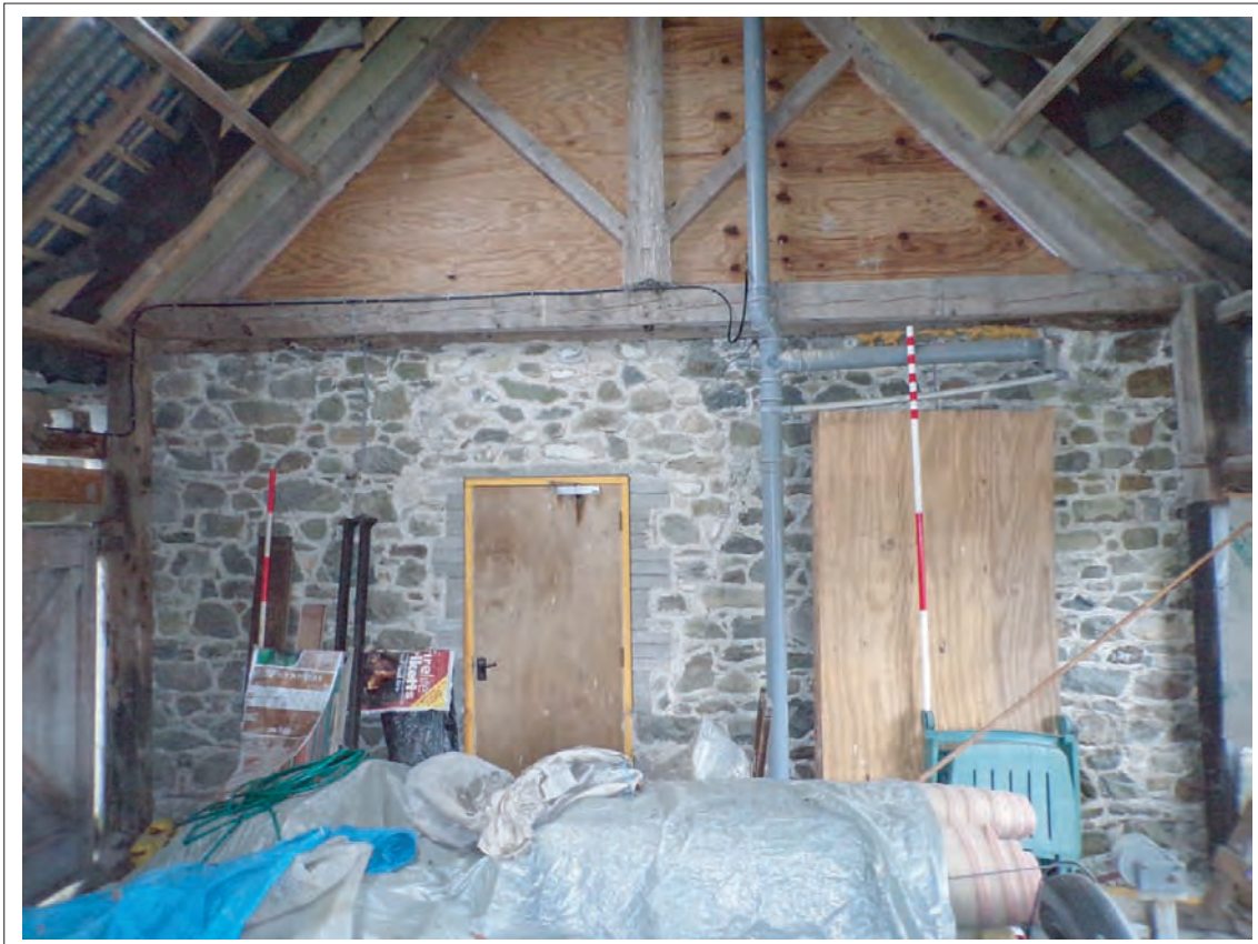
Plate 31: View west of timber king post frame butting north-south range Scales 1x1m & 1x2m
