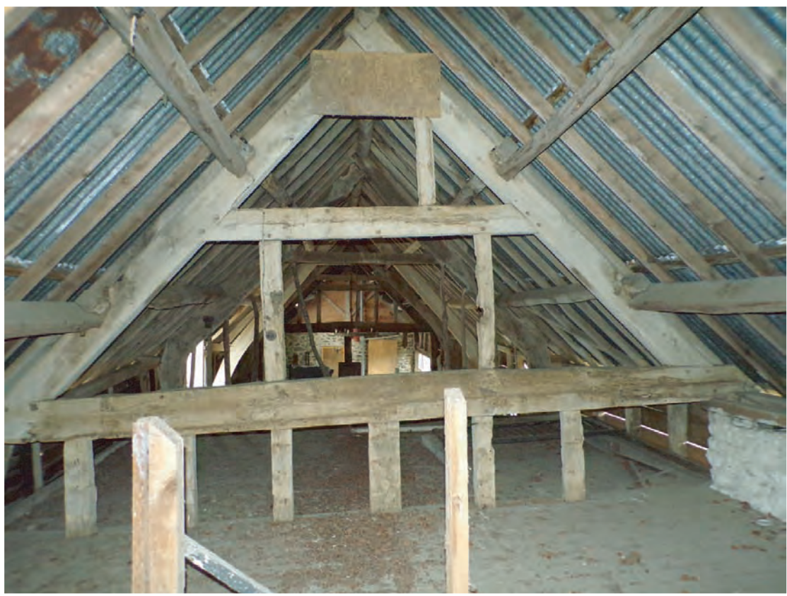
Plate 73: View of upper timbers of eastern 1772 gable end, looking west within loft space Note stone extension butting in bottom right
