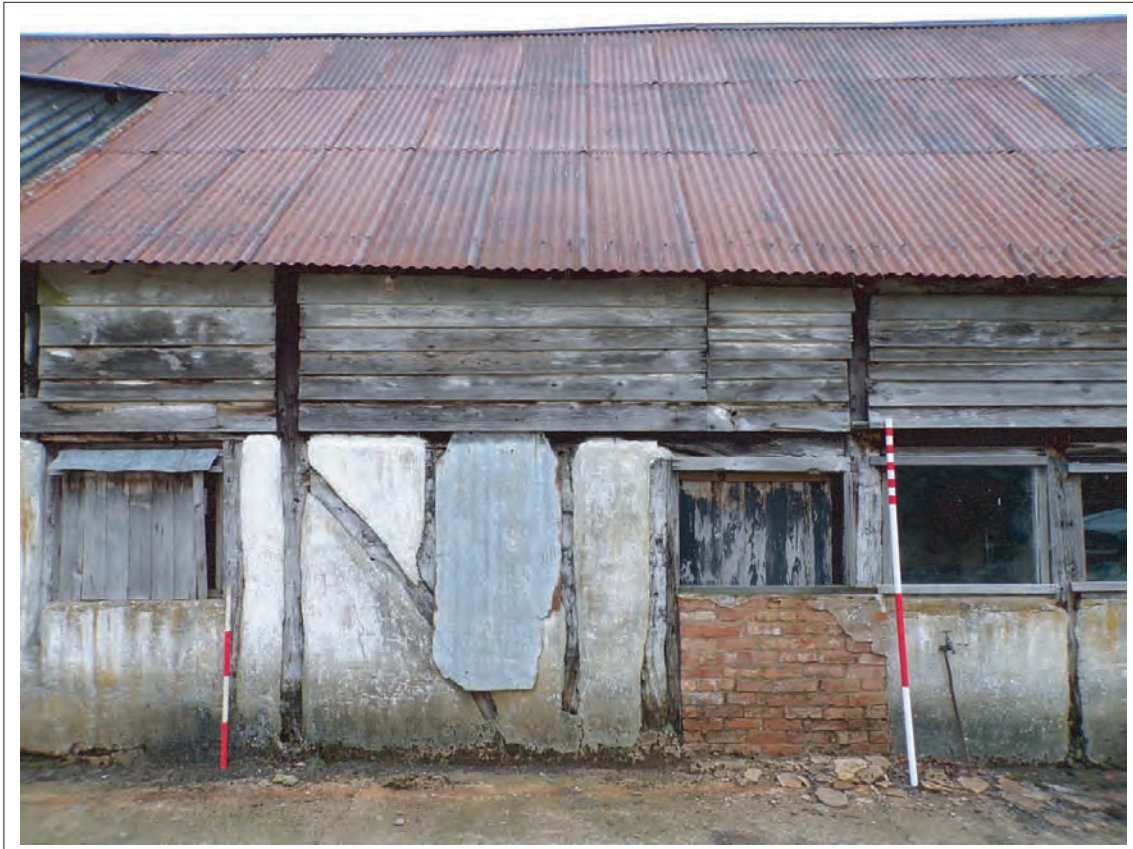
Plate 8: View of blocked doorways within southern elevation to left of each ranging rod Looking north, Scale 1x1m & 1x2m
