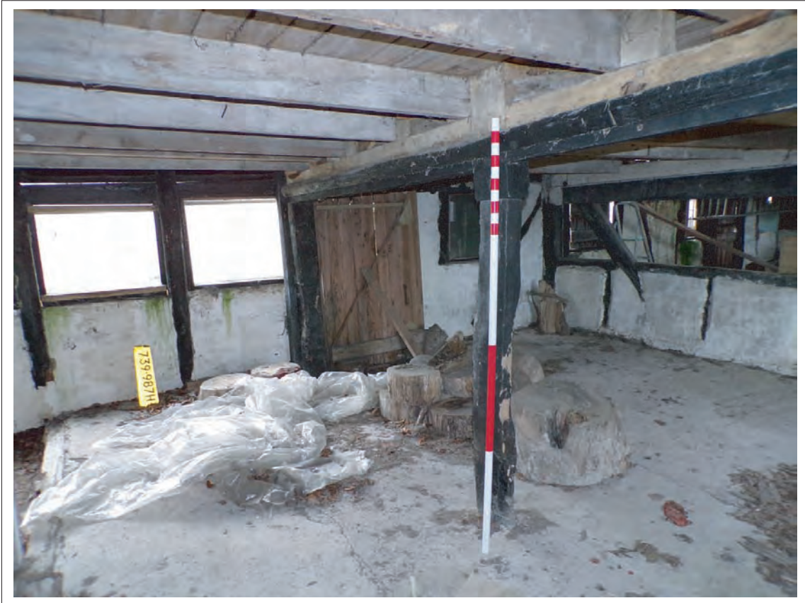
Plate 59: View of replaced central support within eastern box frame gable end Looking south east, Scale 1x2m
