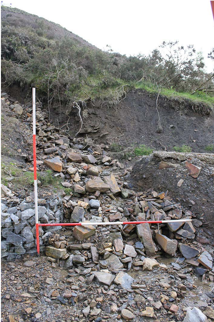
a. Before excavation - showing the deposit of water bourned rocks on the tramway edge
