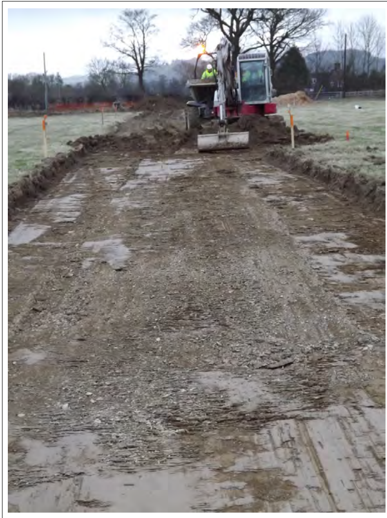
Plate 3: View of road excavation underway. Note patch of gravel banding within surface of subsoil
