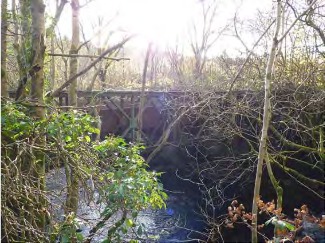
Photo 27: View ESE of the surviving rail bridge across the river to the northeast of the site.
