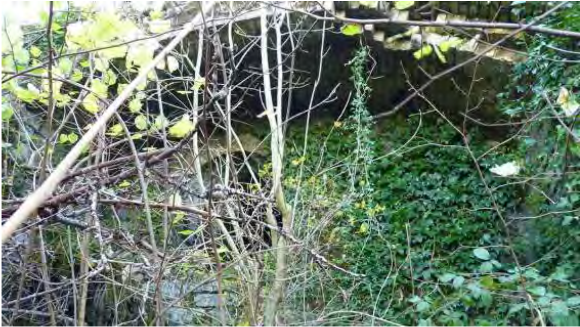
Photo 15: View S of the westernmost arched recess, shrouded in undergrowth. The smaller arched passage is just about visible in the centre.
