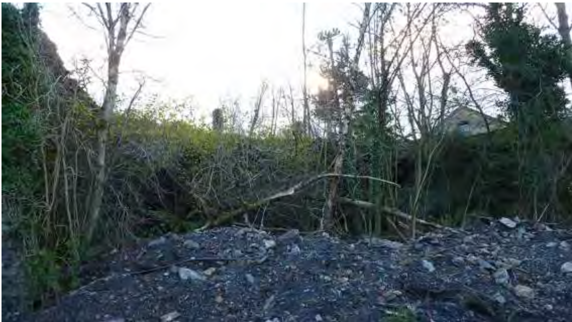
Photo 12: View SSE showing the vegetation and rubble that has built up in front of the possible Boiler House Wall.
