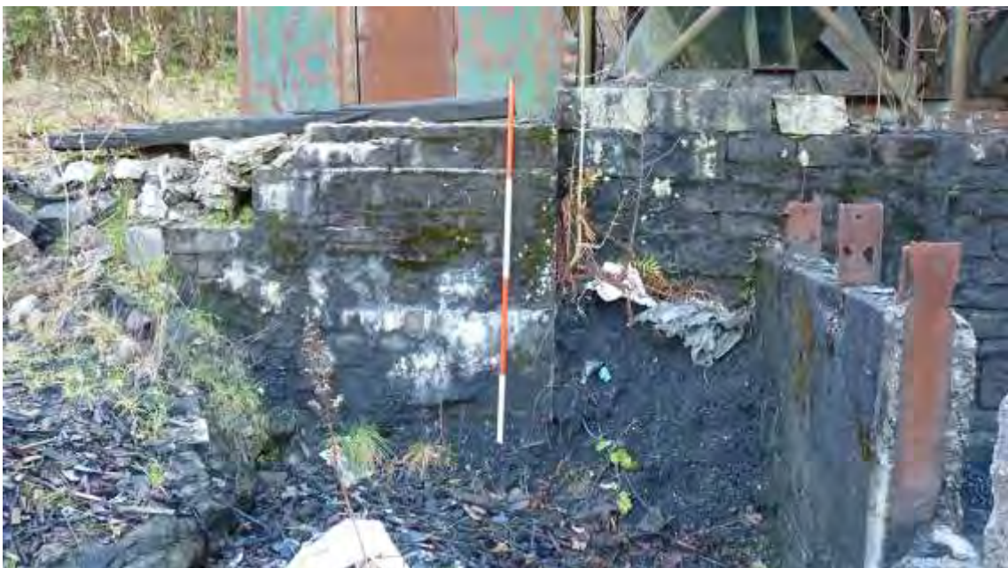
Photo 18: View SSE showing the two adjoining early walls, thought to be surviving elements of the ironworks and brickworks buildings. 2m scale.
