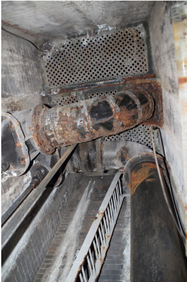
Figure 14. Looking up into the shaft in the east tower, at the end of the tunnel to the grating shown in Fig. 13
