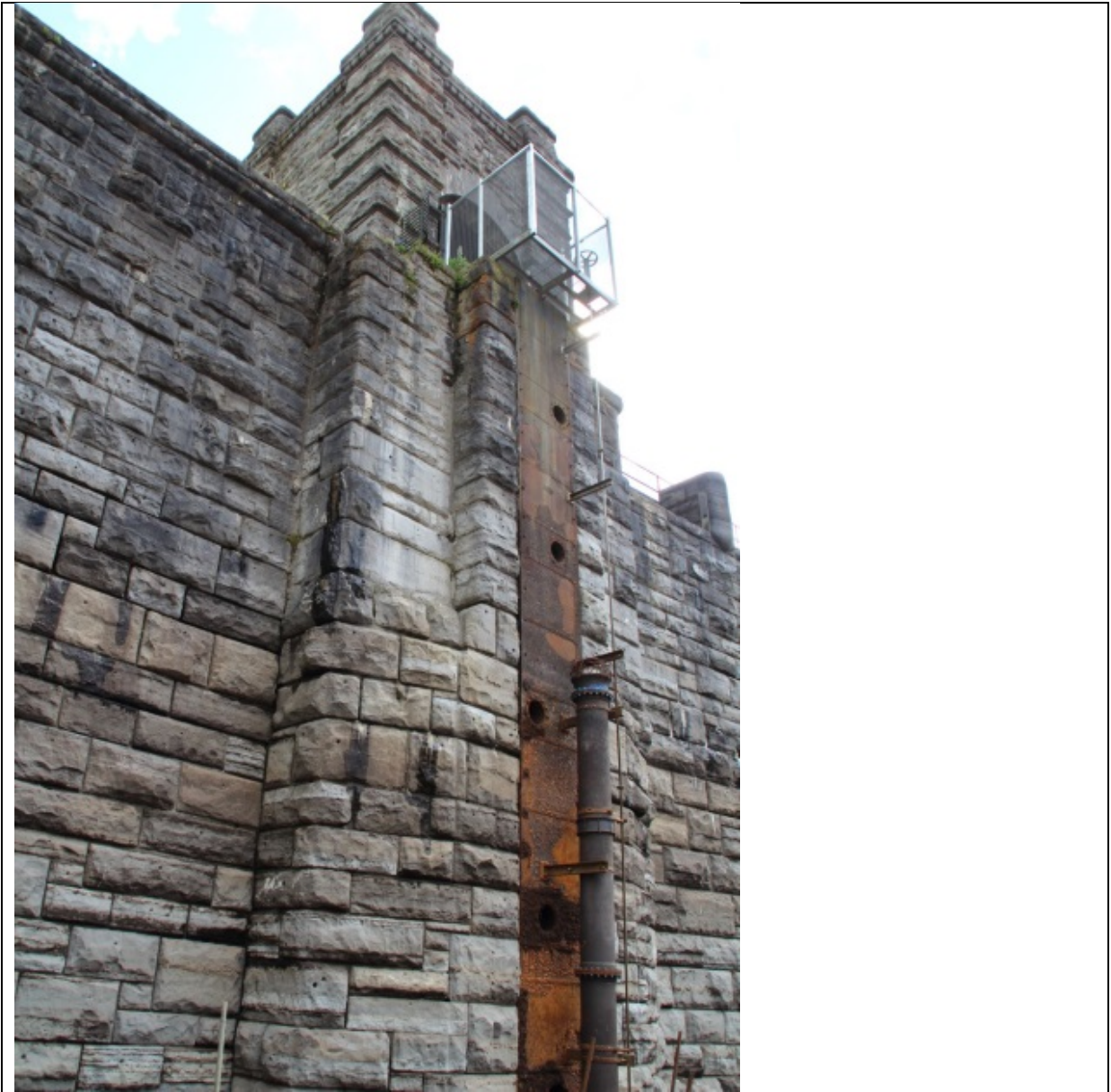
Figure 16 The north face of the east tower, showing inset steel duct and now-redundant presumed level control valve sites, looking south-west
