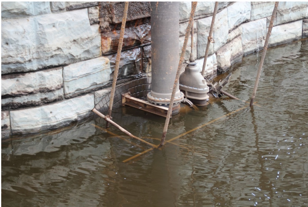
Figure 15. The brick voussoirs of the tunnel visible on the north side of the dam and the pipe, valve and control gear, looking south-west
