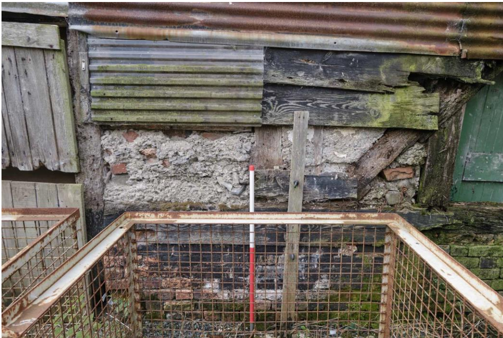
Figure 11. Unreinforced concrete in the north wall of the main barn.
