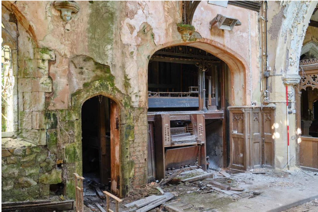
Figure 14. South wall of the chancel, with a wide arch to accommodate the organ.
