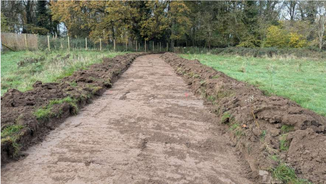
Plate 6: Strip area leading to plantation woodland, looking south, with patches of red clay exposed along western edge of excavated area.
