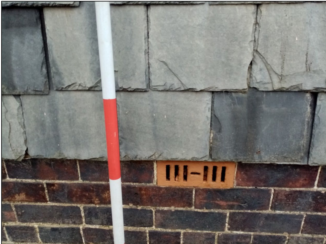
Plate 6: GCP2023_006. A view of detail of an air brick on the southern wall of the chapel. Looking north-northeast. The red section of the scale represents 20 centimetres.
