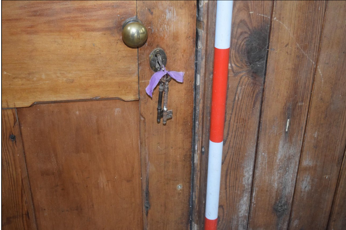
Plate 24: GCP2023_024. The original keys in the doorway to the south side of the pulpit. Looking west-northwest. Red section of scale is 20 centimetres.
