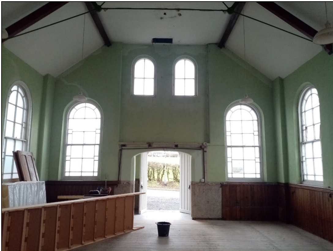
Plate 18: GCP2023_0018. A view of the interior of the chapel, looking towards the eastern end of the building, with the main door open. Looking east-southeast.
