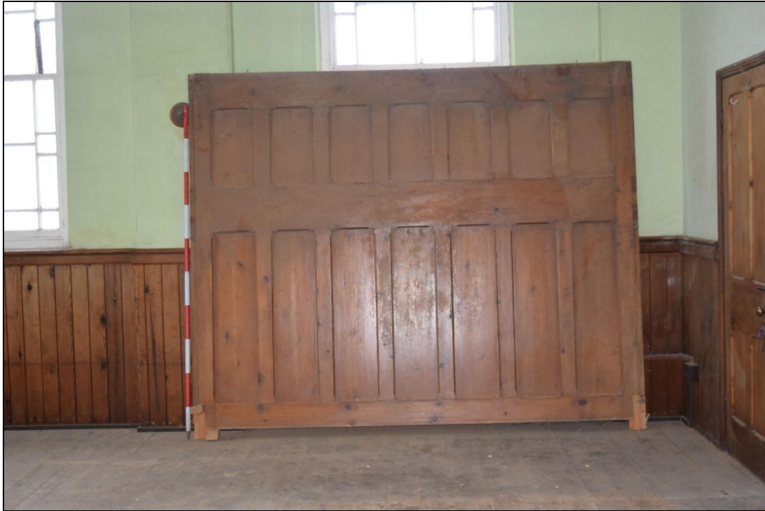
Plate 28: GCP2023_028. A view of a wooden panel which formerly formed part of the inner lobby inside the main entrance of the chapel. Looking south-southwest. Two metre scale.
