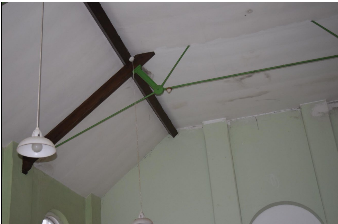
Plate 37: GCP2023_037. A view of the ceiling at the southwest corner inside the chapel, showing exposed wooden roof timbers and iron reinforcement bars. Looking west.
