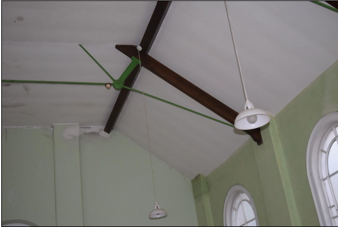
Plate 38: GCP2023_038. A view of the ceiling at the northwest corner inside the chapel, showing exposed wooden roof timbers and iron reinforcement bars. Looking north-northwest.
