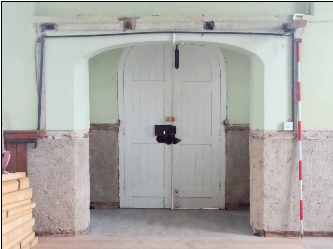
Plate 29: GCP2023_029. A view inside the chapel looking towards the main door. The scar of the inner lobby which formerly existed inside the porch can be seen on the wall. Looking east-southeast. Two metre scale.
