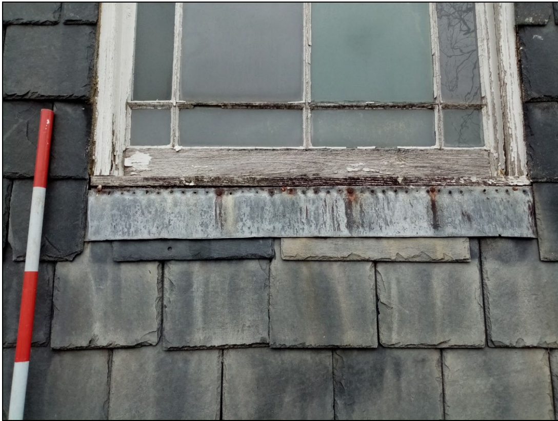
Plate 5: GCP2023_005. A view of detail of lead flashing and slates covering the southern wall of the chapel. Looking north-northeast. Three full 20 centimetres of 1 metre scale visible.
