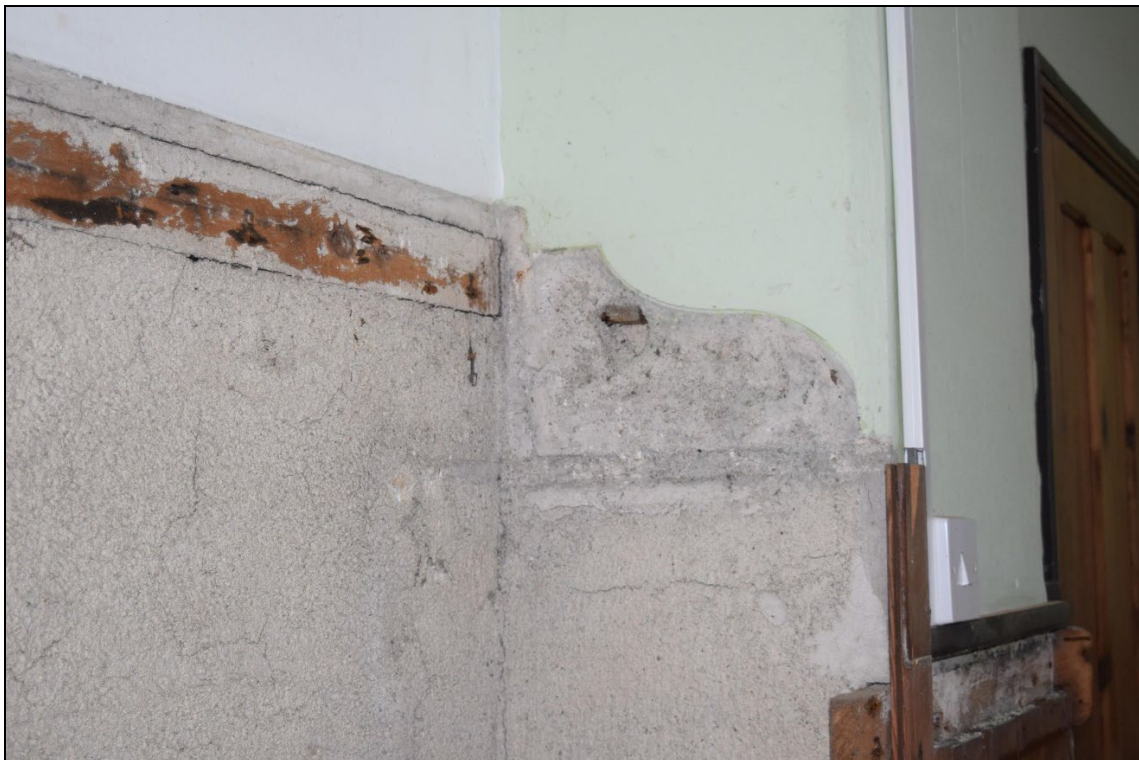
Plate 35: GCP2023_035. A view of a scar left by the now removed pulpit against the western gable wall of the chapel. Looking north.
