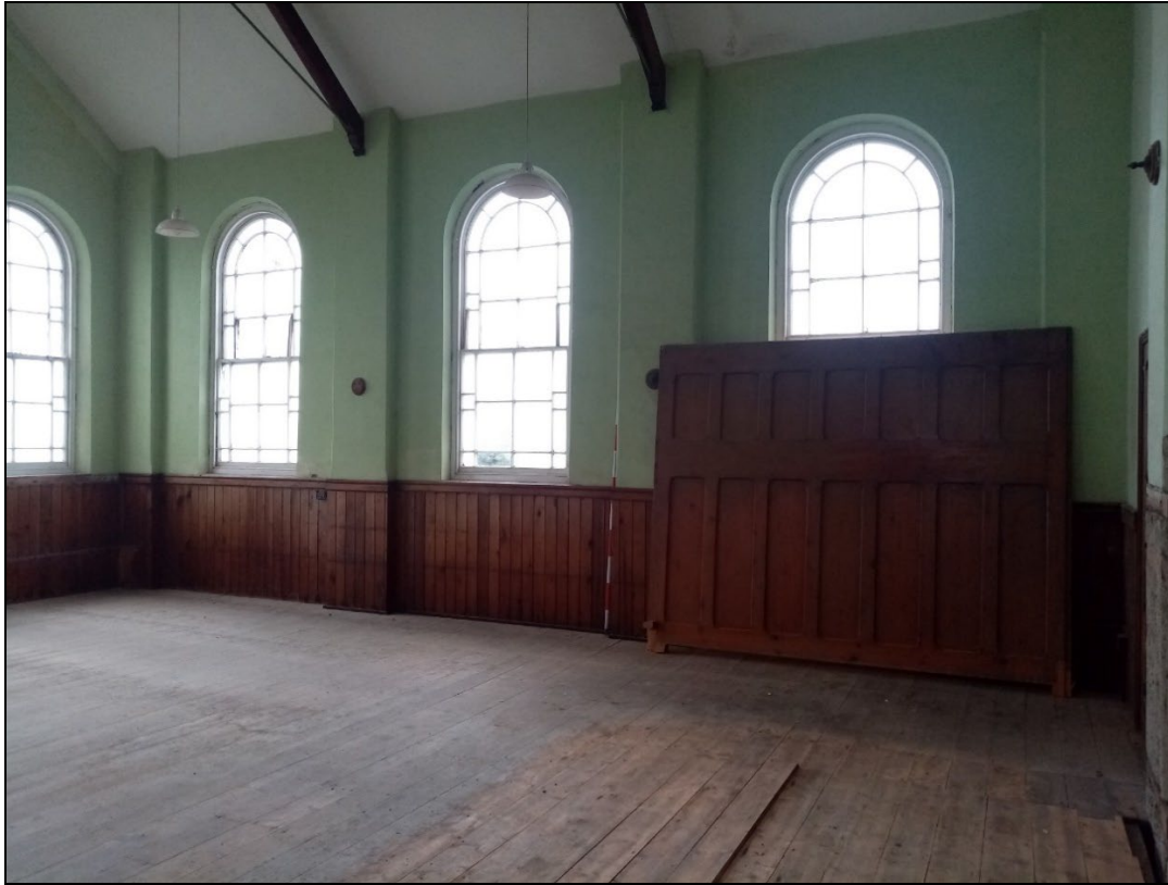
Plate 13: GCP2023_013. A view of the interior of the chapel, looking towards the southern side of the building. Looking south-southeast. Two metre scale. The wooden partition was originally by the main door creating a small internal lobby.
