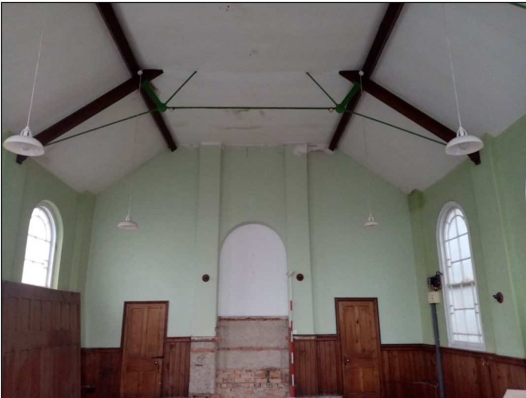
Plate 12: GCP2023_012. A view of the interior of the chapel, showing exposed roof timbers and an iron reinforcement frame in the ceiling. Looking west-northwest. Two metre scale.
