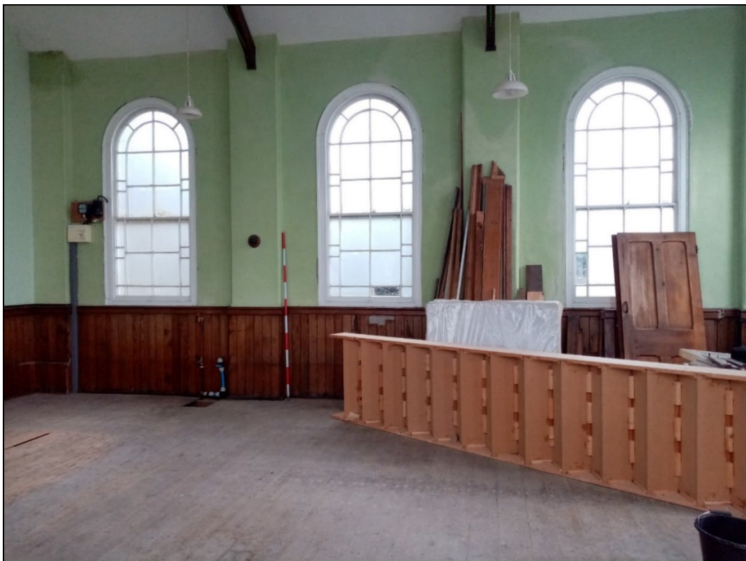
Plate 16: GCP2023_016. A view of the interior of the chapel, looking towards the northern side of the building. Looking north. Two metre scale
