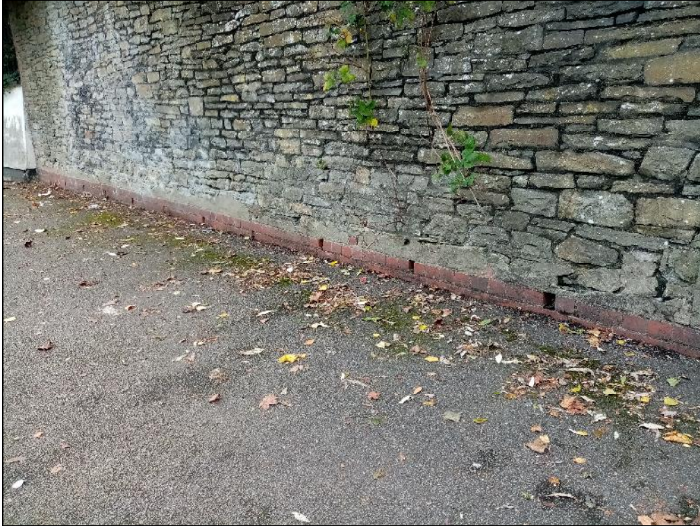
Plate 7: A view towards the base of the stone wall forming the eastern property boundary, looking southwest. Note the brick courses with drainage holes below.
