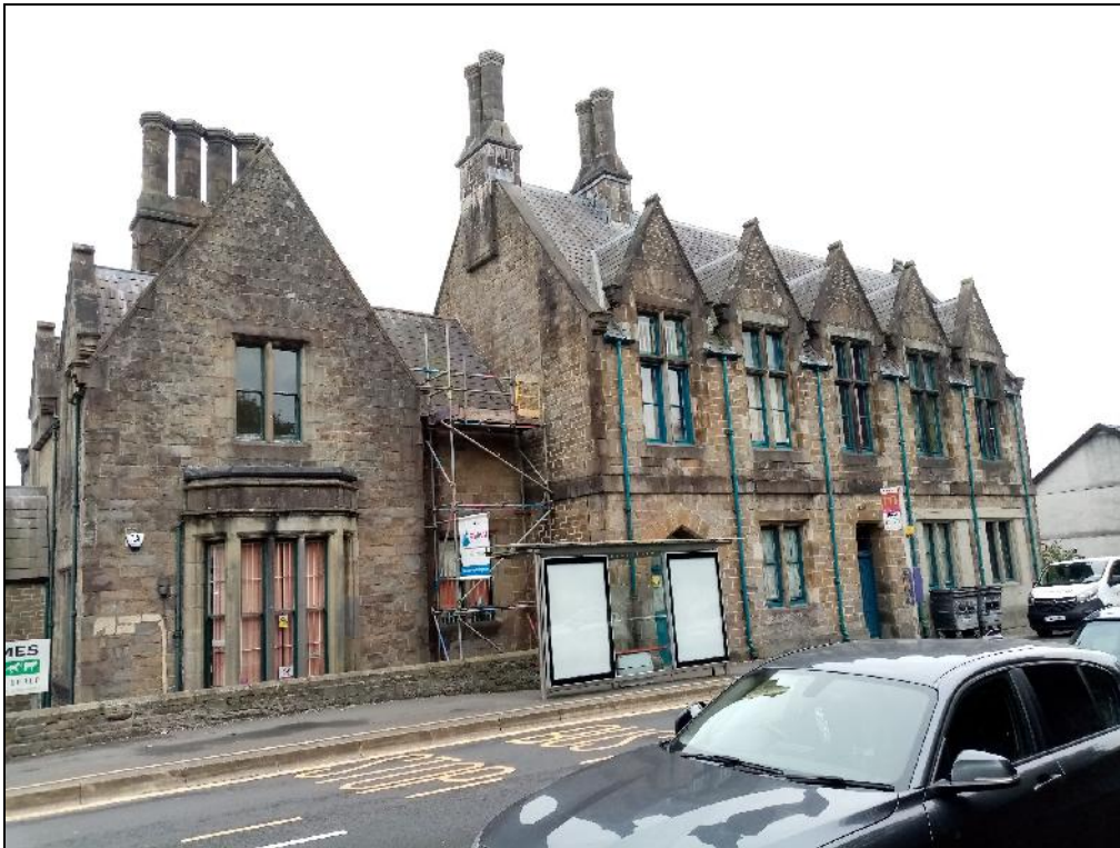
Plate 8: A view towards the former Police Station and house, both Listed Buildings from outside 69 Martin Street, looking southeast.
