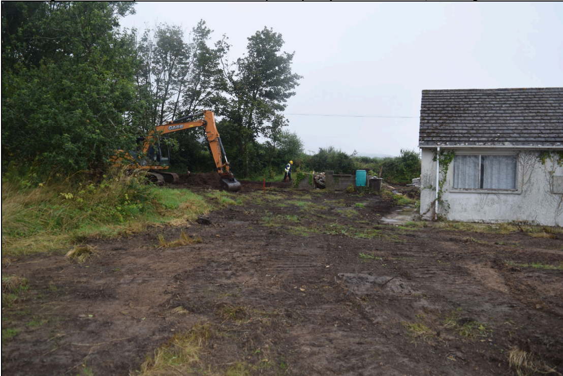
Plate 6: PCG2021_106 General view of the western side of the plot and existing dwelling after vegetation scraped off but before topsoil (001) was removed, looking north-northeast
