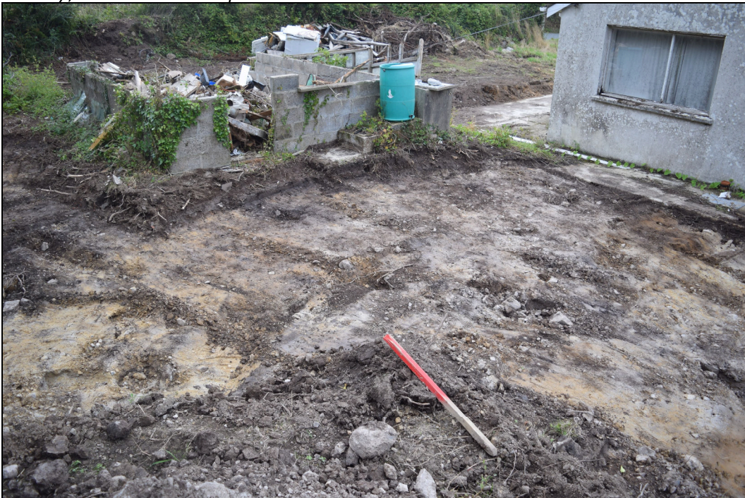
Plate 28: PCG2021_128 After removal of (001) to the west side of the current house, looking east. The surface of the subsoil undulated suggesting that the ground was formerly more uneven. This area was also impacted by remains from the nursery, such as modern postholes
