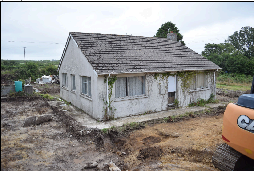
Plate 26: PCG2021_126 After removal of (001) to the southern side of the current house, looking east-northeast. The surface of the subsoil undulated suggesting that the area to the south of the house was on slightly higher ground surrounded by lower ground, or small streams.
