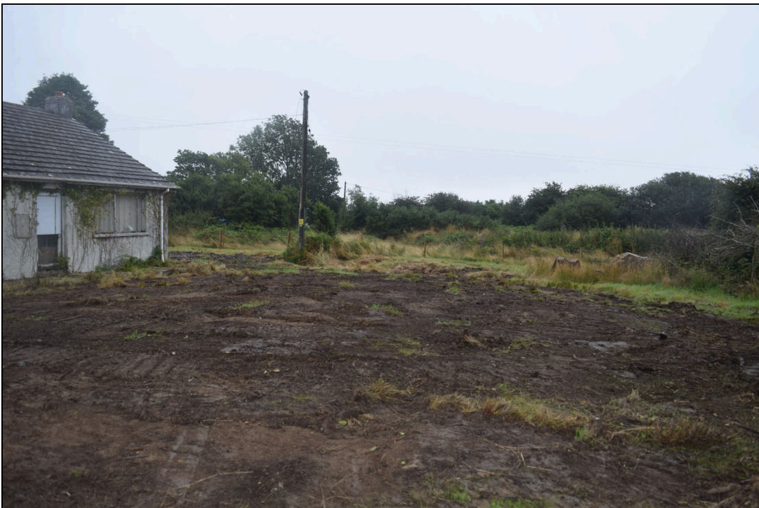
Plate 8: PCG2021_108, General view of the southern side of the plot after vegetation scraped off but before topsoil (001) was removed, looking east-southeast.
