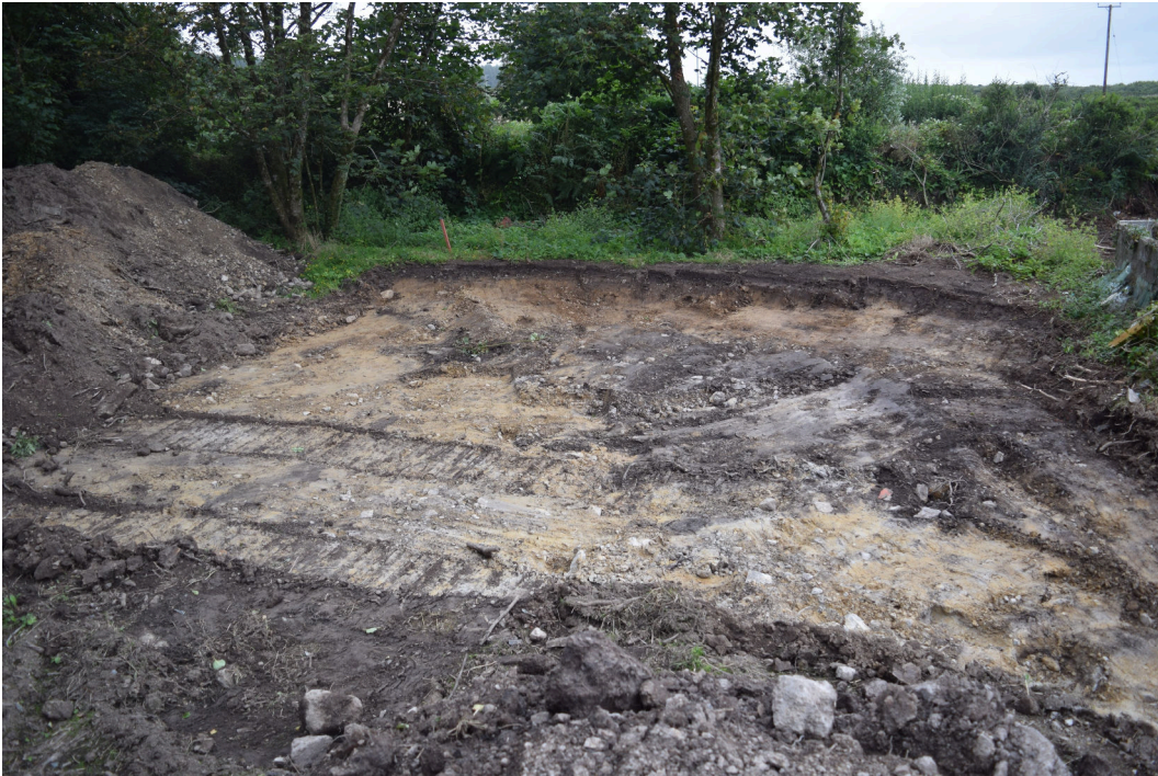
Plate 27: PCG2021_127 After removal of (001) to the west side of the current house, looking north-northeast. The surface of the subsoil undulated suggesting that the ground was formerly more uneven. This area was also impacted by remains from the nursery, such as modern postholes
