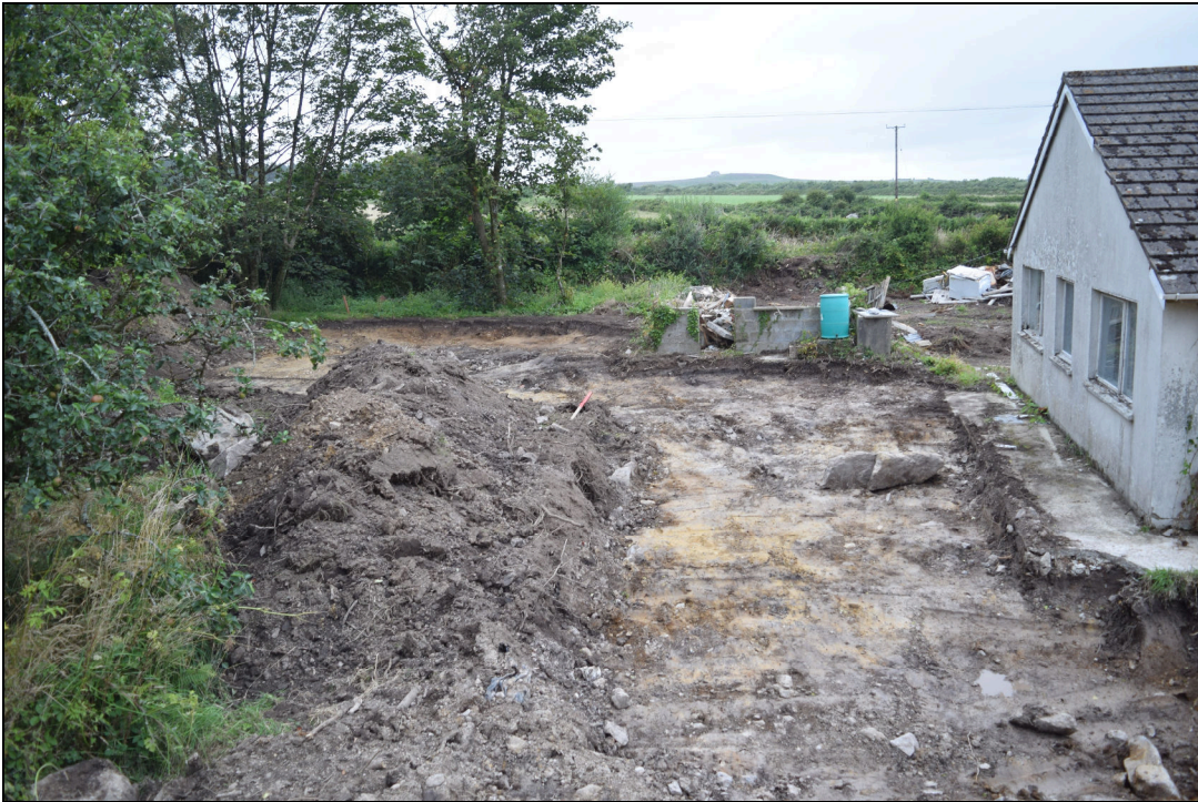
Plate 25: PCG2021_125 After removal of (001) on the western side of the current house, looking north-northeast. The surface of the subsoil undulated suggesting that the area to the south of the house was on slightly higher ground surrounded by lower ground, or small streams.
