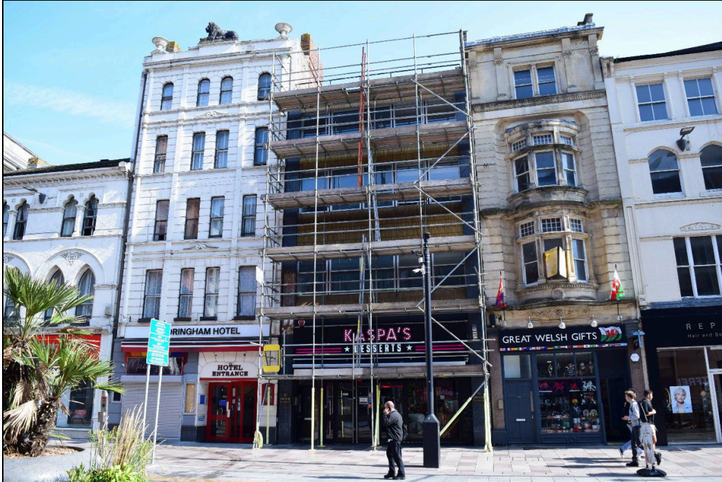
Plate 1: A view of the front of No.22 St. Mary Street, Cardiff. Scaffolding has been erected following the loss of some parts of the existing façade.
