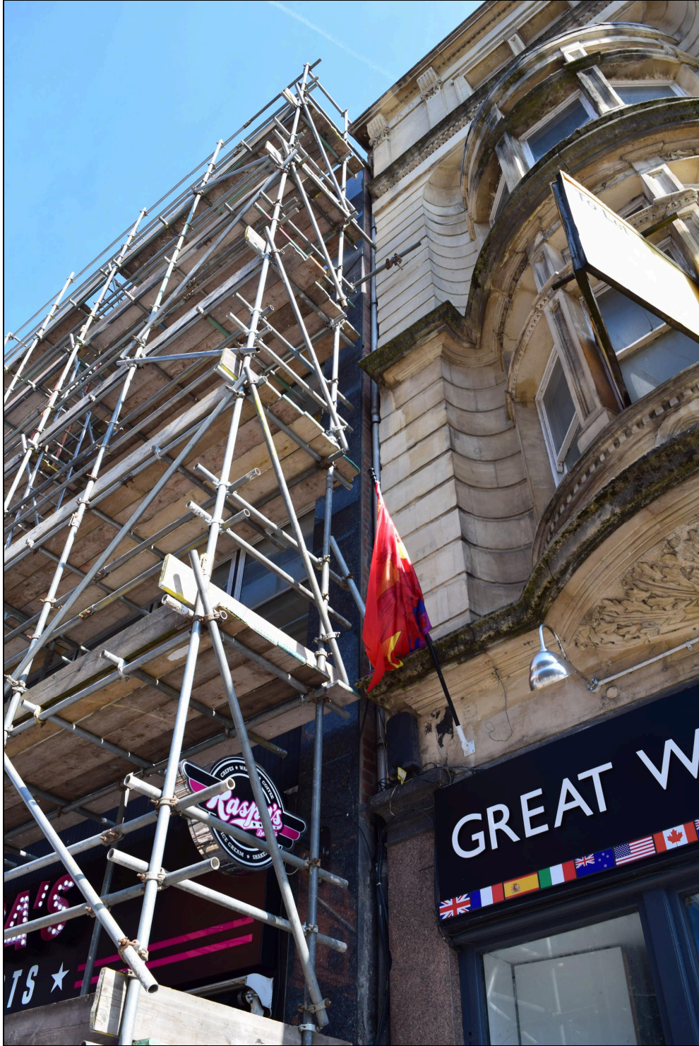
Plate 8: A view up the joint between No.22 and the property to its southern side. The marble attached to the façade has fallen away higher up the wall, revealing modern brickwork. There appears to be a narrow gap between the facades of the two buildings.
