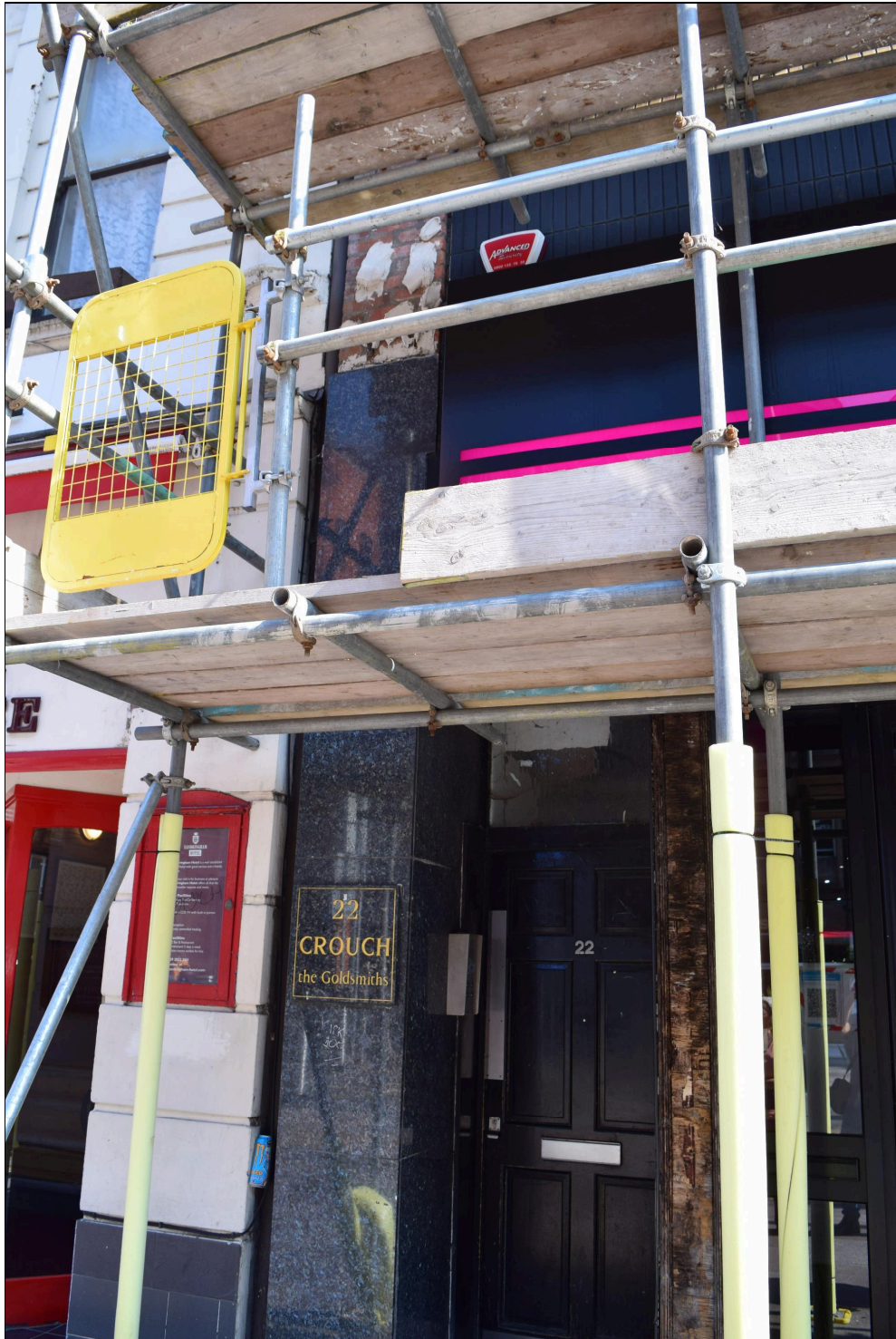
Plate 7: A view of the doorway into No.22, which still bears the name plate of Crouch the Goldsmiths. Note that the marble façade above the doorway and to the right of the door has fallen off the wall.
