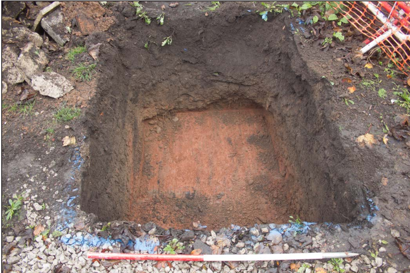
Plate 02: Plan shot of new soakaway, at Bridgewater, Church Street, Holt, Wrexham - from the north - 1.00m
