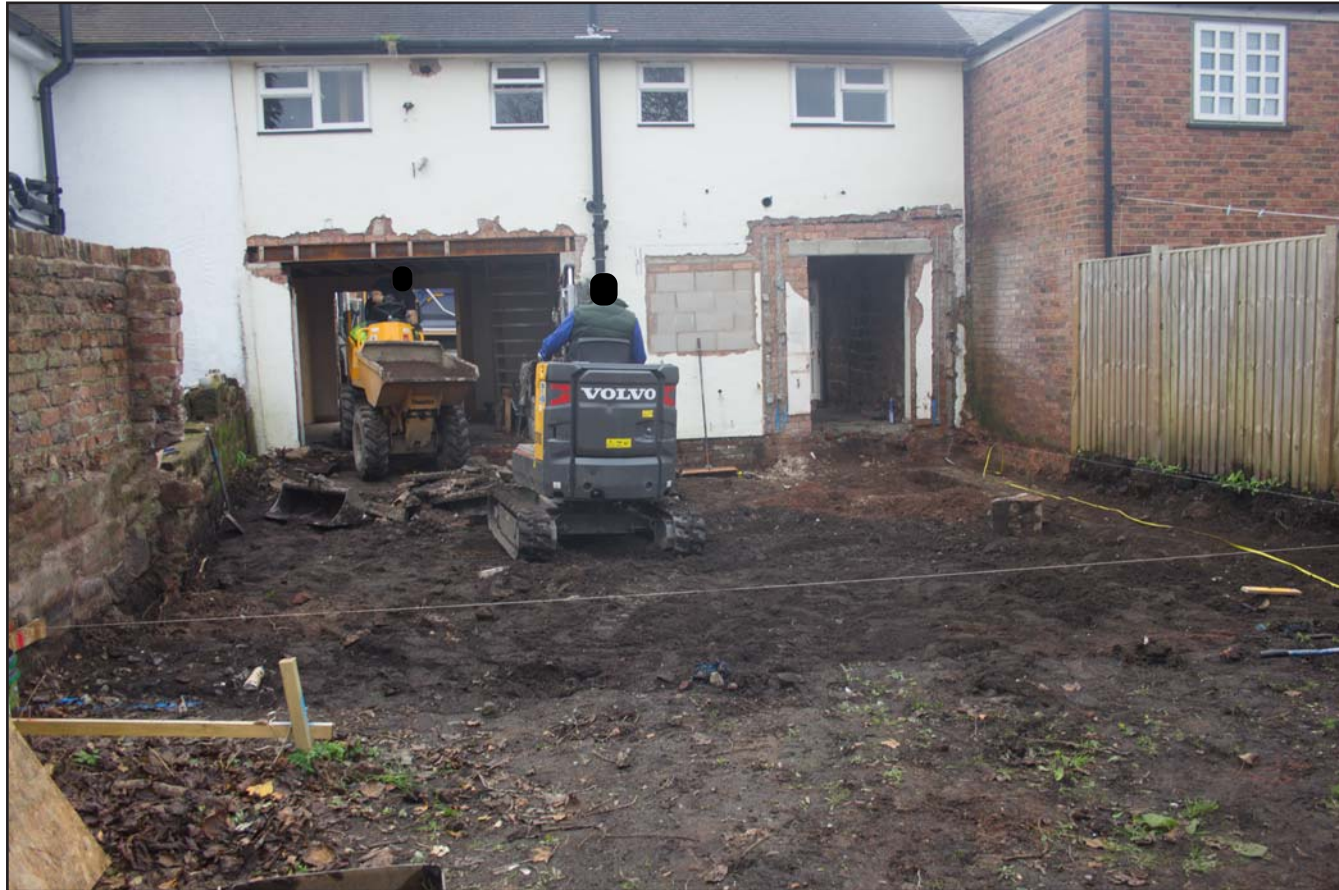
Plate 04: Working shot post topsoil strip, at Bridgewater, Church Street, Holt, Wrexham - from the west - no scale
