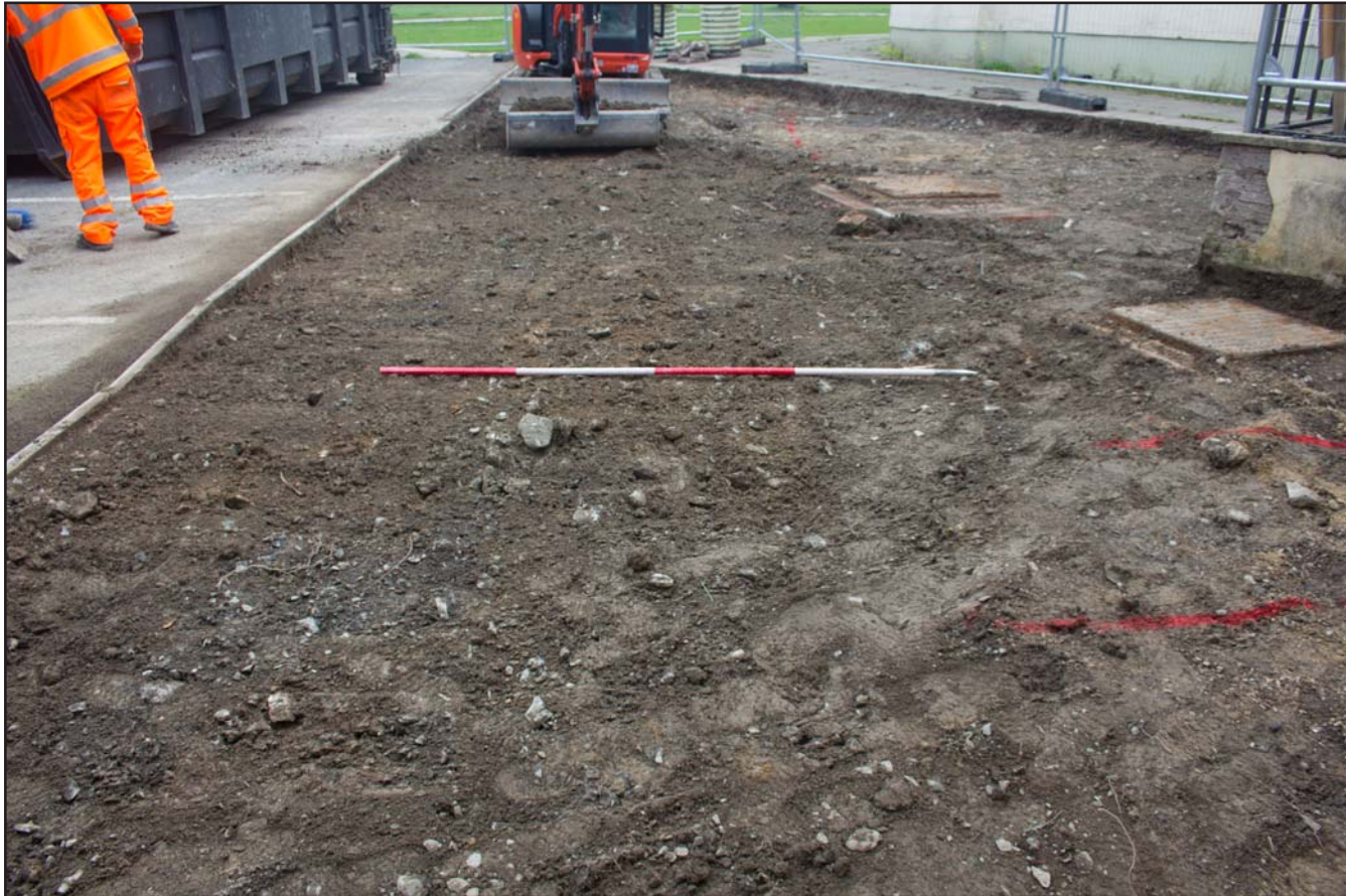
Plate 04: Topsoil Strip of development area, Y Plâs, Community Centre, Machynlleth, Powys - from the northwest - 2.00m
