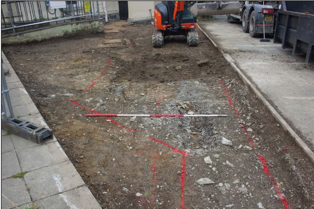
Plate 05: Topsoil Strip of development area, Y Plâs, Community Centre, Machynlleth, Powys - from the southeast - 2.00m
