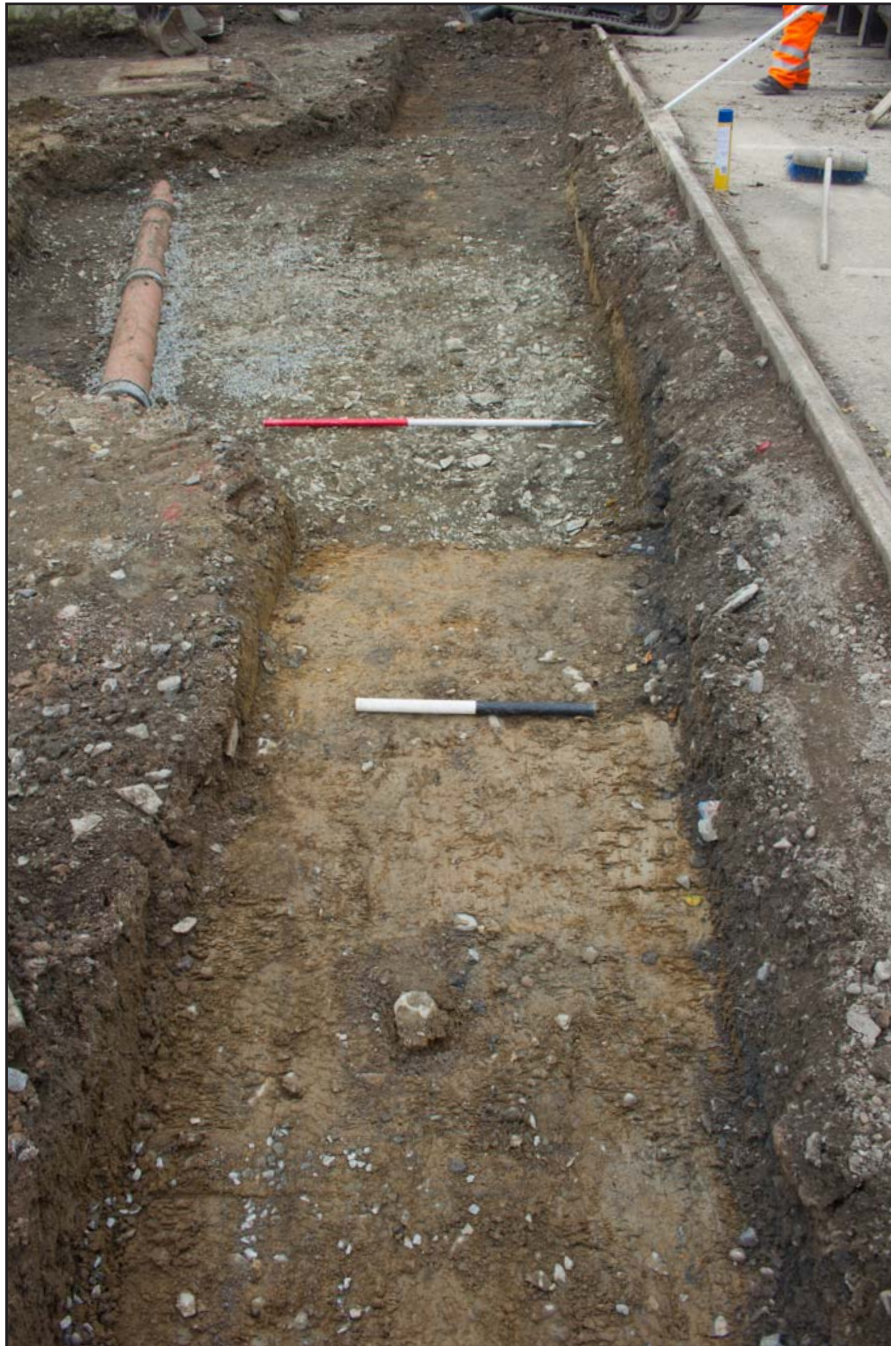
Plate 06: Wall foundation within development area, Y Plâs, Community Centre, Machynlleth, Powys - from the southeast - 1.00m & 0.50m
