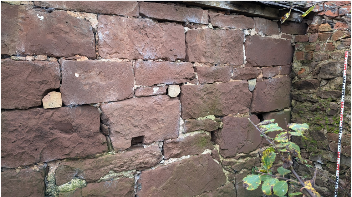
Plate 19: Eastern elevation of Room C showing breather voids
