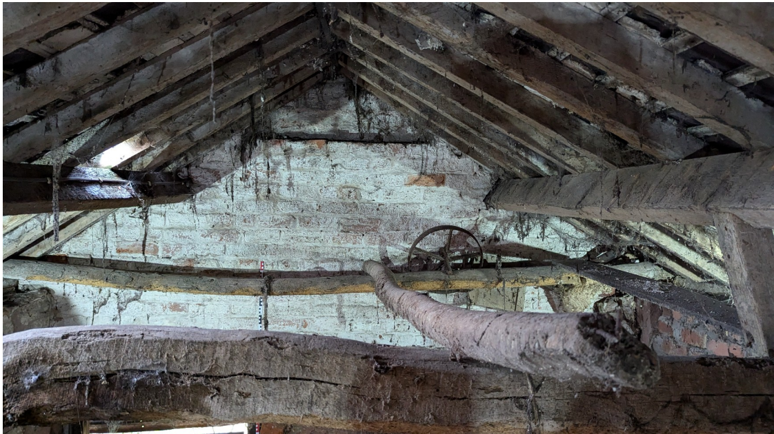
Plate 31: Room C upper section of southern wall
