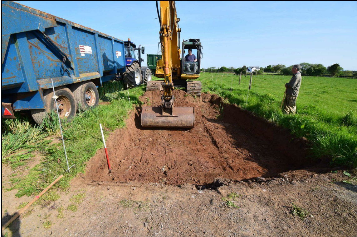
Plate 1: MYW2023_101: Excavation of a test area to test the depth of natural subsoil at the southwestern end of the new access track, at approximately ST0373075412, looking north-northwest. Here the topsoil (001) was deeper than elsewhere. A water pipe trench ran diagonally southeast to northwest across and that and the proximity to the existing farm yard may explain the depth.
