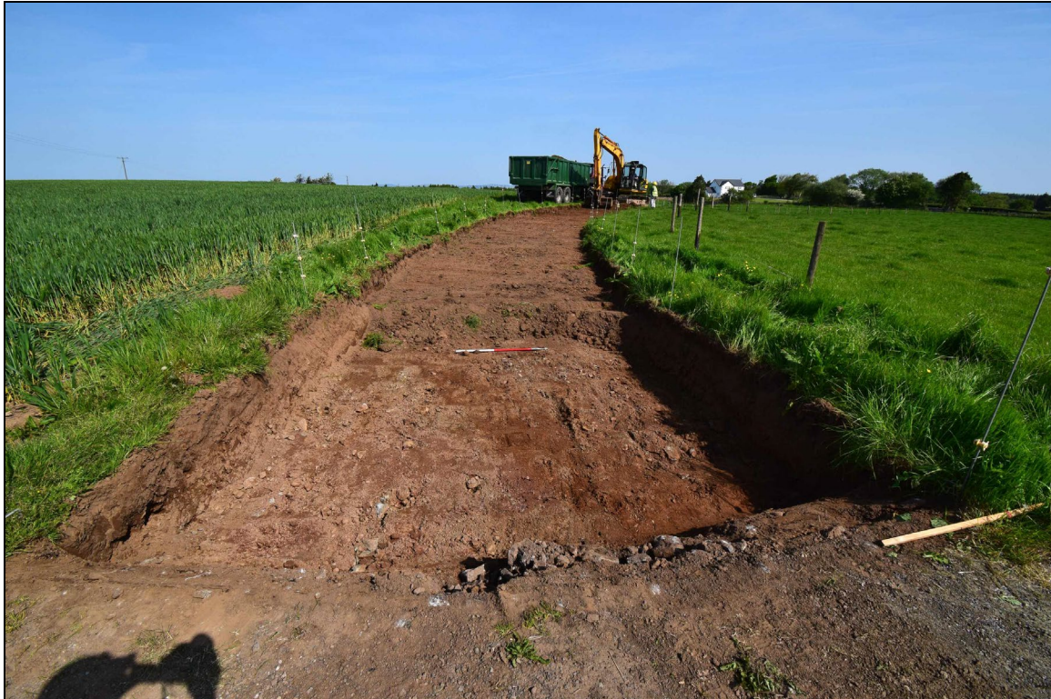
Plate 3: MYW2023_103: From ST0373075412, looking north-northwest, showing how the natural subsoil rose up after the initial 5 metres at the southwest end. The line of the water pipe can be seen in the foreground running diagonally across the base of the trench.
