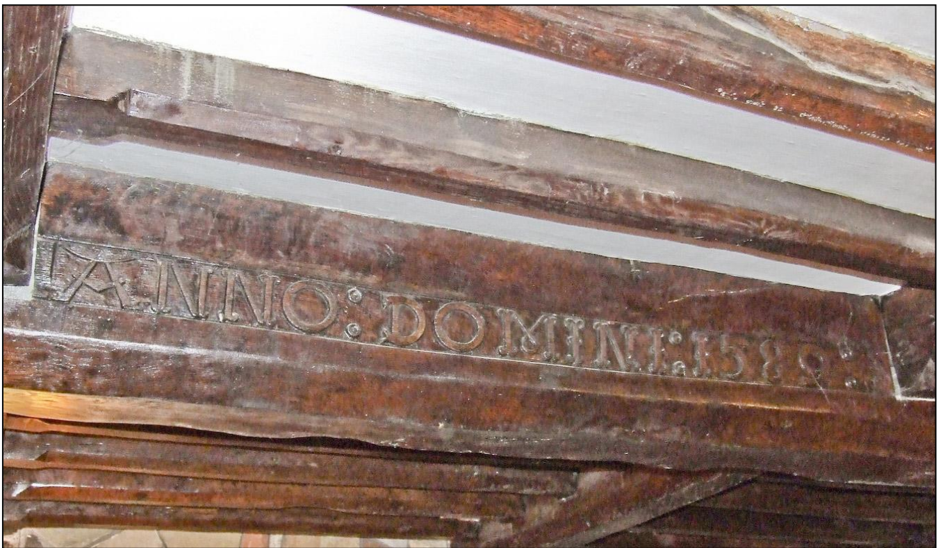
Figure 2: Carving on the main ceiling beam in the parlour, bearing the date 1589.
