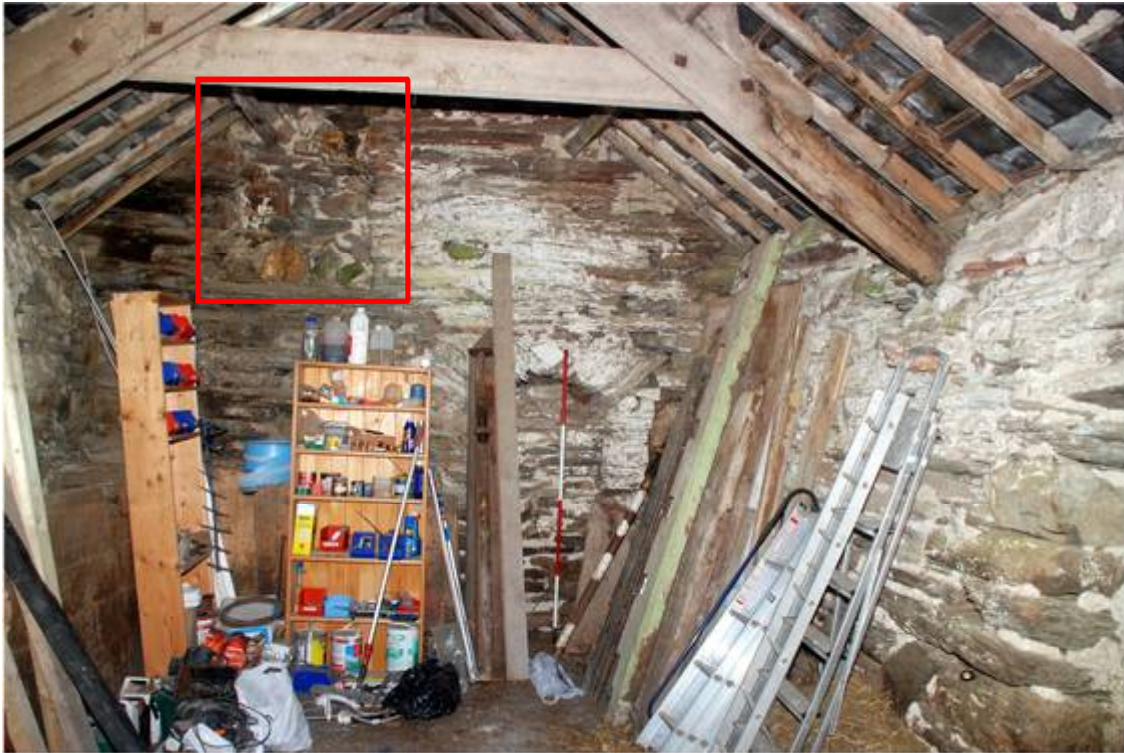
Plate 7: Blocked openings in cow house
