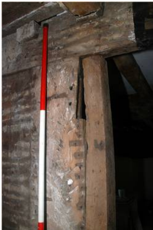
Plate 14: Detail of joint in the partition between the passageway and the main room, looking north
