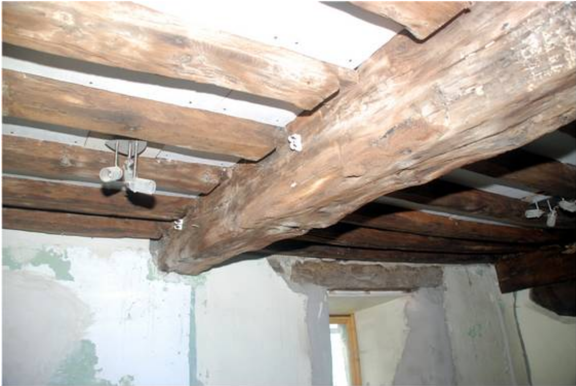
Plate 15: Detail of the ceiling beam and joists in the main room, looking north
