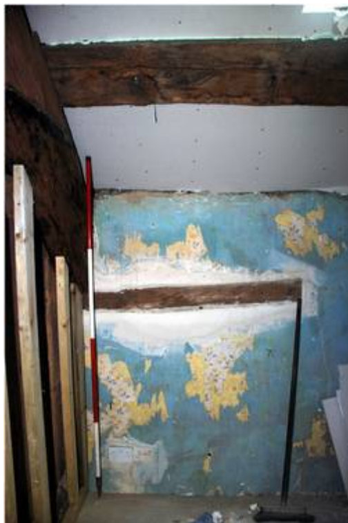
Plate 28: Wooden plate below Truss 2
