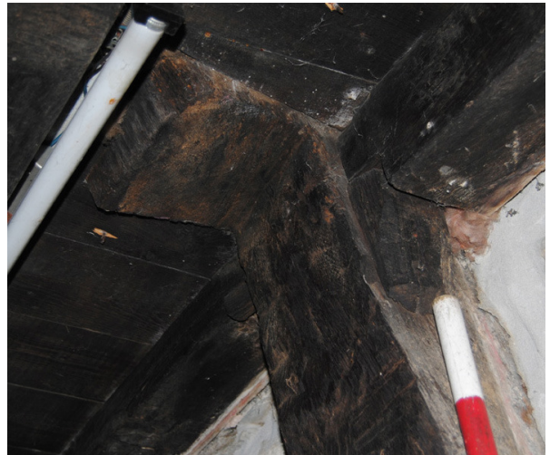
Plate 15: Western cruck blade cut back at level of inserted floor.
