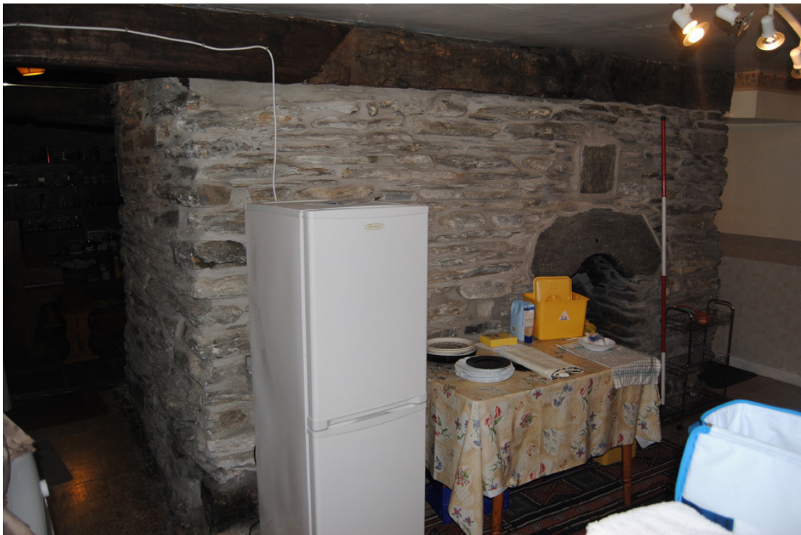
Plate 18: Rear (south) face of inserted stack; note FP (see Plate 19) and spliced head beam (Room [GF03]).
