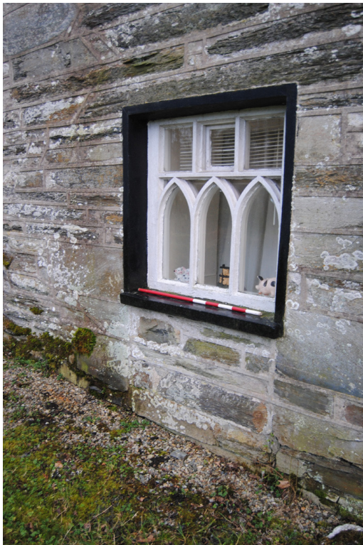
Plate 28: Eastern window with SJs beneath cill.
