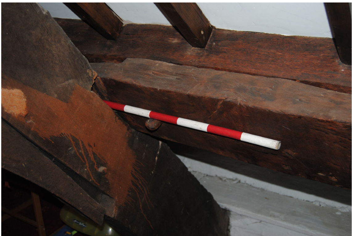
Plate 24: Surviving section of primary lower purlin to SE quadrant of roof structure.
