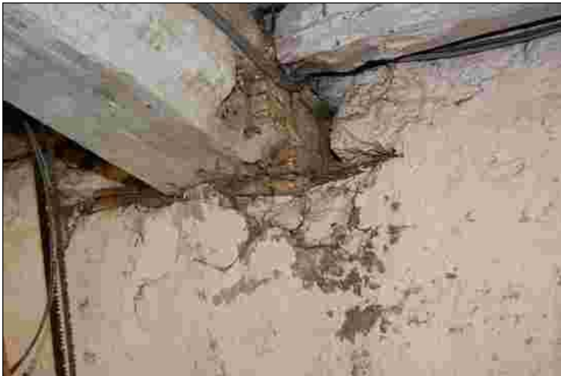
Plate 10: The eastern end of the southern ceiling beam in the southern ground floor room
