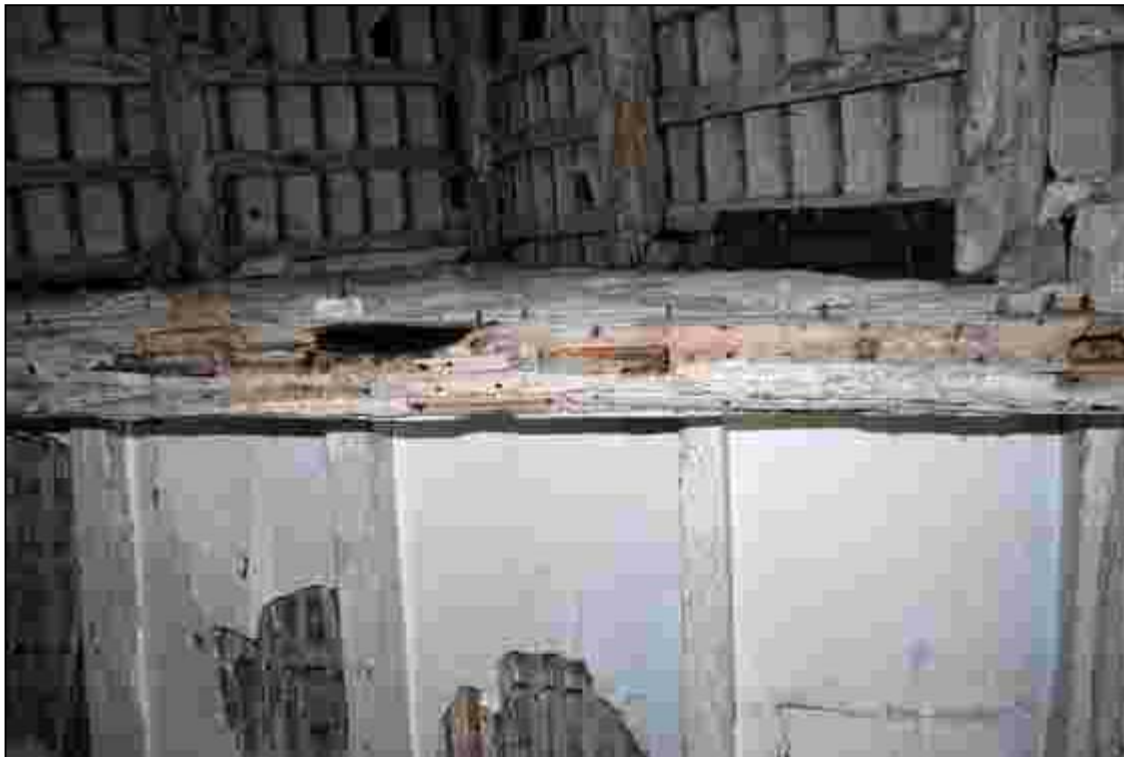
Plate 27: Mortice holes below Truss 2
