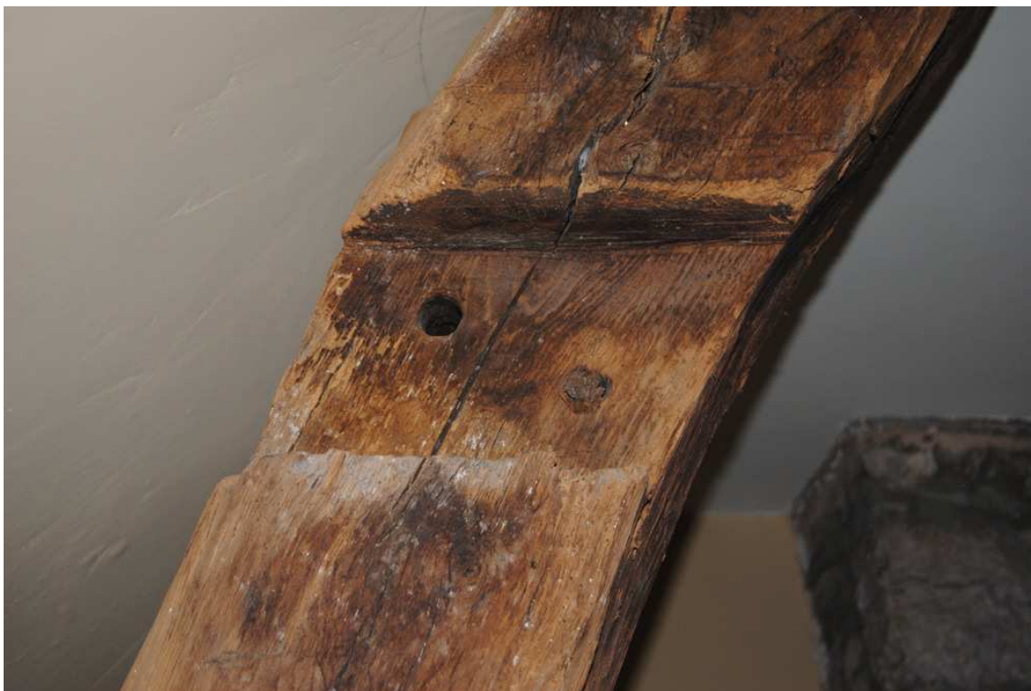
Plate 11: Cruck [T3] (E), redundant lap-joint for tie.
