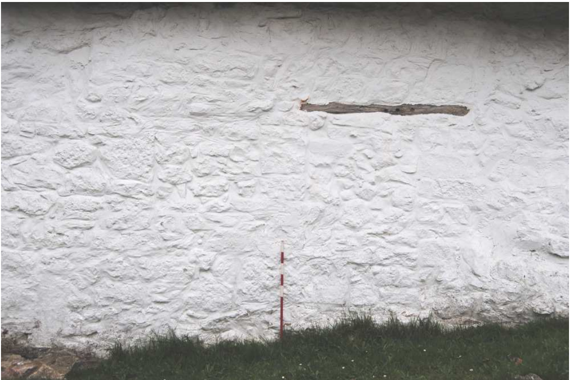
Plate 5: Blocked window (left) and doorway (right with lintel) at north end of west elevation.
