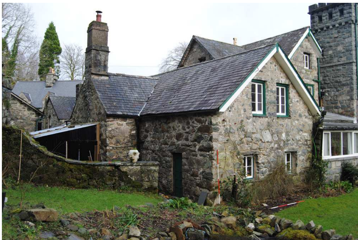
Plate 4: 'Old Hall' range from south-west with gabled lateral stack projection to left.
