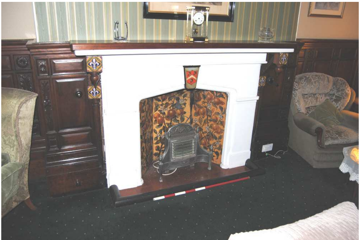
Plate 23: 'Arthro' range, [GF01] inserted fireplace with painted slate panels.
