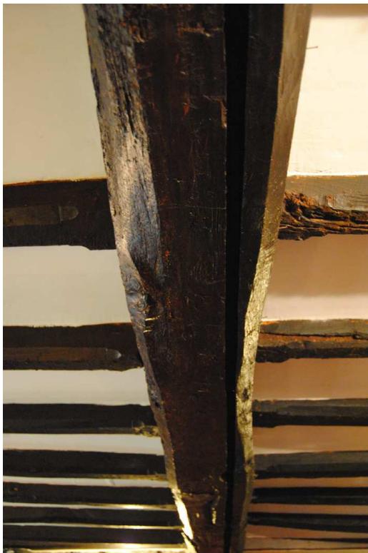
Plate 9: [GF01]: groove to soffit of beam C.
