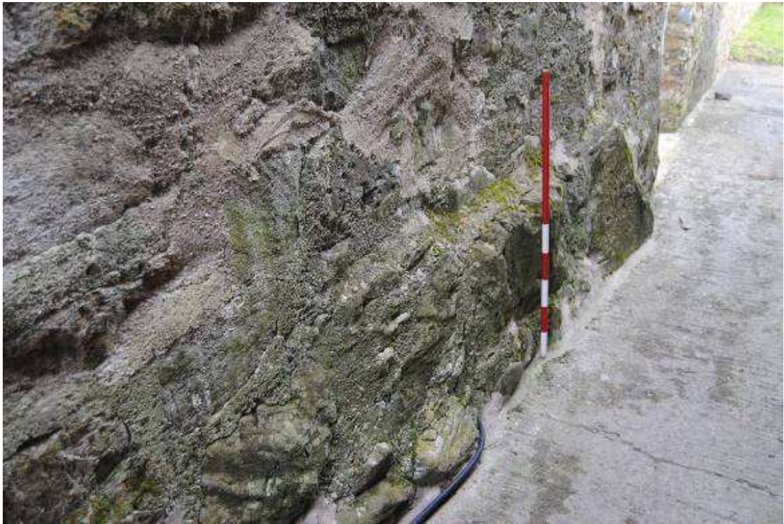
Plate 7: Offset boulder footings to south elevation (also present to east and north elevations and evidenced to west).
