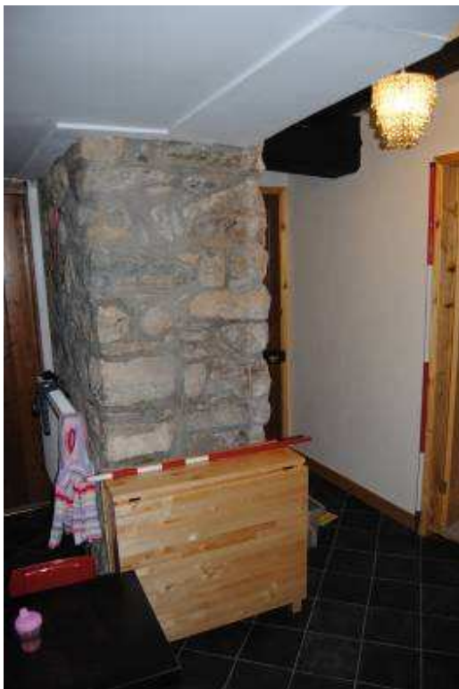
Plate 13: [GF04] truncated west wall.
