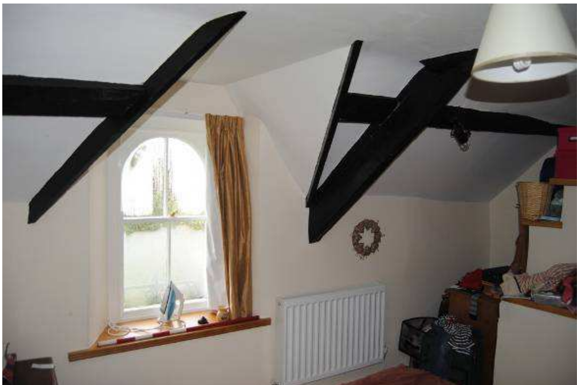
Plate 23: Principal rafter of Truss T1 within Room [1F02] with C19th dormer to left.
