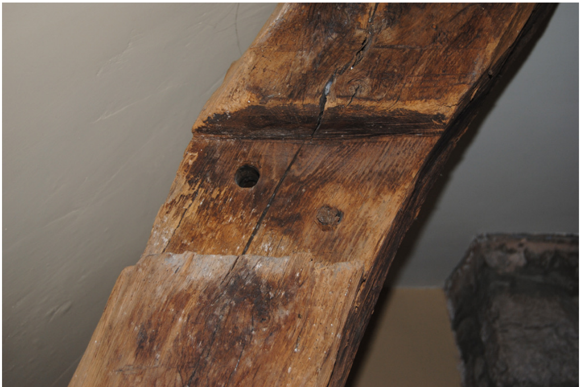
Plate 11: Cruck [T3] (E), redundant lap-joint for tie.
