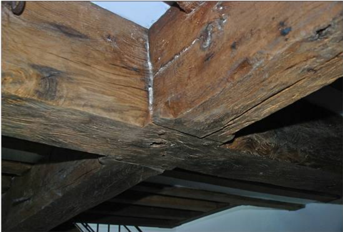
Plate 13: Detail of chamfers and stop at intersection between the longitudinal and lateral beams.
