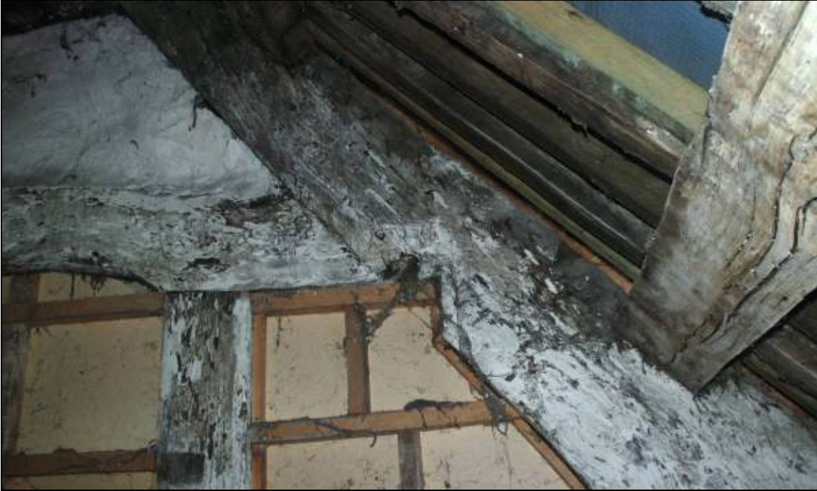
Plate 8: Cut out on northern principal rafter, Truss 1, looking west.
