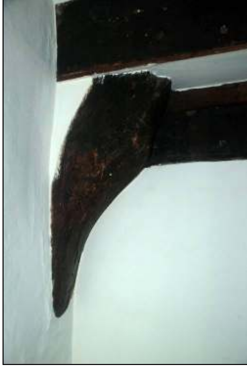
Plate 3: Base of the northern cruck frame, east side of the house, looking north.
