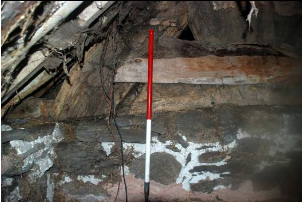
Plate 15: Half lap joint between the principal rafter and tie beam on the barn gable end truss looking SE
