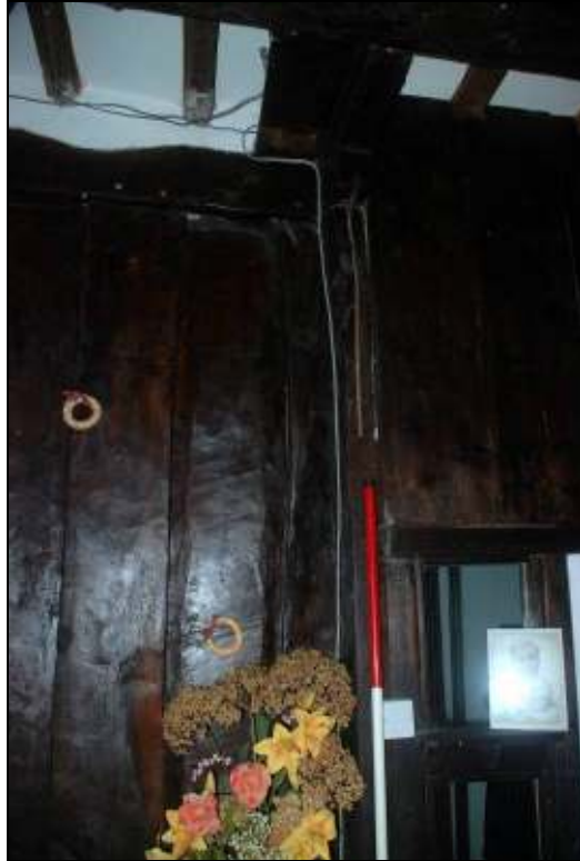
Plate 19: Position of a partition in the western ground floor room, South Wing, looking south
