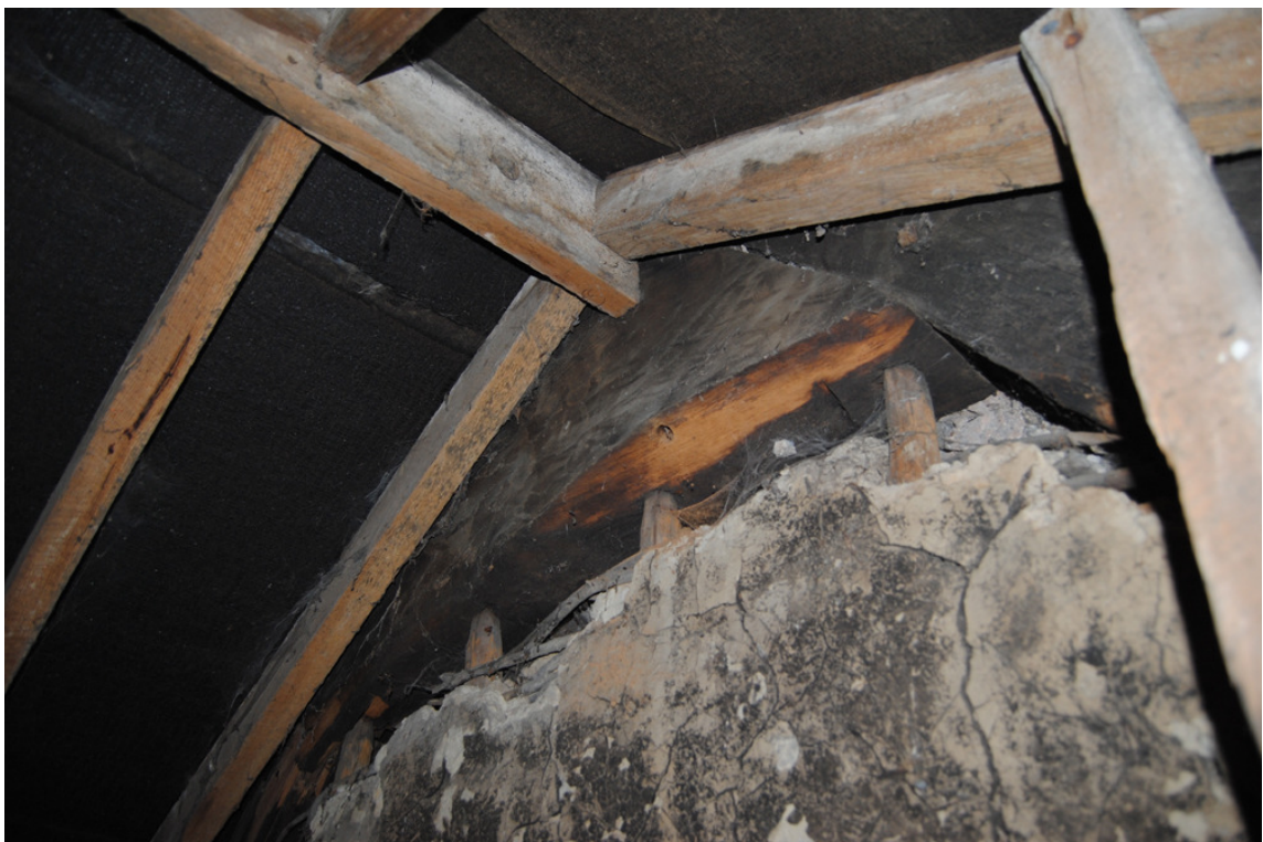
Plate 27: Apex detail of Cruck [T4] as observed above room [1F05], NB: wattle and daub infill (with smoke blackening) applied to staves below yoke. Yoke core [deni7] dated to winter 1488/89.
