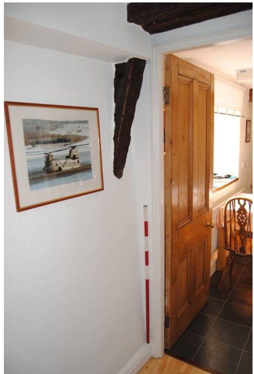
Plate 11: Lower cruck blade of [T2] visible at doorway between [GF01] and [GF02].
