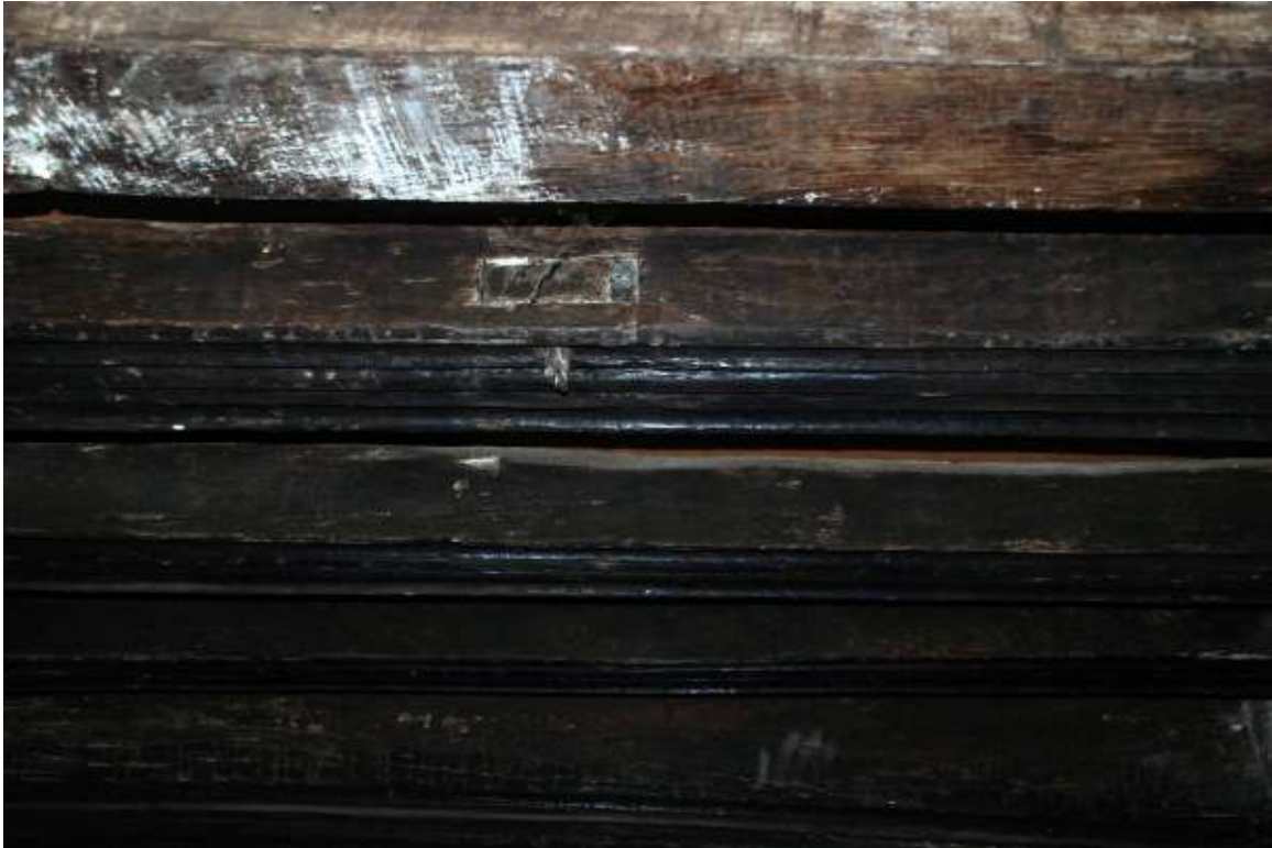
Plate 46: Mortice hole for a lost trimmer in ground floor SW room, looking NW
