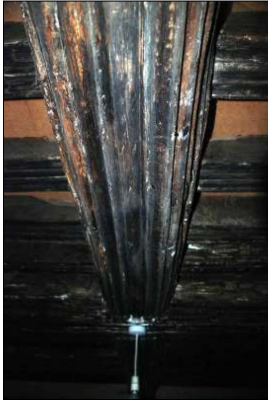
Plate 43: Detail of moulding on ceiling beam in SW ground floor room, looking NW
