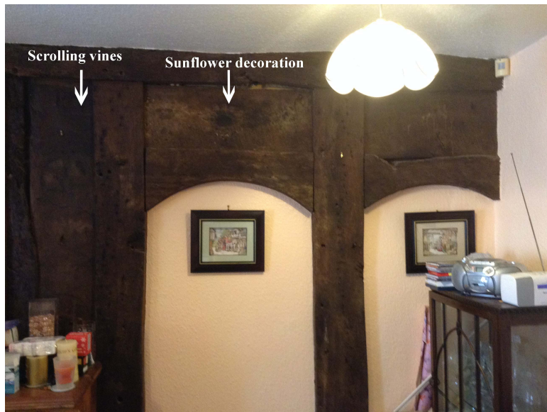
The post and panel wall showing the original doorways connecting the parlour and service area to the main hall, and the painted decoration.
